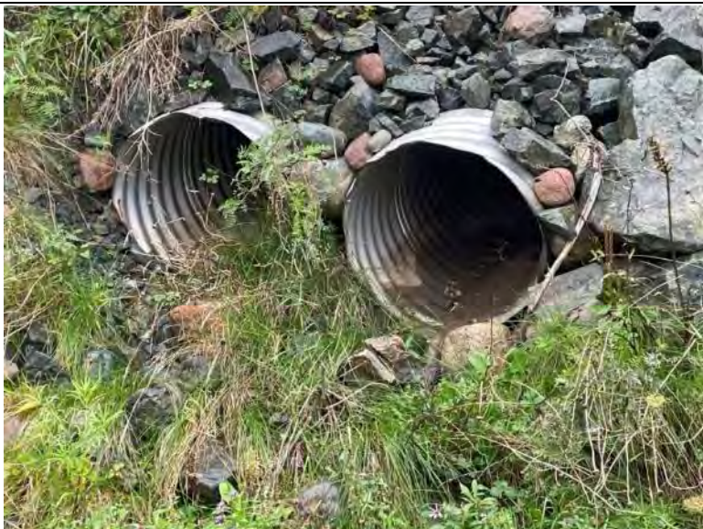
Photo 49 Double Culverts at WCS-409 (Profile 108039). Approximately 1050 m From the Confluence With Turning Basin.
