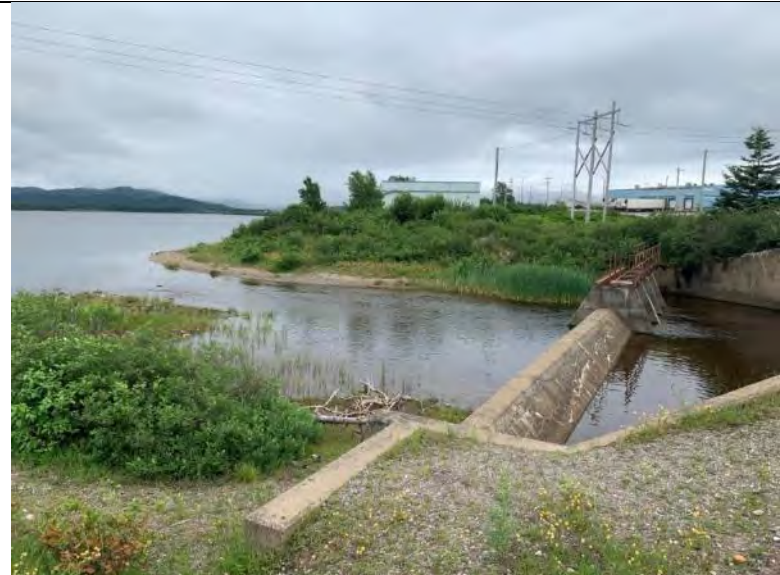
Photo 68 Remnant Concrete Dam at the Outlet of Noels Pond, WCS-410 (Profile 96345), Facing Upstream Approximately 4000 m From the Confluence with the Ocean.
