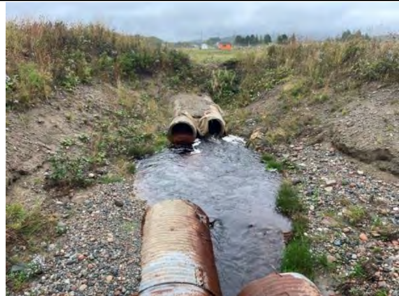
Photo 34 Double Culverts at WCS-407 Upstream of the Road Crossings, Facing Upstream Towards the Plant Site.
