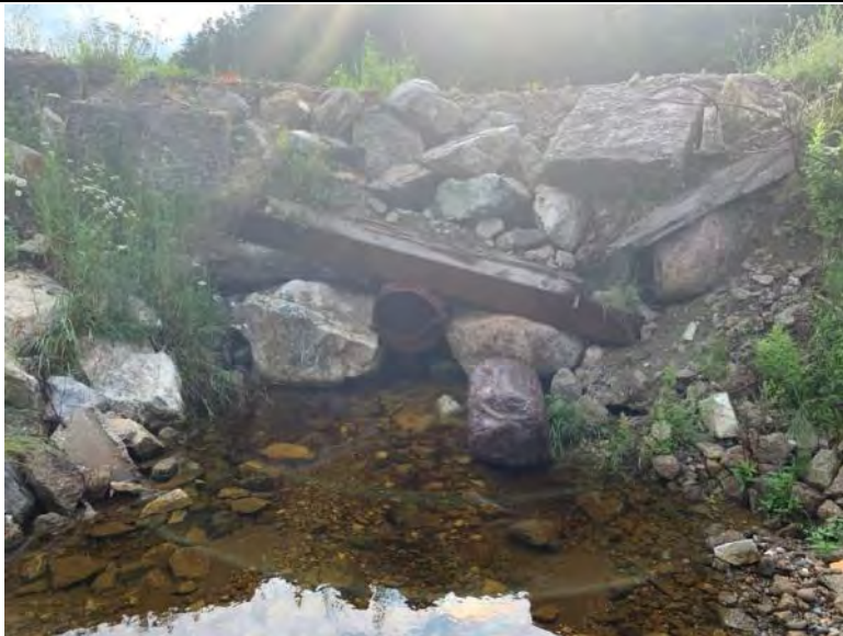
Photo 37 Steel Culvert at WCS-409 (Profile 96348) Approximately 75 m From the Confluence With Turning Basin.
