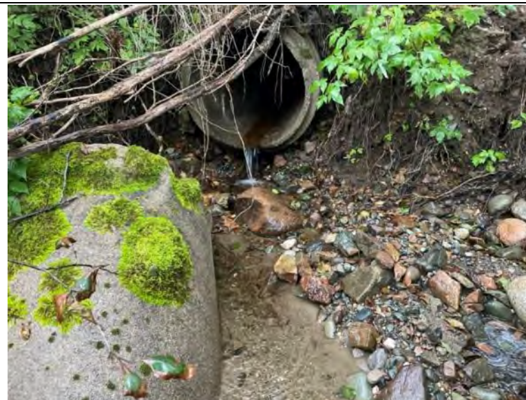
Photo 46 Concrete Culvert at WCS-409 (Profile 108037). Approximately 965 m From the Confluence With Turning Basin.
