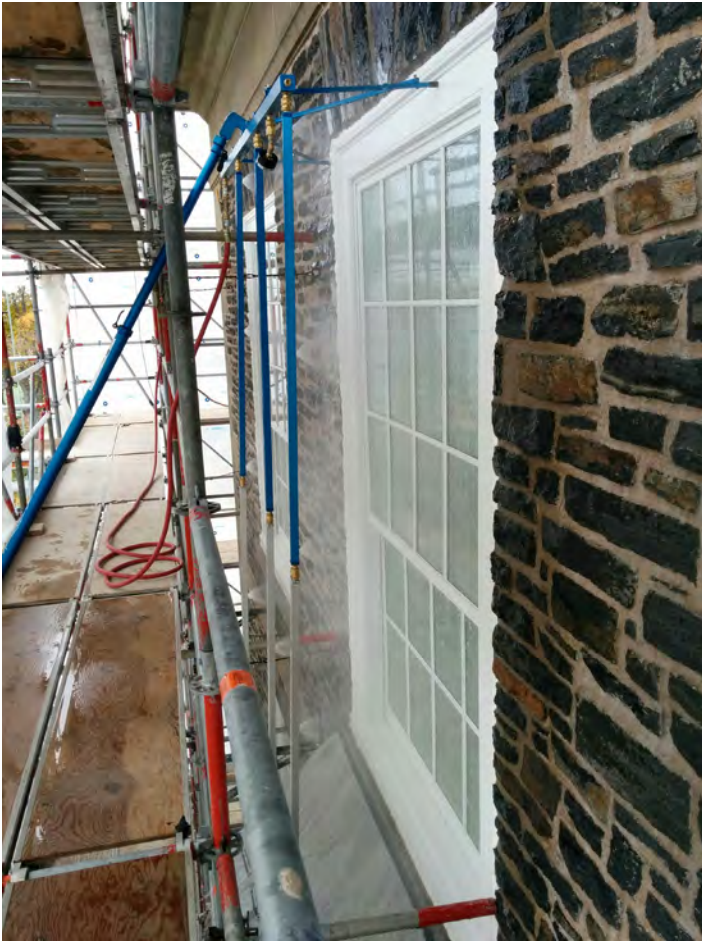
This image shows a window installation being tested for water infiltration. The building owner wanted to verify that the window and the installation met the expected performance specification.
