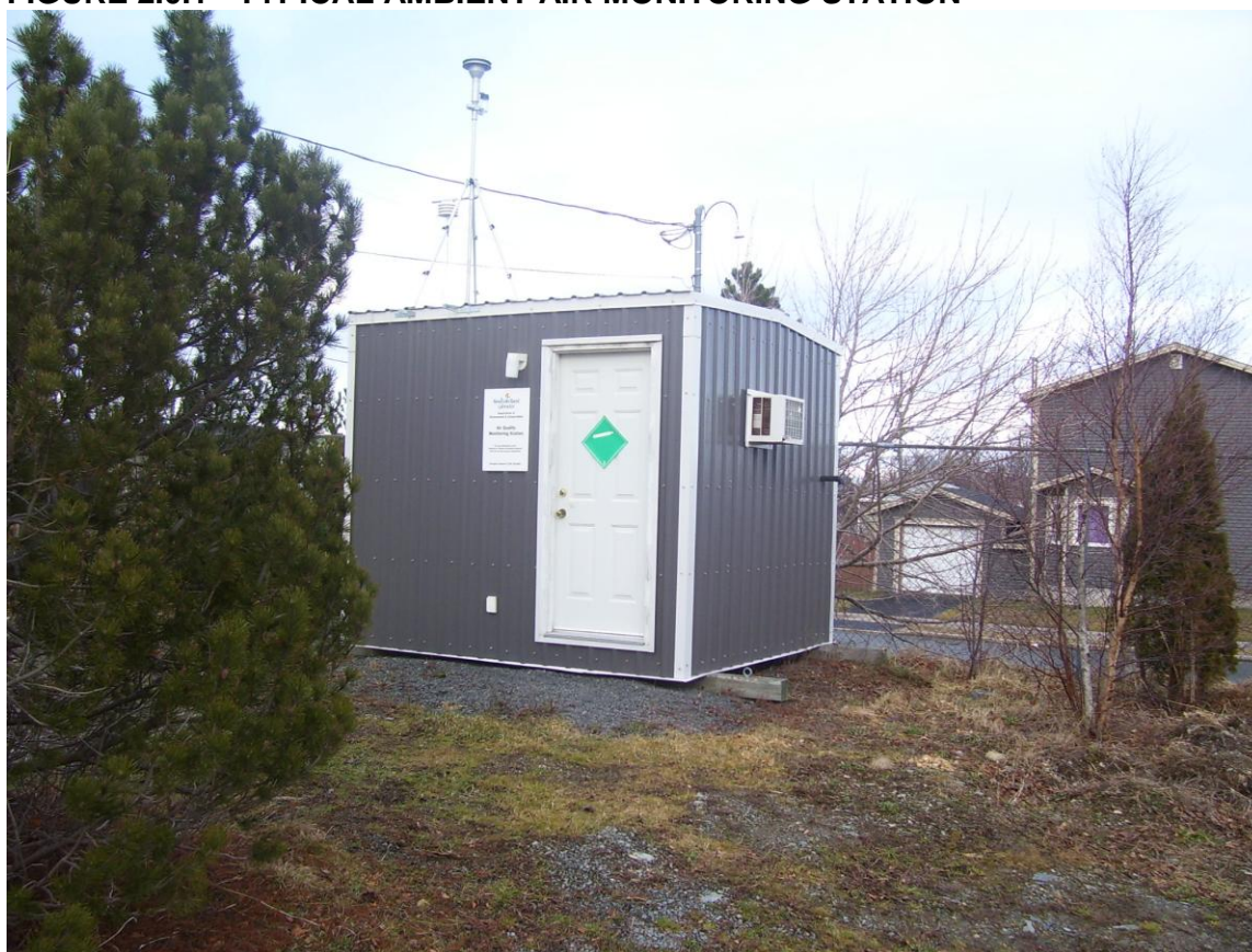
FIGURE 2.0.1 - TYPICAL AMBIENT AIR MONITORING STATION
