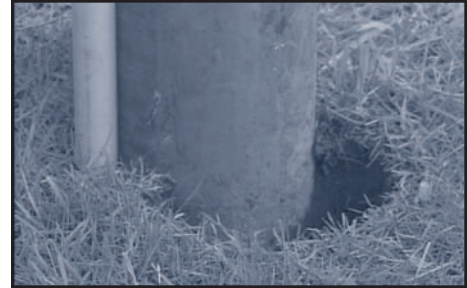
Faulty annular seal.
