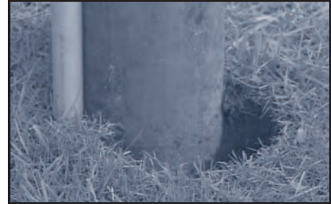
Faulty annular seal.
