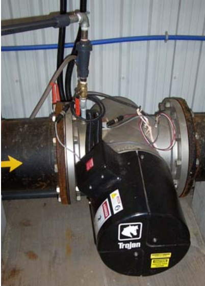
Figure 38: UV treatment system from Pasadena WTP
