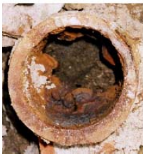
Figure 6: Corroded CI pipe
