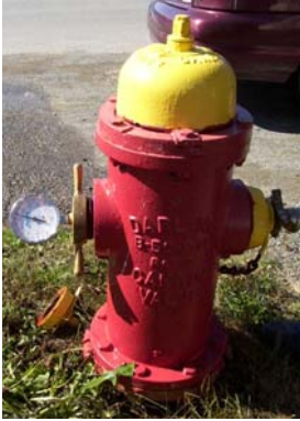
Figure 54: Brighton system pressure reading from fire hydrant
