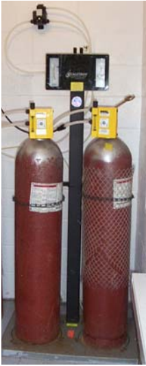
Figure 139: Hawke's Bay chlorination system
