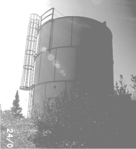
Figure 50: Brighton water storage tank
