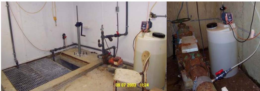
Figure 94: Ferryland chlorination system at the intake (left) and at the flow meter (right)
