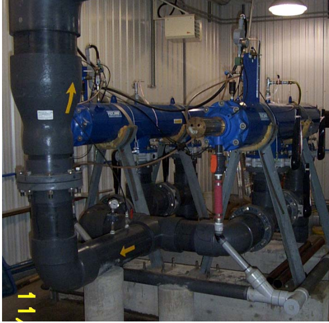
Figure 41: Pre-filtration system at Pasadena WTP
