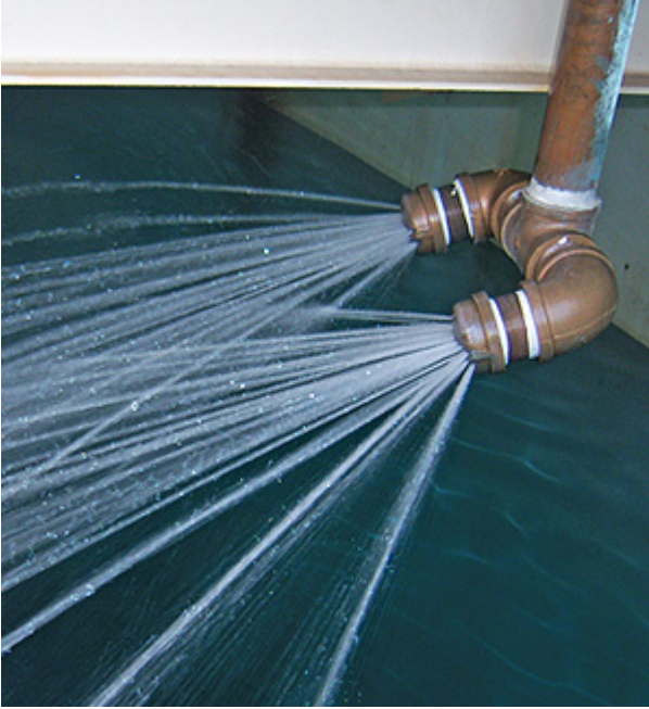
Figure 34: Aeration system in water storage tank
