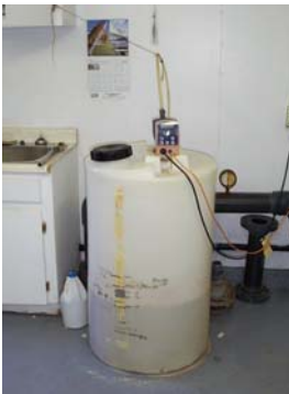
Figure 52: Brighton hypochlorination system
