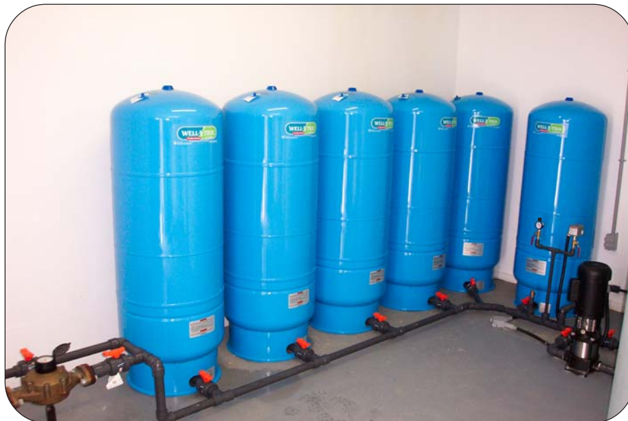
This is the pump system for a well in Chance Cove. From right to left are the booster pump, six pressure tanks and a flow meter.
