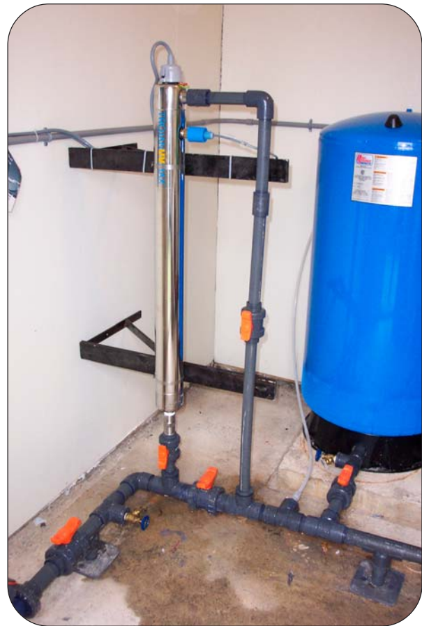
An ultraviolet (UV) disinfection system on the Town of Colliers #5 Well - Whalens Well. The UV system is the vertical silver tube on the left.
