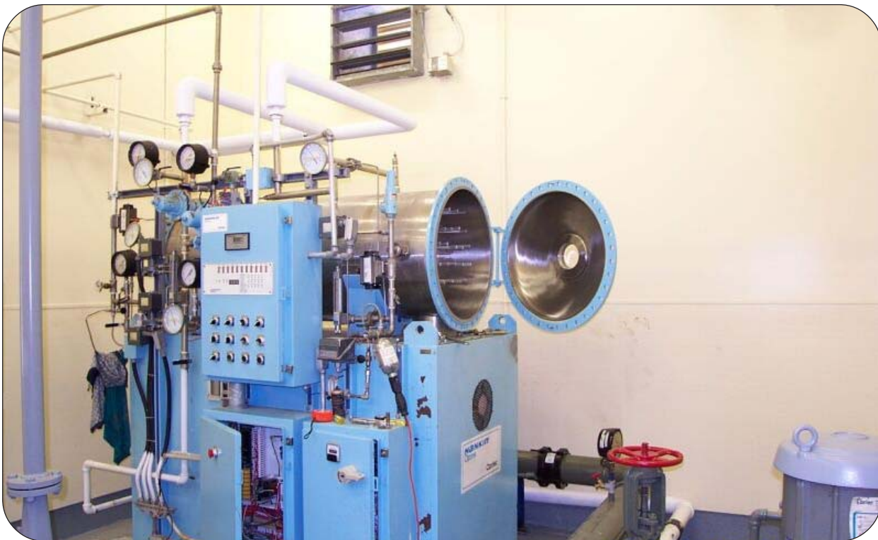
Ozone generator at the water treatment plant in the Town of Placentia (Dunville)
