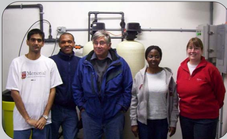
Groundwater Resources Manager and project supervisor Keith Guzzwell (centre) with the four graduate engineering students (left to right: Jayakumar Balakrishnan, Eleghasim Ndukauba Michael, Abiodun Abati and Trish Johnson). The picture was taken in front the first arsenic removal equipment to be installed in the province, at the Angus Brace public water supply well in Chance Cove.
