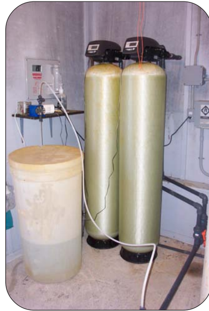
Arsenic filter unit (cylinders in center of picture) on Southside Well in Harbour Grace has been successful in removing arsenic from source water so that drinking water is now in compliance with GCDWQ.
