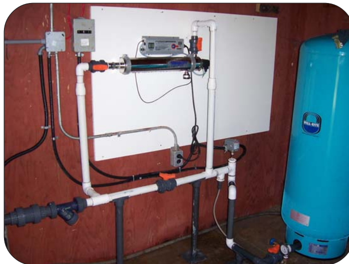
UV disinfection system (silver tube in center of picture) in the western Newfoundland town of Bay St. George South.
