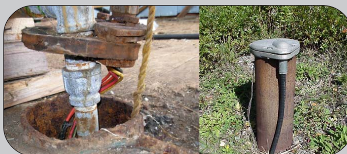
Above: A poorly constructed, improperly sealed floor-level well (left), and a properly constructed well (right).
