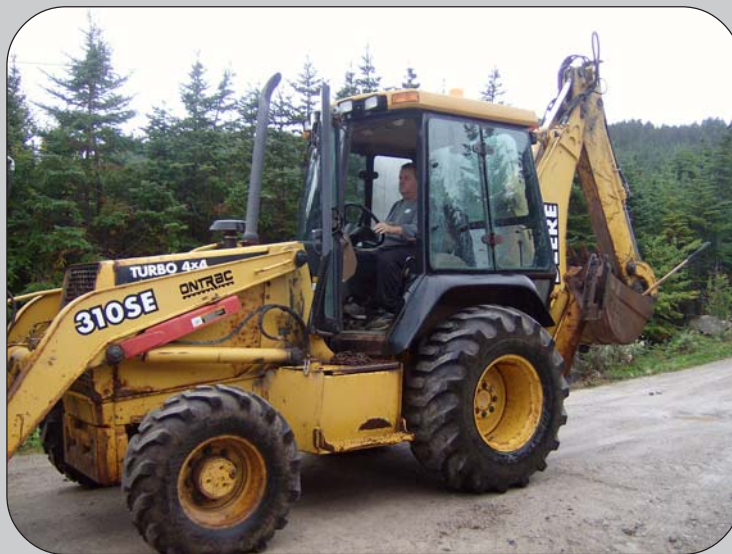
Above: Wayne Rouzes of Cape St. George operates an excavator to fix leaks in the town's water-distribution system.
