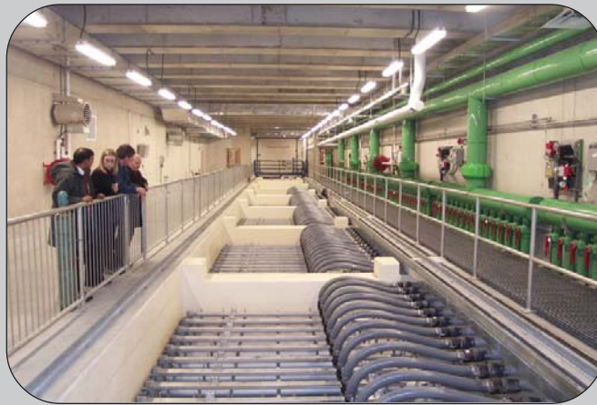
Above: City of St. John's and ENVC staff overlook the Windsor Lake Water Treatment Plant, shown are Haseen Khan, Lynnann Stapleton, Martin Goebel, Art Cheeseman.
