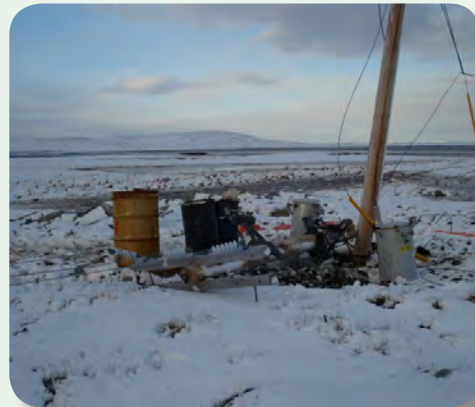
Downed and leaking transformers
