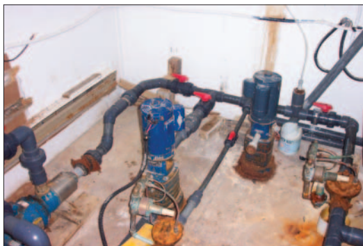
Nicky's Nose Cove pump house, Jackson's Cove-Langdon's Cove-Silverdale
