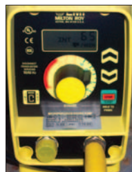
Chlorine metering pump
