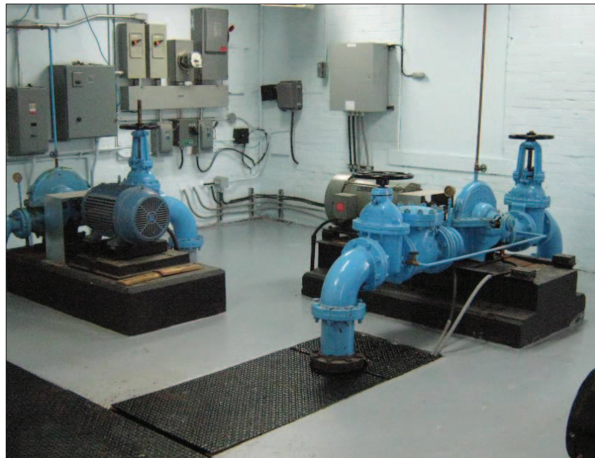
Drinking water distribution piping, Exploits Regional Water Treatment Facility
