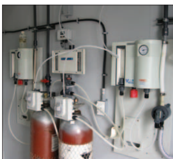
Gas chlorination, Ramea water treatment plant
