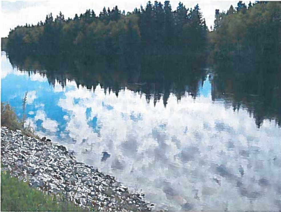
Figure 7: Repair of upstream face of West Bank Dyke opposite of natural stream in the vicinity of Weirs 7 & 8
