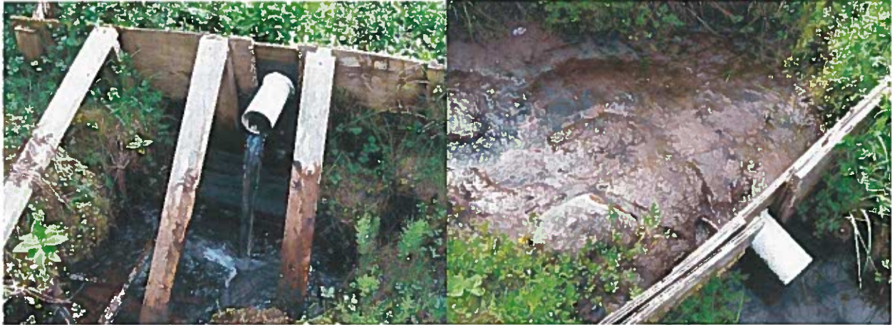
Figure 6. Weir 2 (left) and Weir 4 with accumulated sediment (right) monitoring seepage from the toe of the West Bank Dyke
