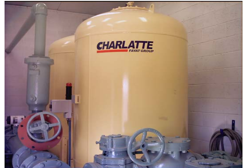
CITY OF FAIRVIEW OREGON. 2x528 GALLON WASTE WATER BLADDER SURGE VESSELS.
