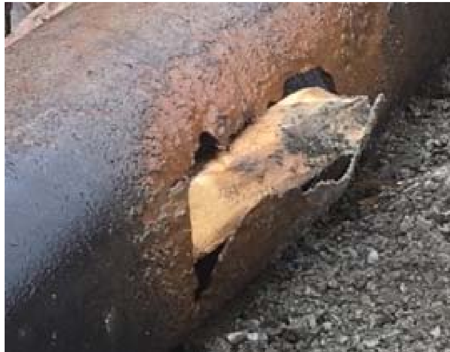
Close-up of ruptured main and piece of timber
