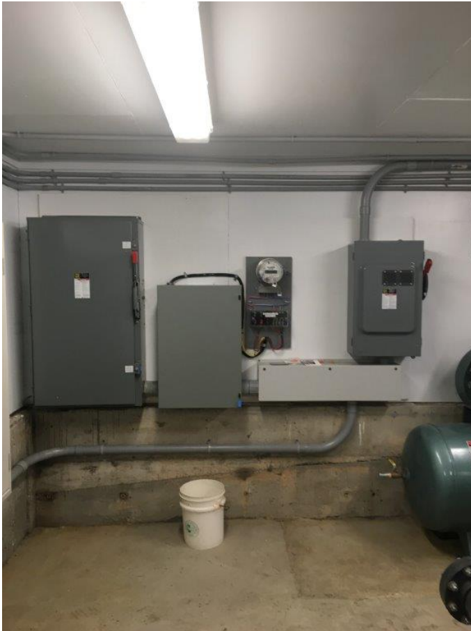
Incoming Power, Disconnects, Meter Base, etc.
