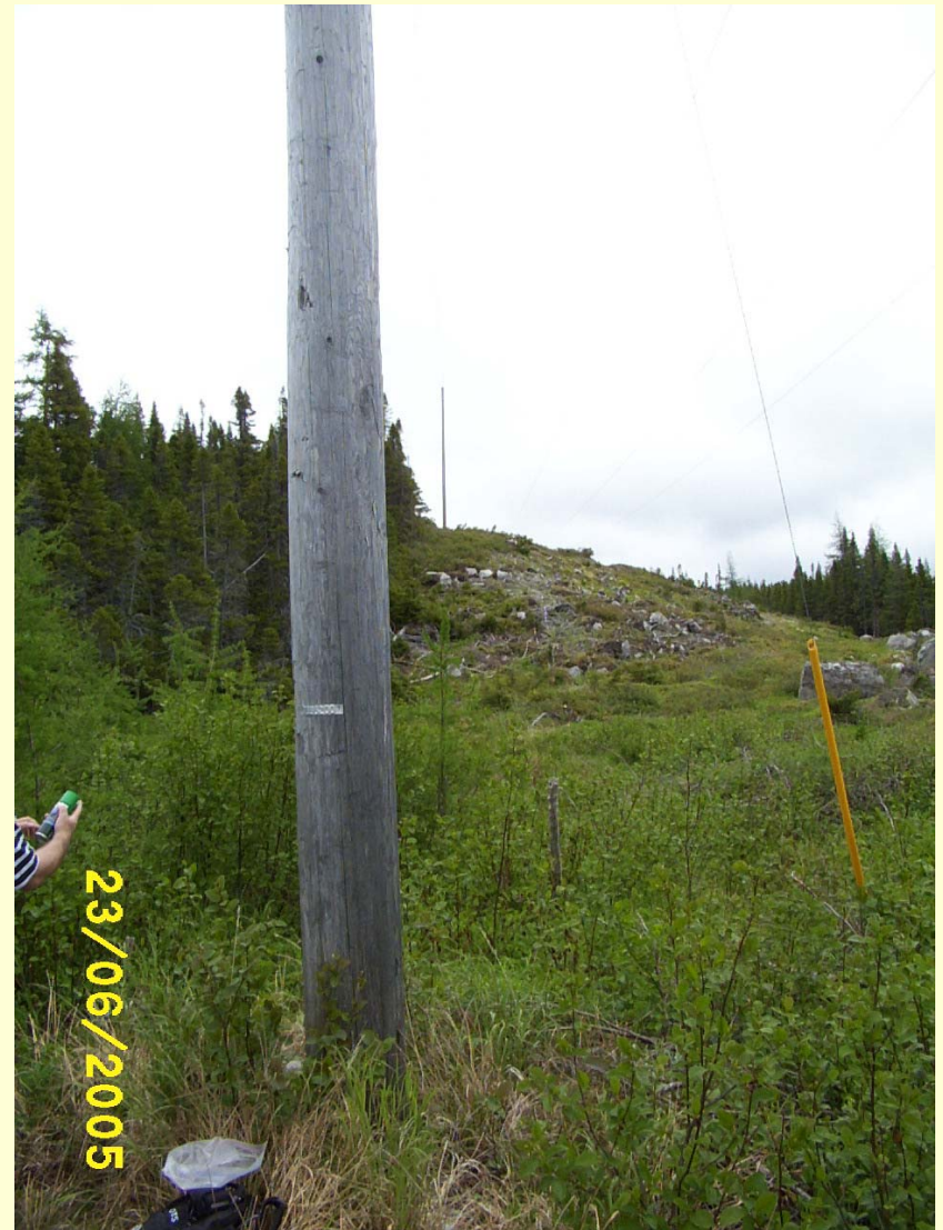
Untreated utility pole used in Steady Brook PWSA
