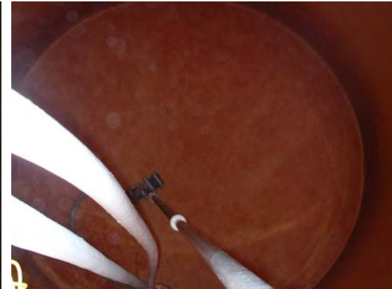
Coagulation and Settling Unit
