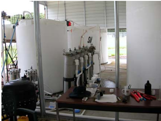
Softening and Filtration Units
