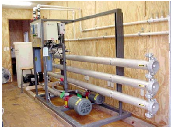
Reverse Osmosis Unit
