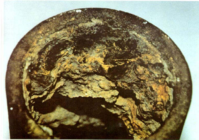
Fig. 5.5. Tuberculation in a cast iron pipe.
