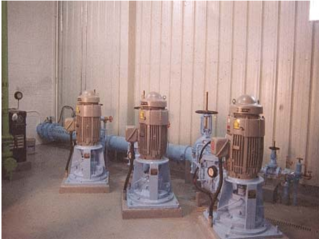
Vertical Turbine Pumps – Goosebay WTP
