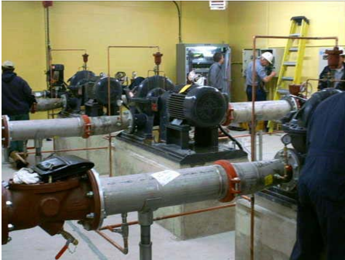
Water Booster System - Ottawa
