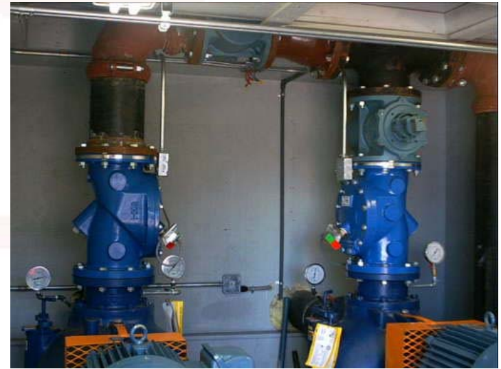
Town of Windsor Pumping Station
