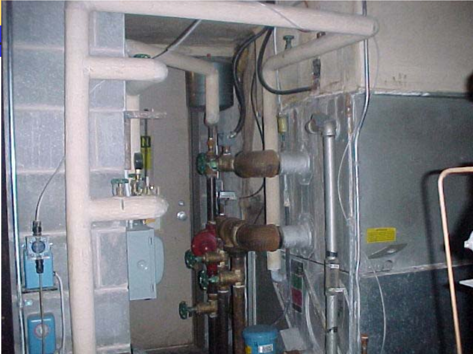
Make-up line for cooling tower and glycol loop
