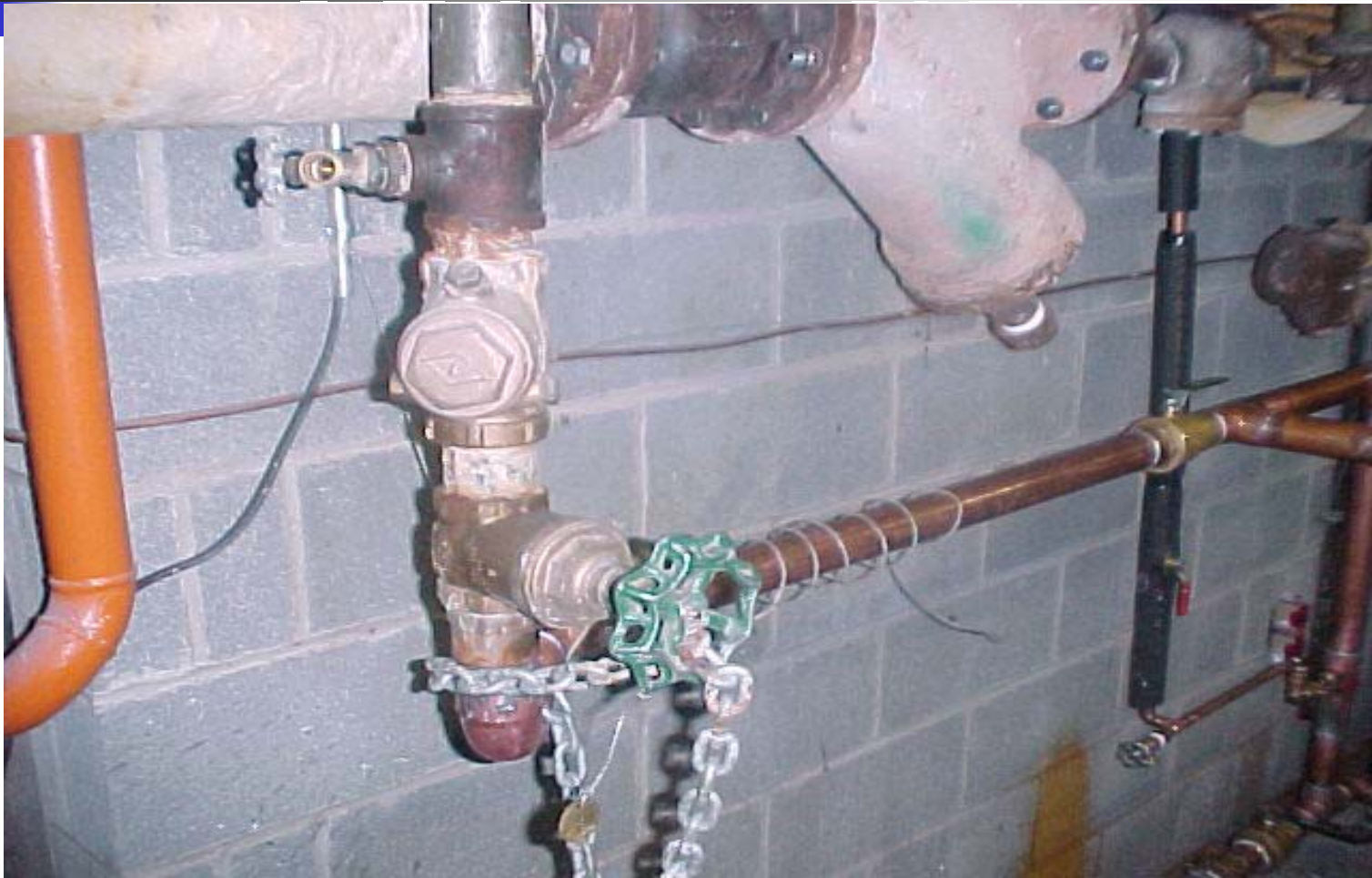
Standpipe for Fire Hose Cabinets
