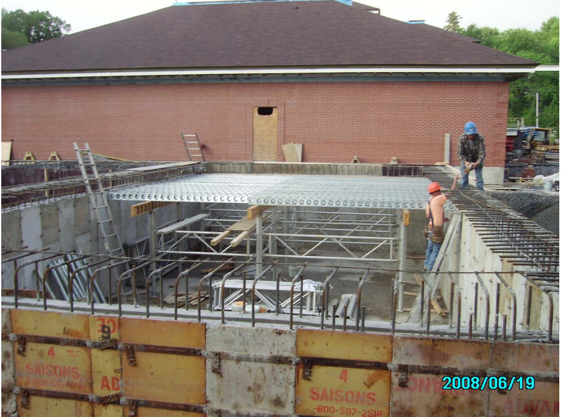
Reclaim Tank at North Building Exterior
