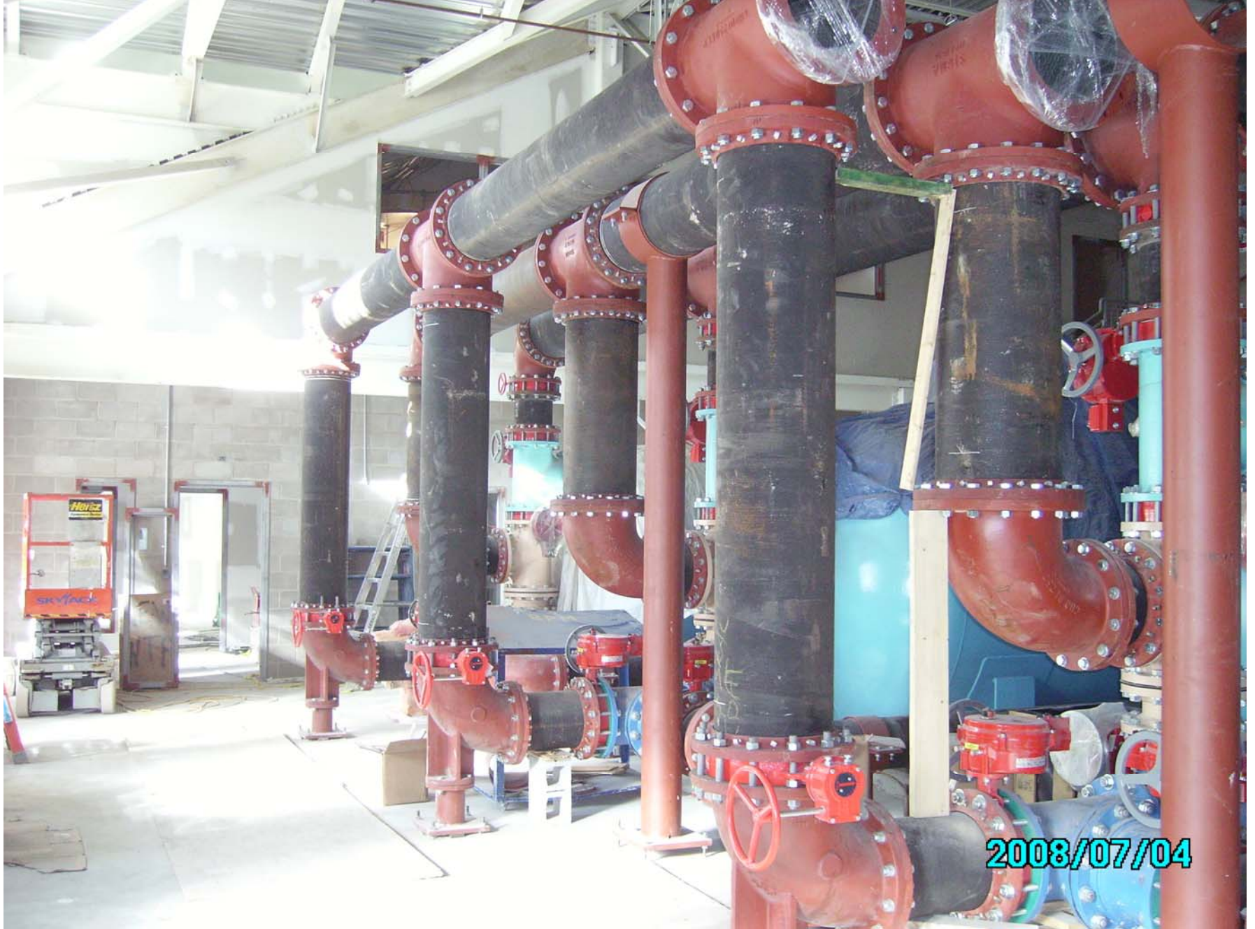
Filtration Room – Pipe Galley
