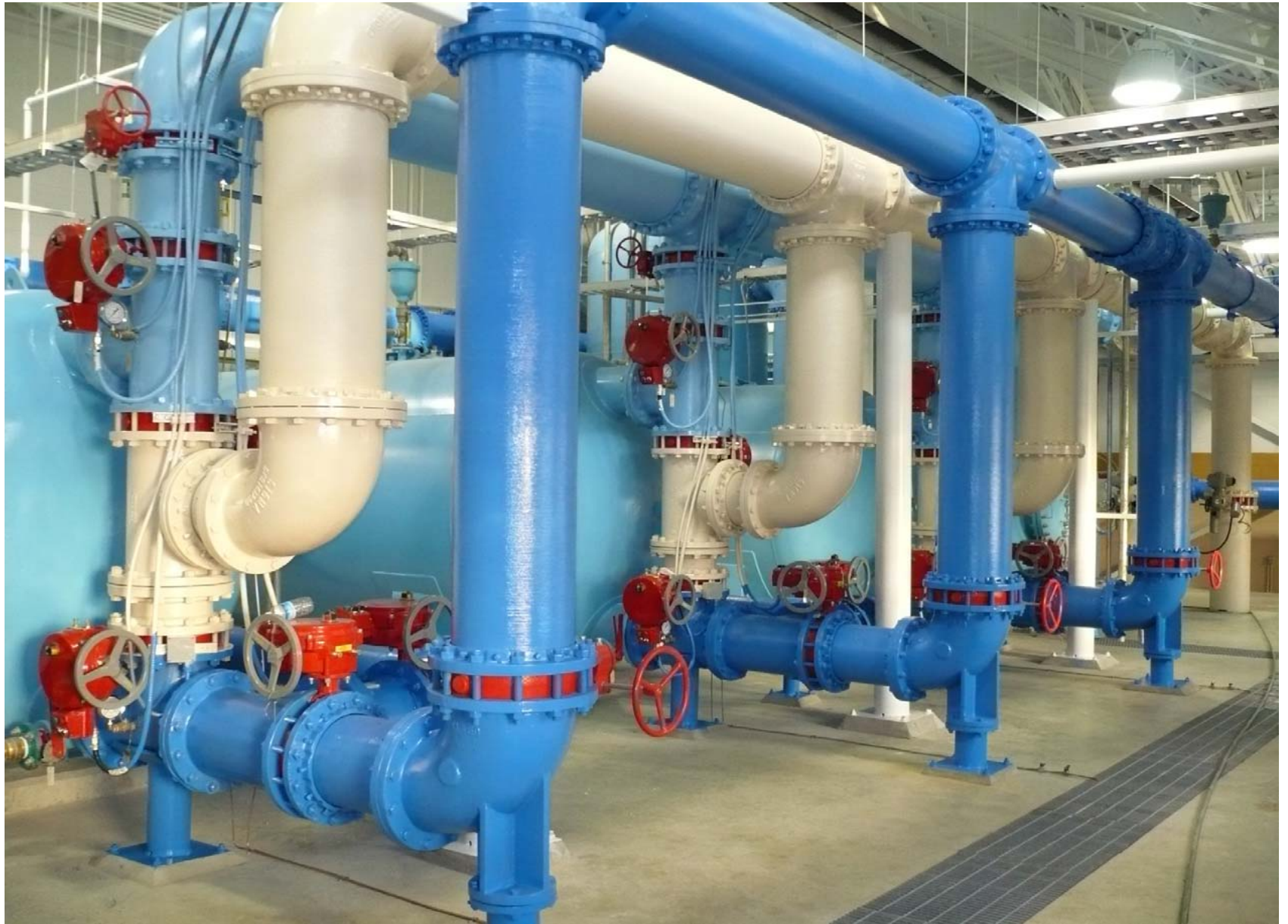
Filtration Room – Pipe Galley
