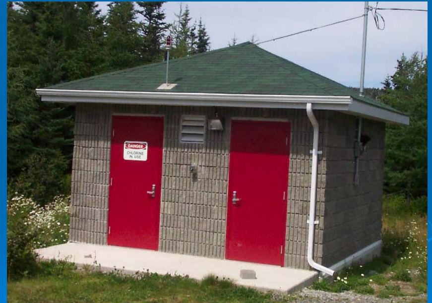
Gas Chlorination Booster
