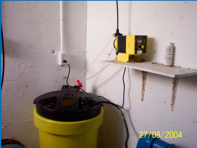
Liquid Chlorination Booster
