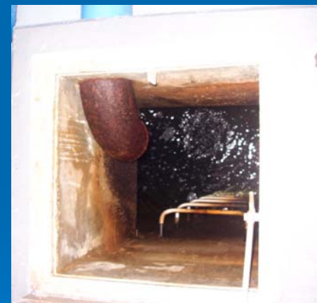
Clear Water Chamber
