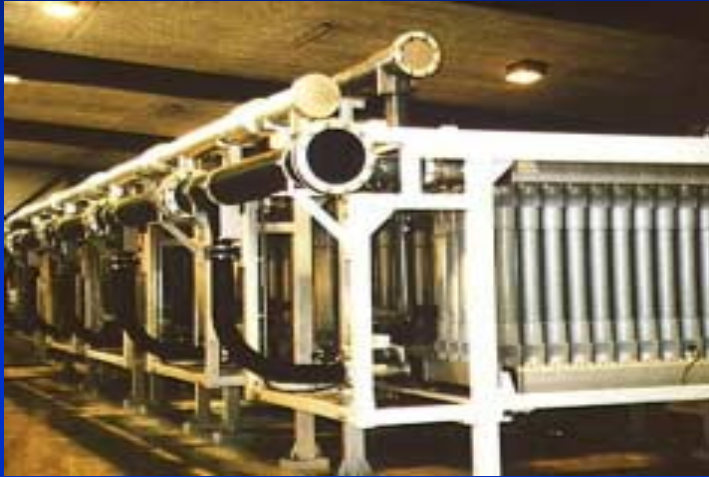
5 Trains of Memcor 90 M10C pressurized modules
