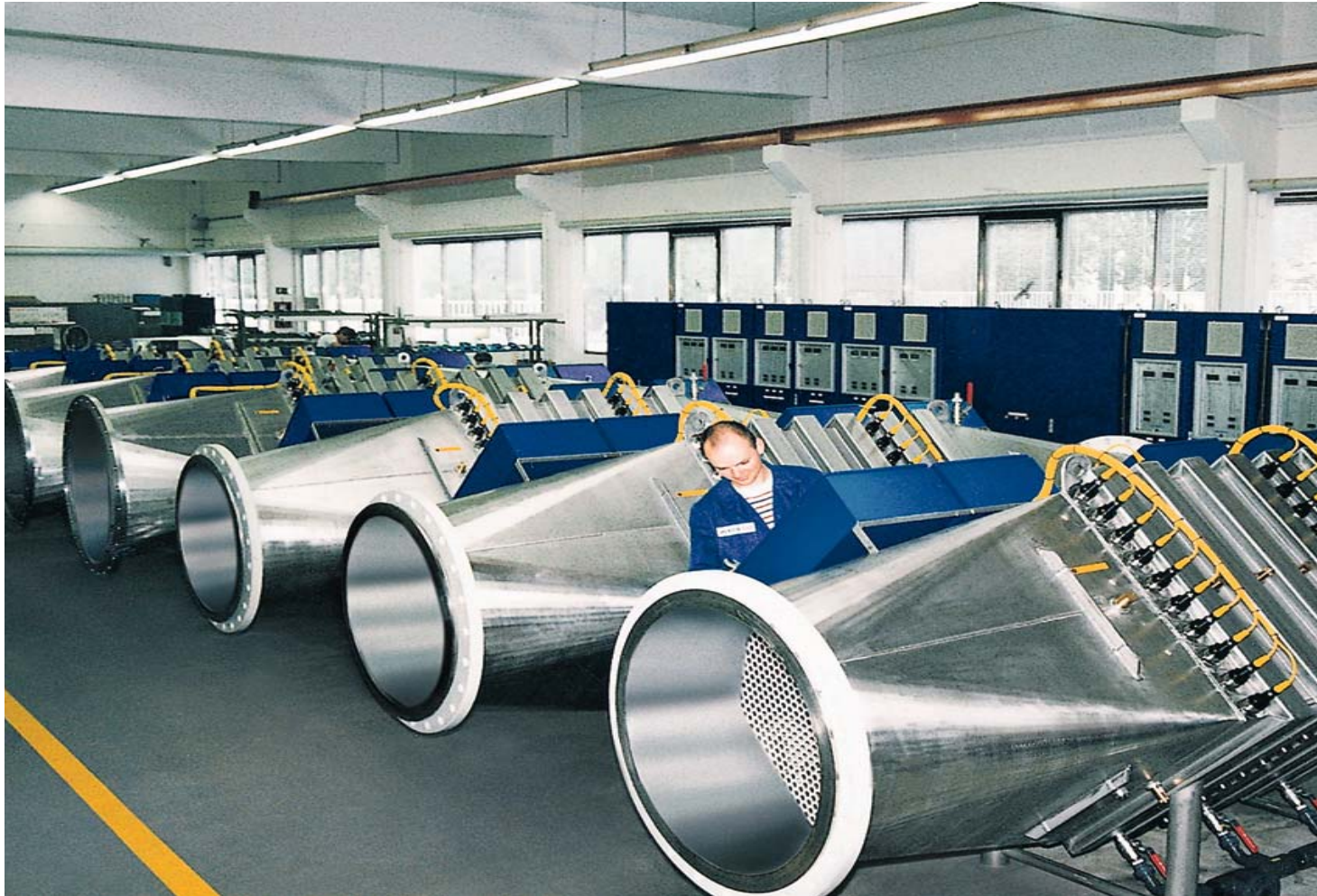
UV disinfection drinking water facility in Helsinki, Finland (Wedeco)
