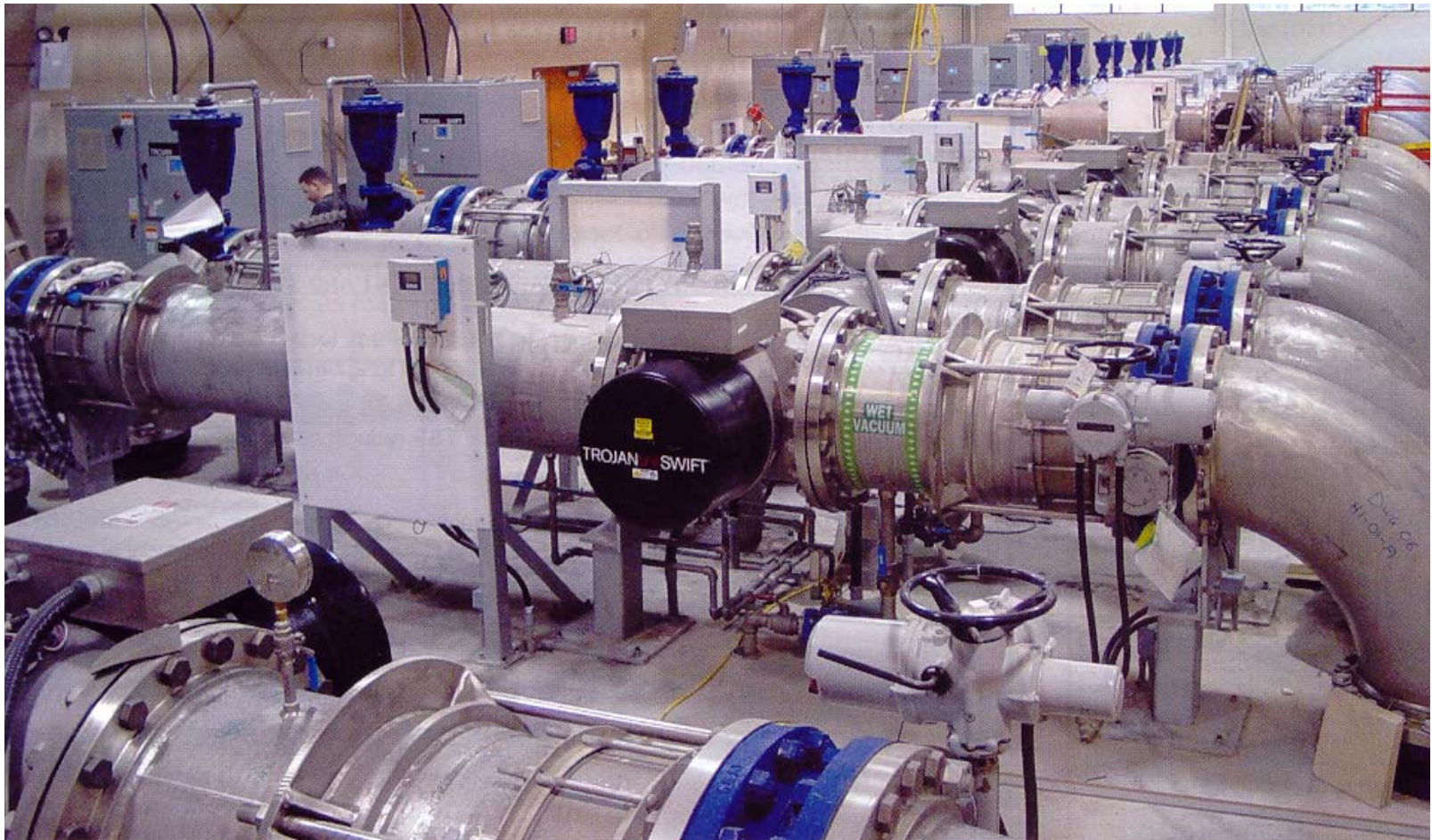
UV disinfection drinking water facility in Victoria (Trojan Technologies)
