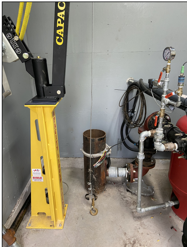
Figure 4: Well Casing in the hut
