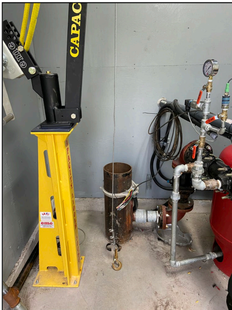
Figure 4: Well Casing in the hu
