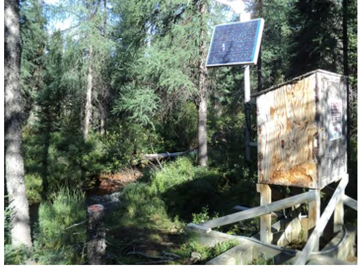
Figure 13: RTWQ hut at Tributary to Reid Brook
