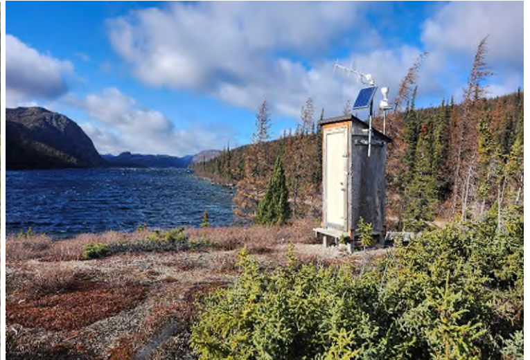
Figure 5: Reid Pond Brook station hut (October 2024)
