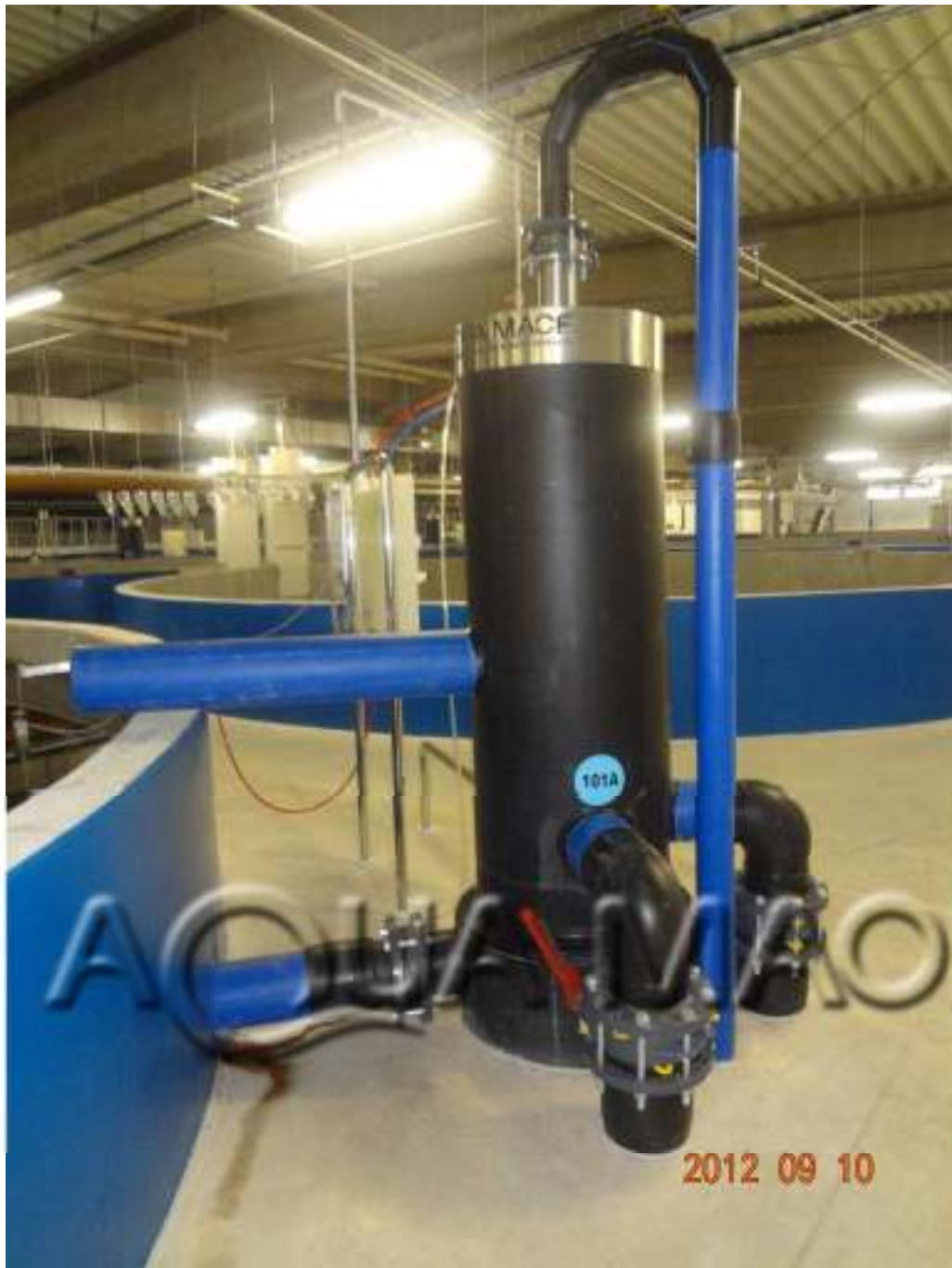
AquaMaof oxygen dissolving system (ODS) showing duplicate water supply from the pipes on lower portion. The duplicate water supply pipes are connected separately to duplicate water pumps. The pipe extending to the top is for adding new water as required. Oxygenated water flows from the ODS through the tank sidewall. The pipe extending from the ODS over the tank sidewall is an overflow pipe.
