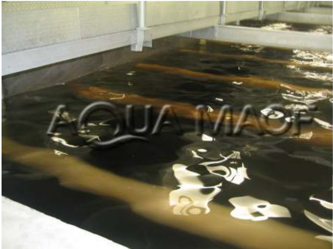
AquaMaof solid waste settler in operation. The pipes visible below the water surface are the water collection pipes distributing water to the biofilter spray nozzles. Water pressure for the spray nozzles is supplied by gravity flow.
