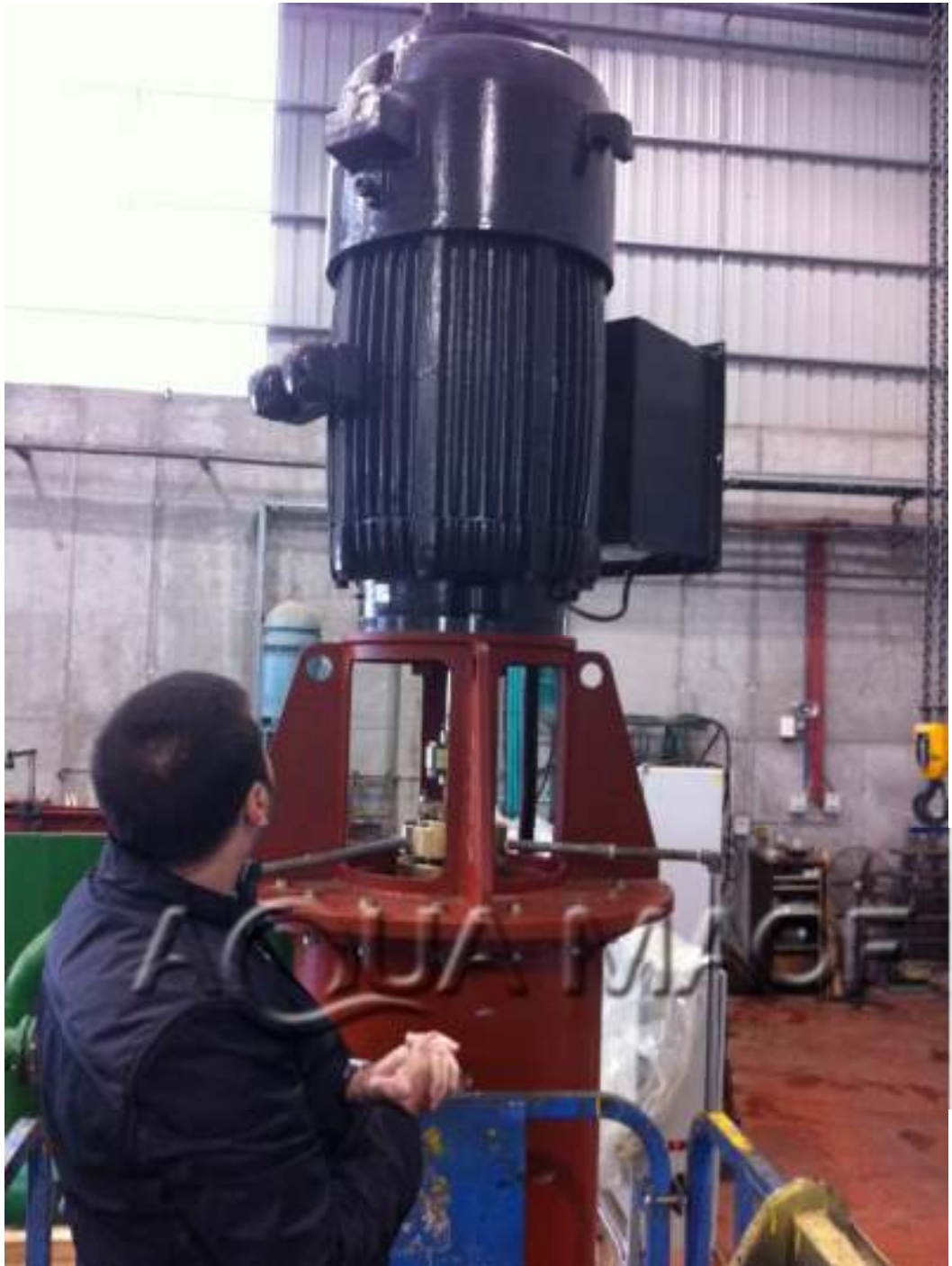
Example of water circulation pumps used in AquaMaof systems.
