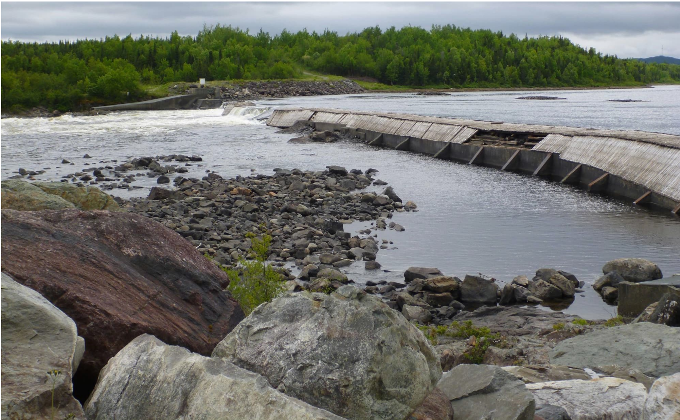
Figure 5-6: Image of Goodyears Dam (looking south) during 2015 breach (June 23, 2025) showing substrates and substrate depth relative to the dam crest behind the northern section
