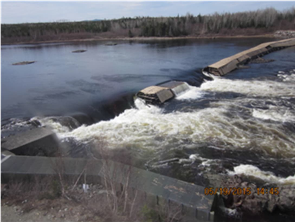
Two sections of timber crib failed
