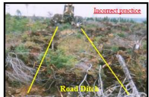
Trenches should not flow into ditches
