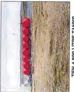
TEN 4,500 LITRE TANKS WITH PIPELINE
