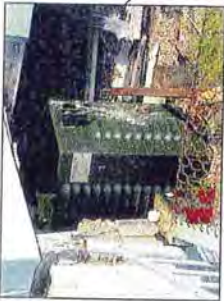
DRY TRANSFORMER UNDER CAMP BUILDING #1
