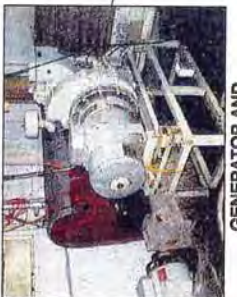
GENERATOR AND 907 LITRE DIESEL TANK
