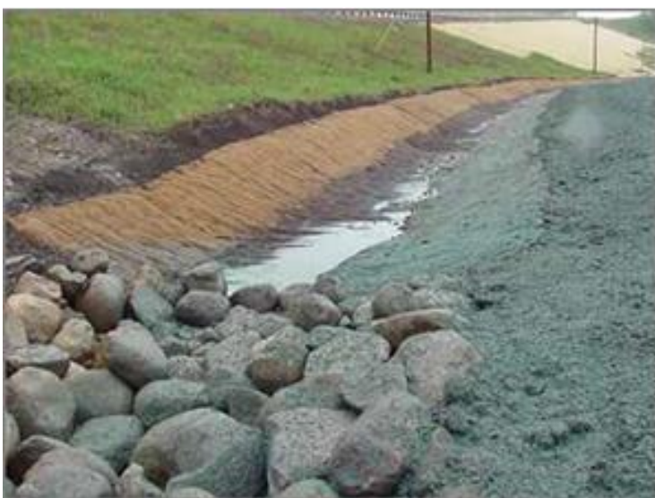
Figure 11-25 - Photograph Shows Erosion Control Blanket on Slope And Erosion Control Mat in Channel
