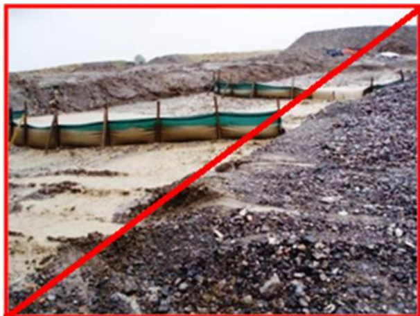
Figure 11-35 - Examples of Poorly Installed Silt Fences
