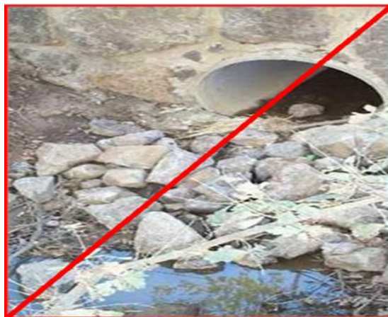
Figure 11-31 - Incorrect Construction of Rock Energy Dissipaters
