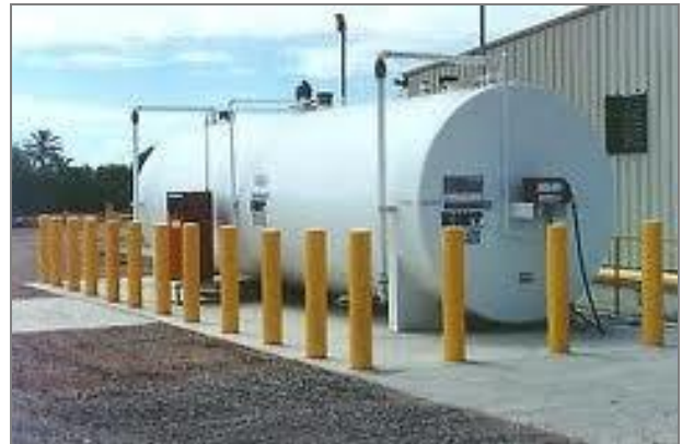
Figure 11-6 - Fuel Storage on Concrete Pad
