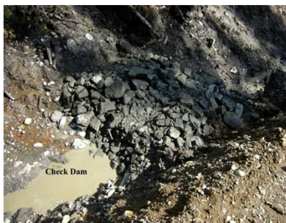
Figure 11-4 - Photograph of Rock Constructed Check Dam
