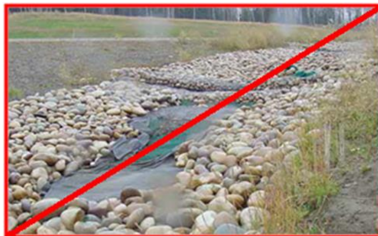
Figure 11-27 - Photograph of failed Rip Rap Protection a Slope
