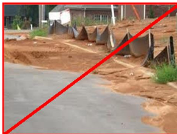
Figure 11-36 - Examples of Poorly Installed Silt Fences
