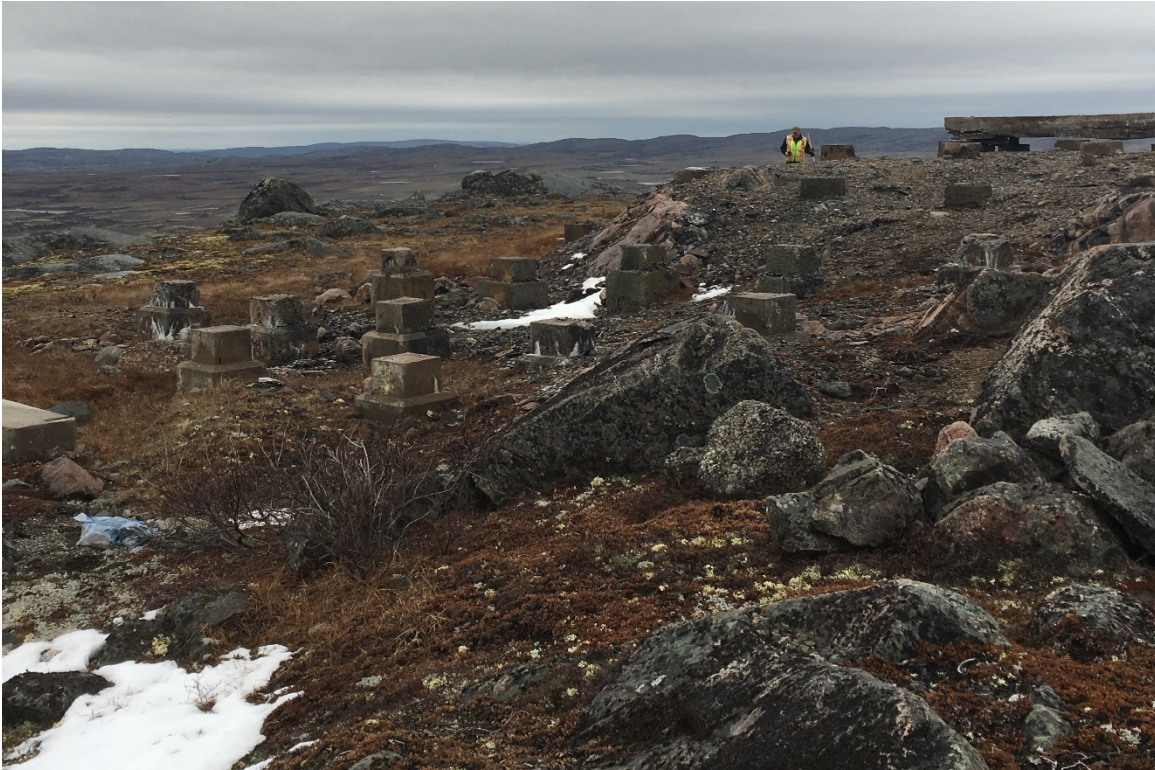
Photo 23 – Upper Site: concrete slab and pillars of Former Operations Building. Looking southwest.
