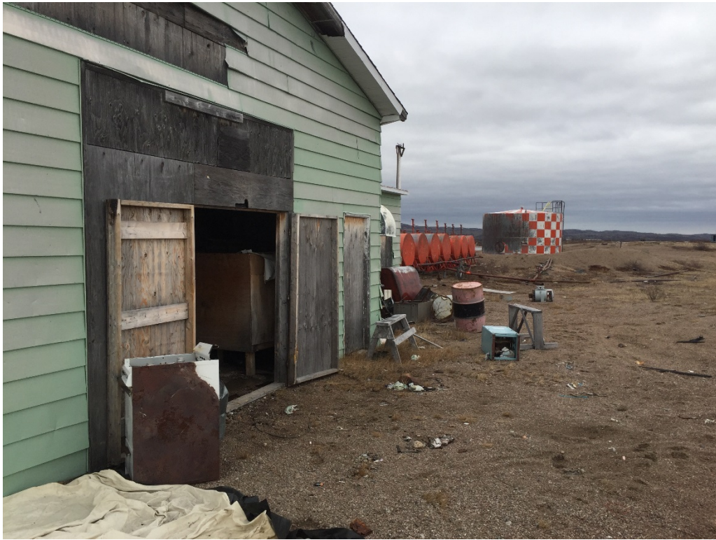
Photo 7 – Camp / Antenna Areas and AES Compound: Camp Garage Building. ASTs and Dyked Tank visible in background. Looking east.
