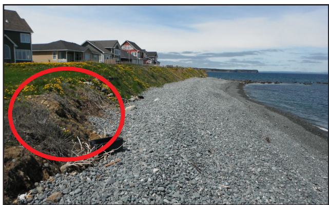
Plate 8. Homeowners placed grass, woody debris and soil (circled) to advance the face of the cliff in Conception Bay South. As this material is loose, it is very vulnerable to erosion during a period of high wind or elevated water, and will likely be displaced during the next storm event.
