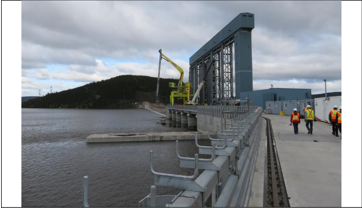
Photo A.1: Northerly view along upstream side of concrete structures with reservoir at full pool level.
