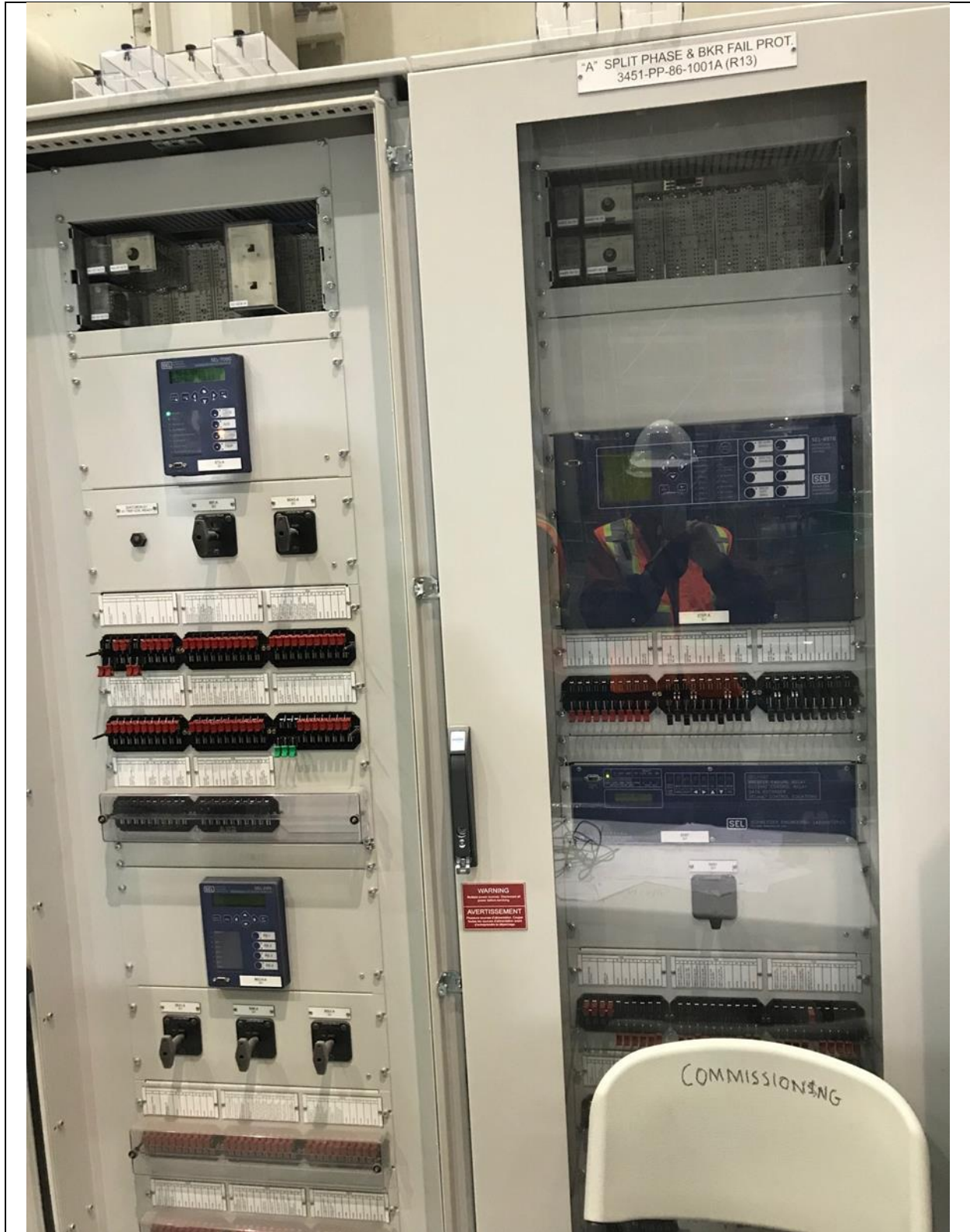
Photo B.6: Protection switchboards.
