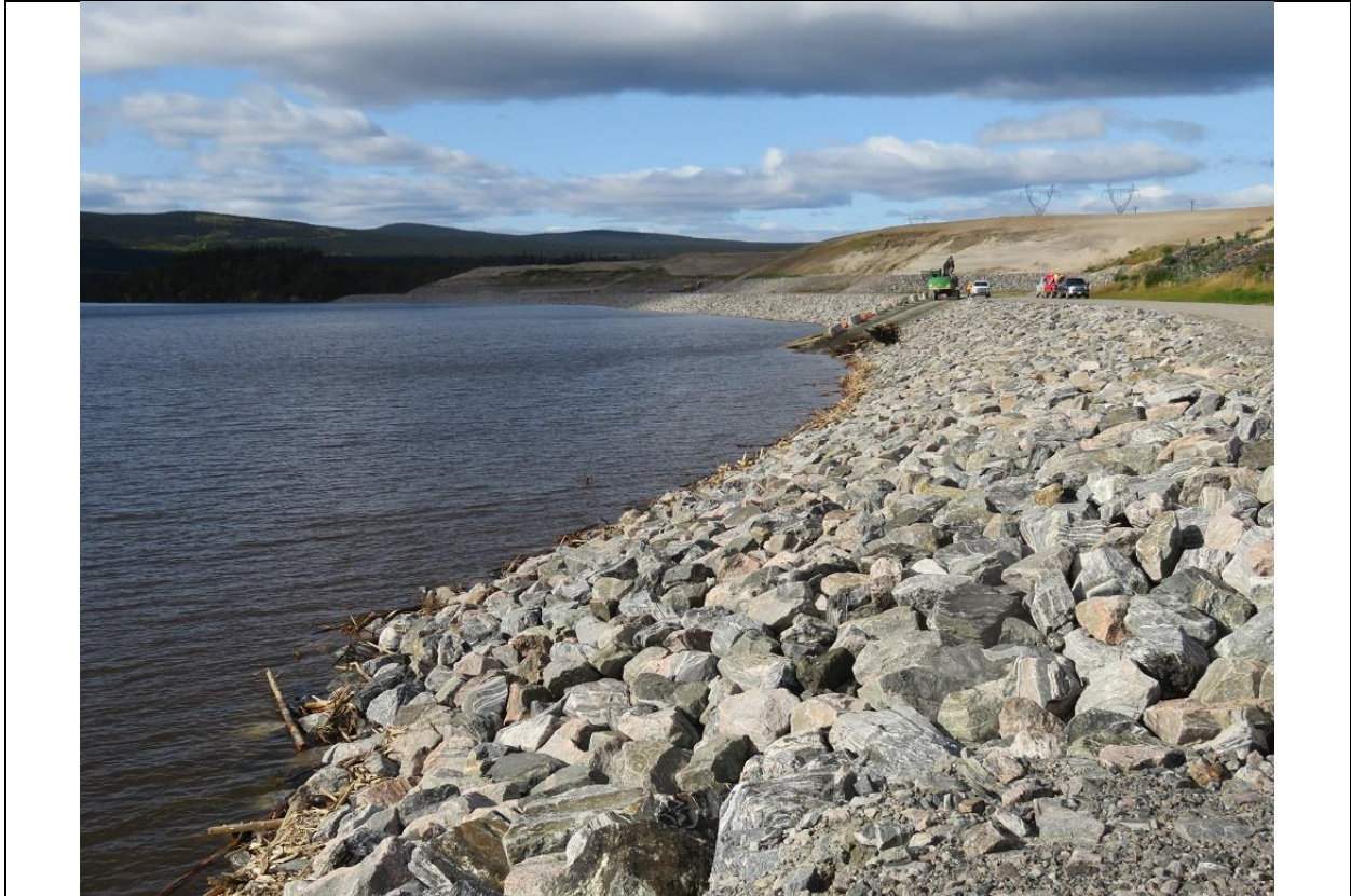
Photo D.1: Upstream side of North Spur. Collected floating debris is removed from reservoir via the ramp near centre of photo.
