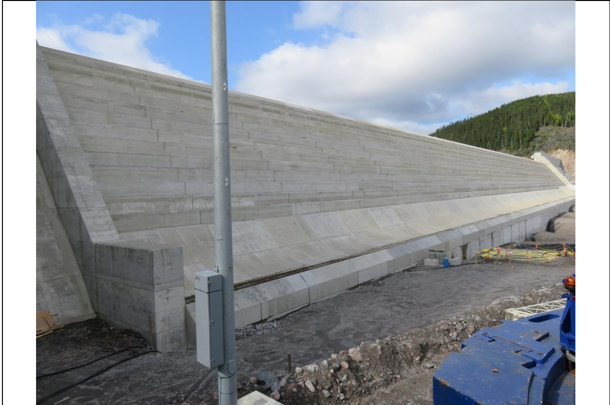
Photo A.4: Downstream side of north RCC dam. Local areas of minor leakage along base appear to be from water ponded in the flip bucket that is draining through construction joints.
