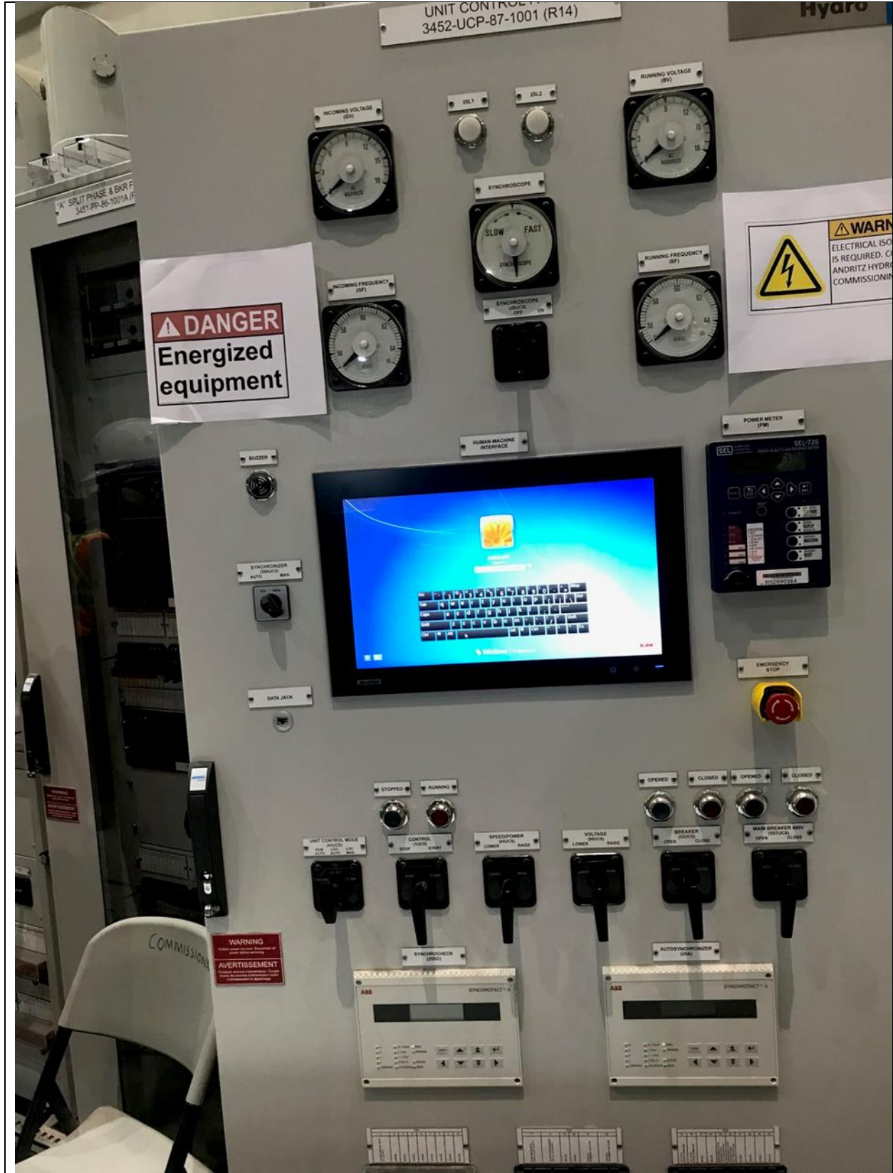
Photo B.7: Unit control board.
