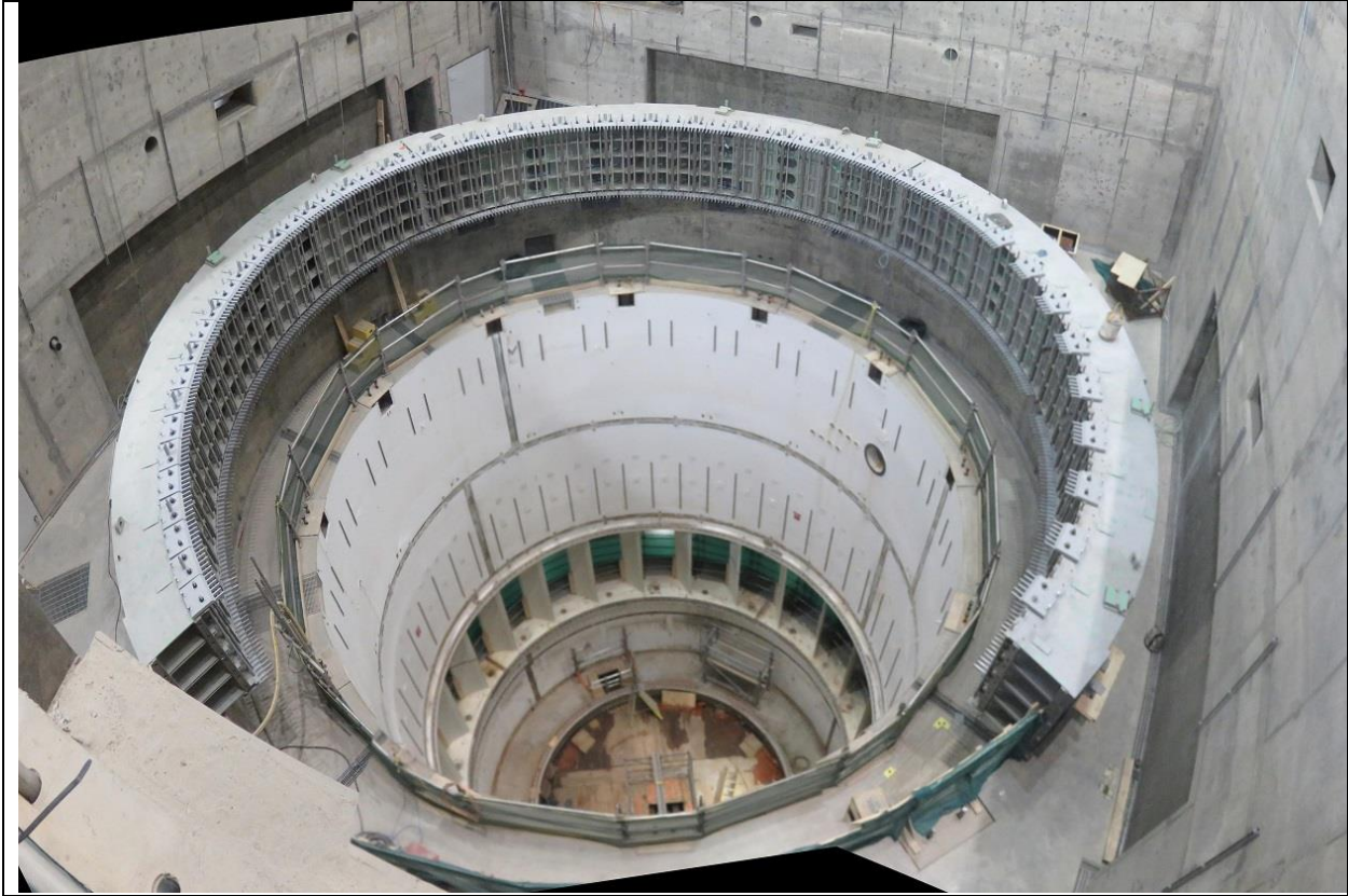
Photo B.5: Unit 4, with partially installed stator frame.
