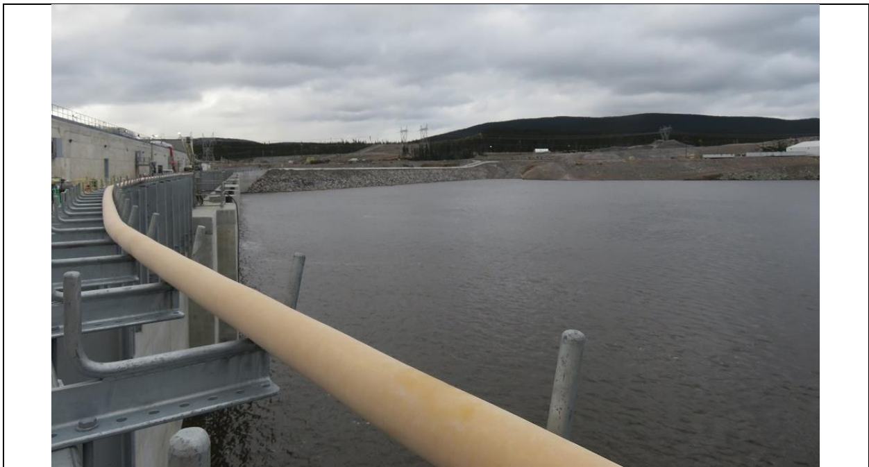
Photo A.2: Southerly view along upstream side of power intakes with south embankment dam in background.
