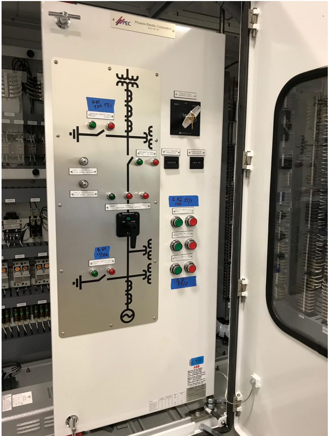
Photo 3: Detail- Mimic board with local controls and display
