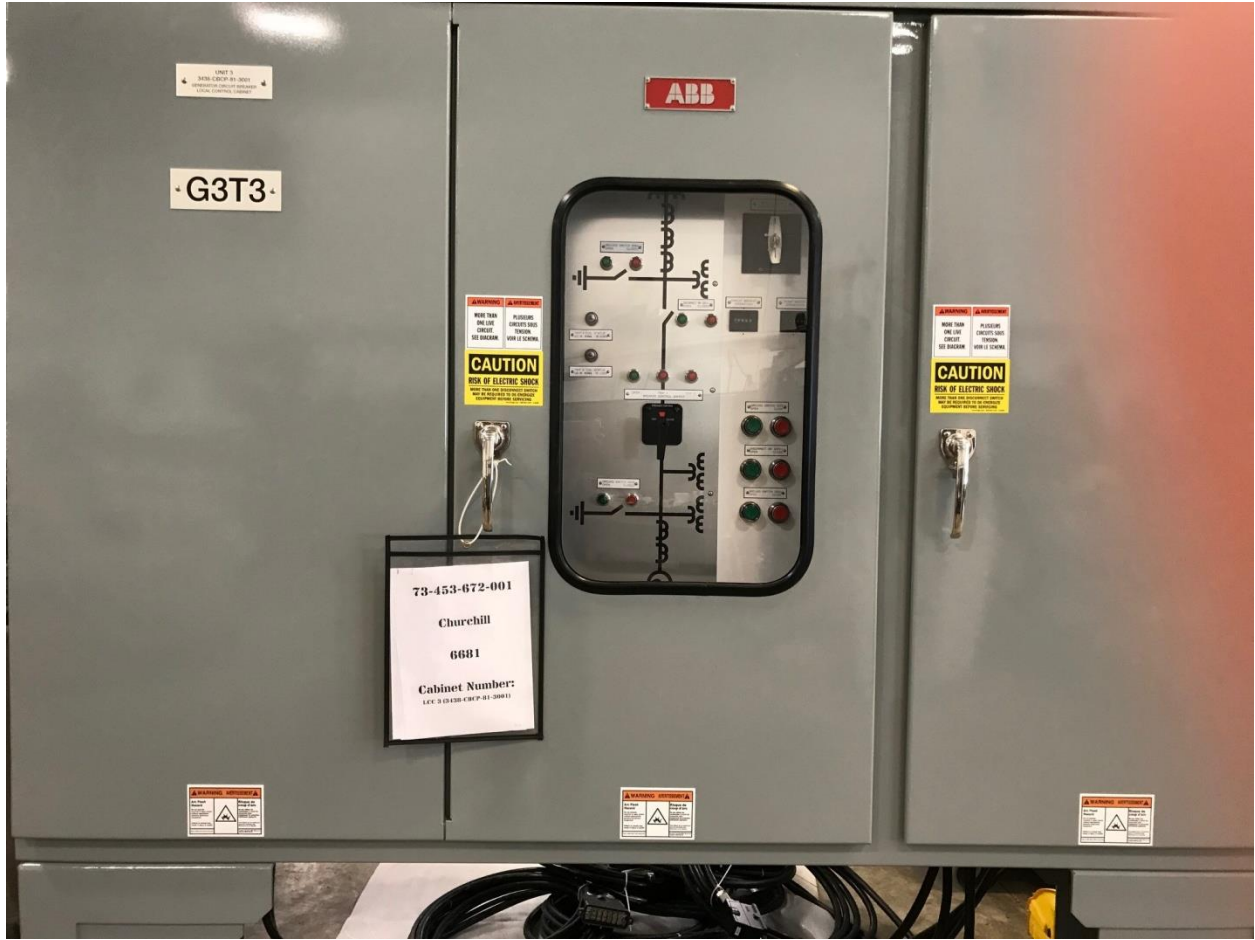
Photo 1: MFA GCB Local Control Cabinet (LCC)
