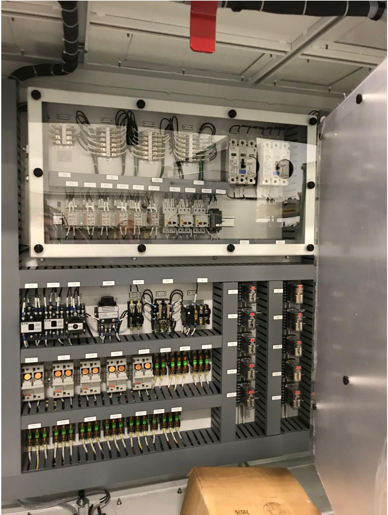
Photo 2: LCC auxiliary relays and fusing
