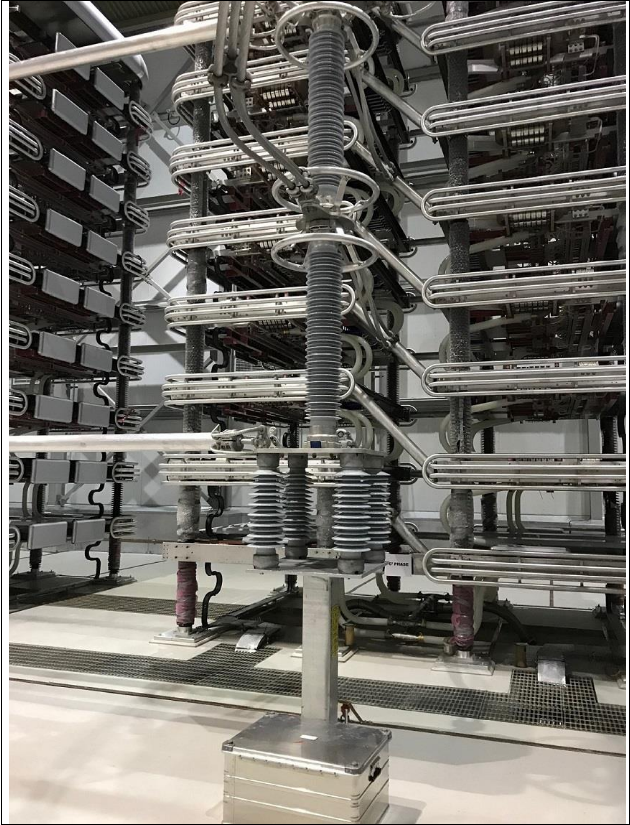
Photo E.3: HVDC valves.
