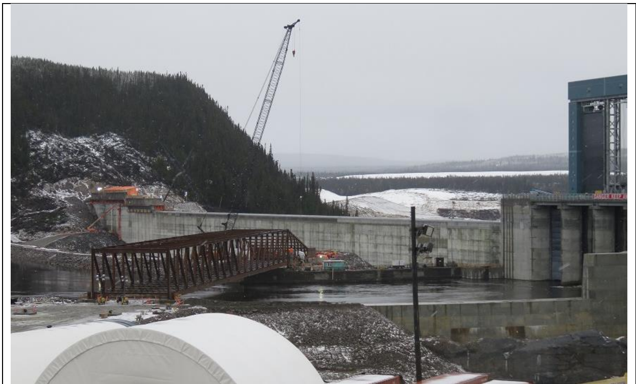
Photo A.2: Removal of temporary construction bridge in progress with completed North RCC dam in background.
