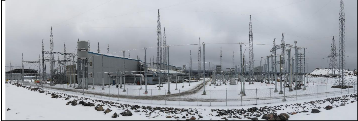
Photo E.1: GIS building and yard.
