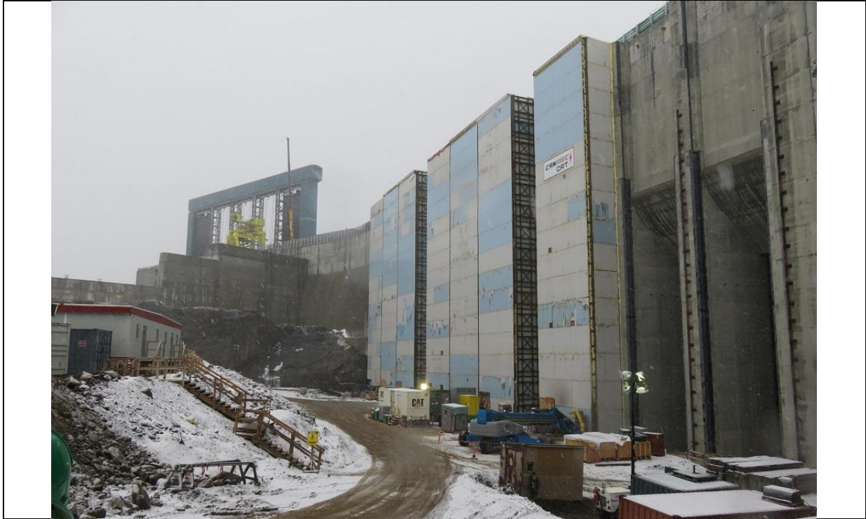
Photo B.1: Power intakes with temporary hoarding and heating in place for completion of second stage concrete for gate guides.
