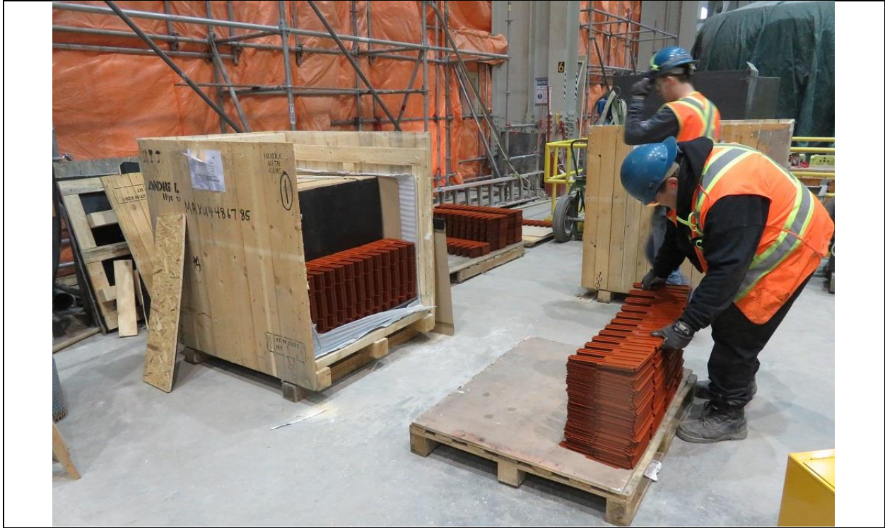
Photo B.6: Unpacking lamination plates for generator stator core.
