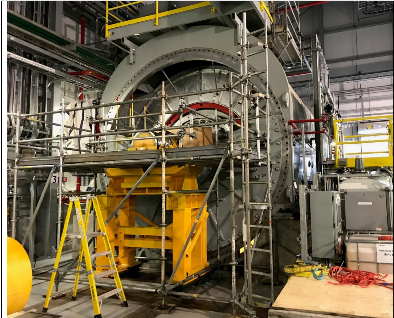
Photo F.1: SOP Unit 1, bellhousing removed.
