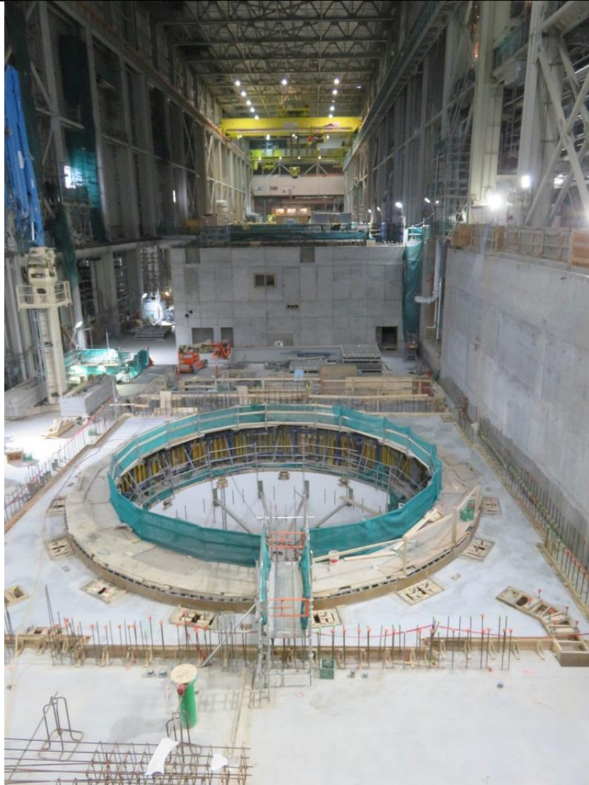
Photo B.5: Interior view of powerhouse from north service bay with Unit 4 in foreground.
