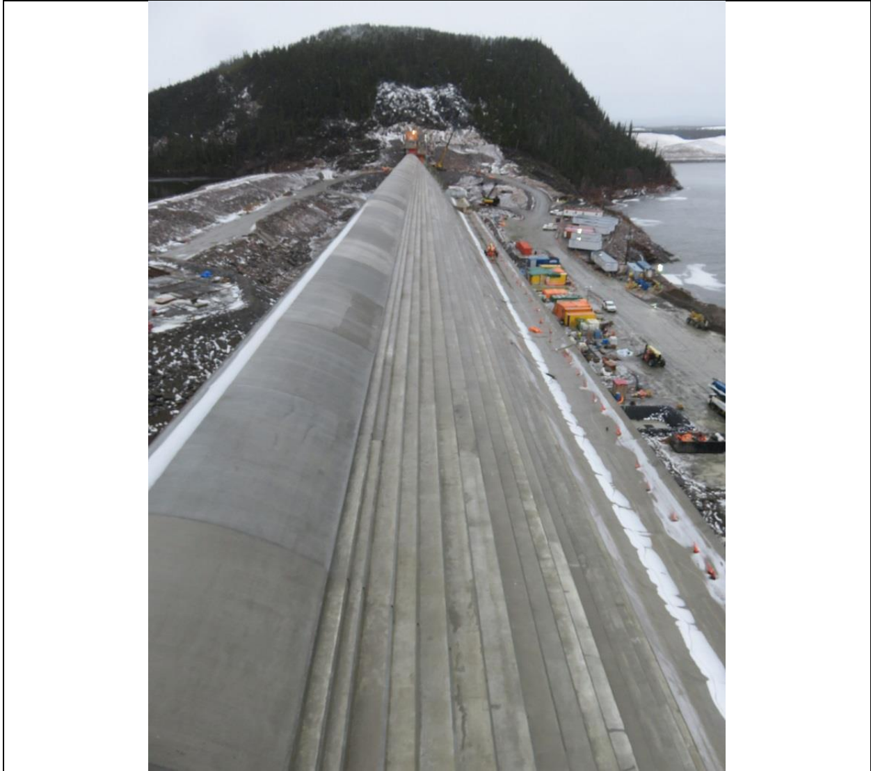
Photo D.1: View from north transition dam looking northerly along top of completed north RCC dam.
