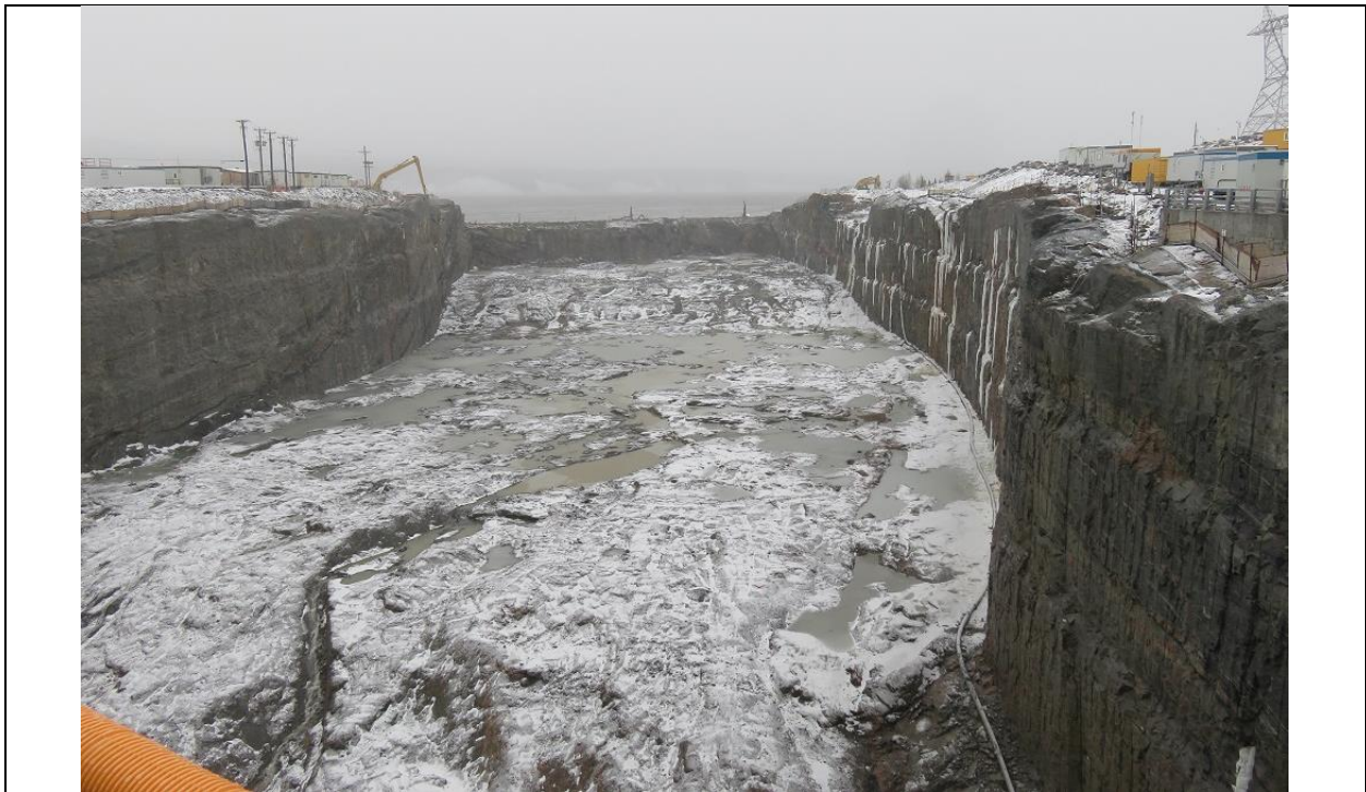
Photo B.10: Removal of rock plug at downstream end of tailrace channel is in progress.
