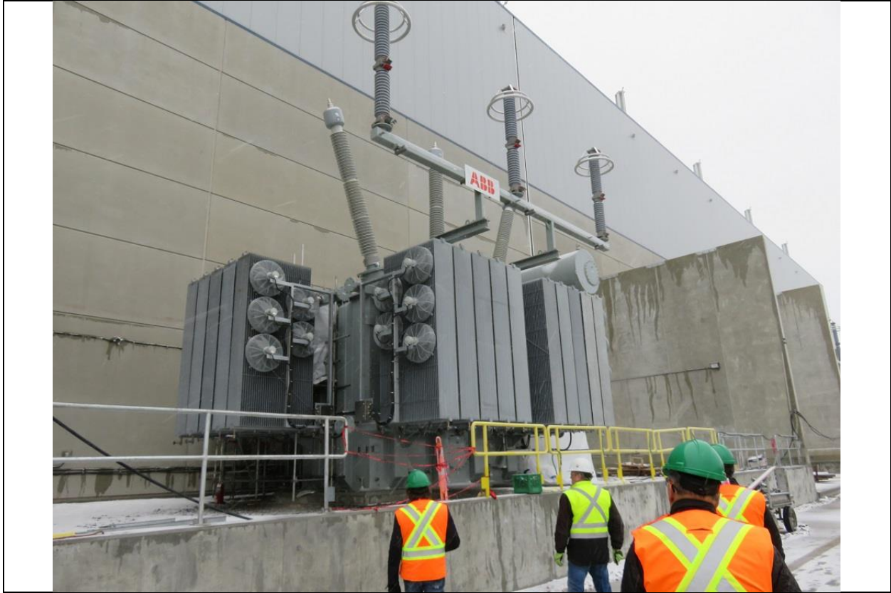
Photo B.9: Generator transformer installed on tailrace deck.
