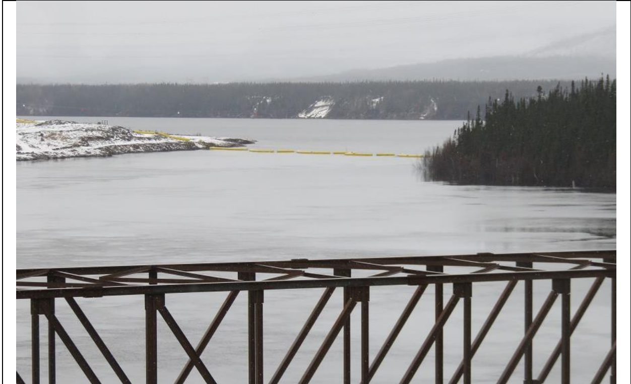
Photo A.1: Upstream view of debris/ice/safety boom. Buoy clamps were replaced, and buoys repositioned along main cable.
