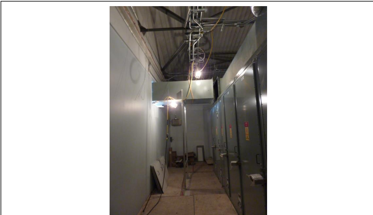
Photo F.10: AC Substation 25kV switchgear arc flash vent detail.
