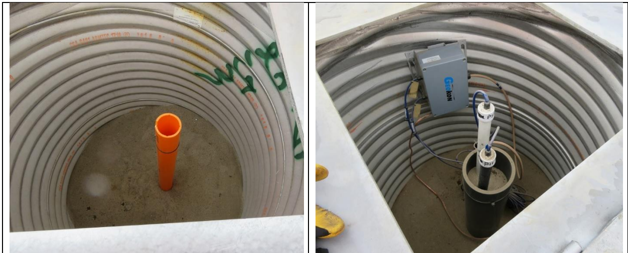
Photo E.9: Typical instrument installations installed inside protective CMP collars with locked steel lids. Inclinator at left and dual vibrating wire piezometers with remote readout system at right.
