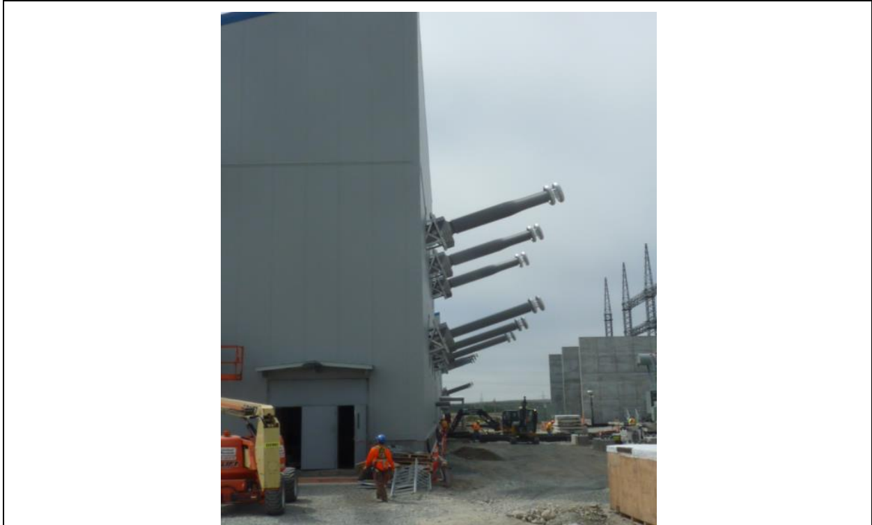
Photo H.1: Converter Station AC Wall Bushings.
