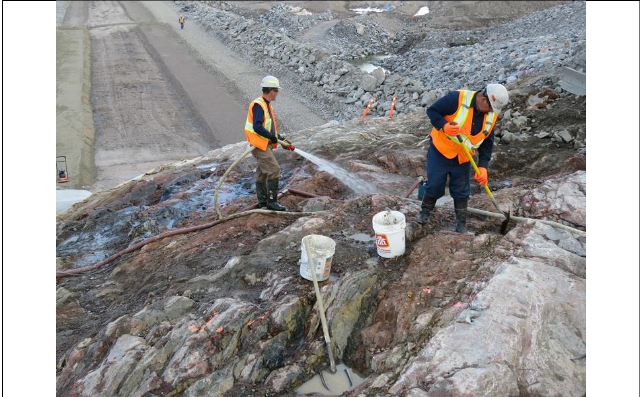
Photo D.3: Final cleanup of foundation bedrock surface by hand methods at right abutment of south embankment dam.
