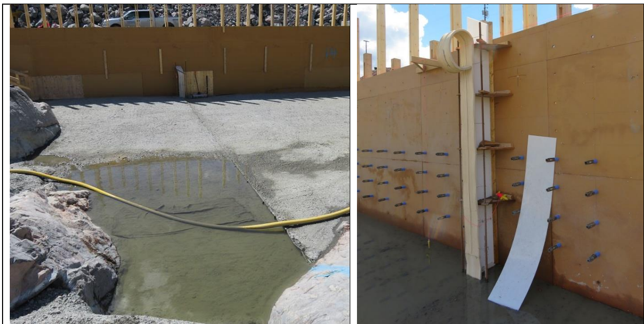
Photo C.8: Typical contraction joint in leveling slab, created with embedded “Stayform”, with waterstop at upstream end of joint (left photo). Details of typical waterstop at upstream side of a contraction joint (right photo).
