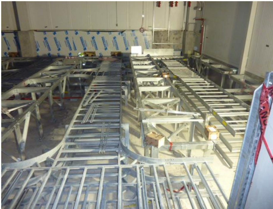
Photo H.8: Converter Station - suspended floor support and cable trays.
