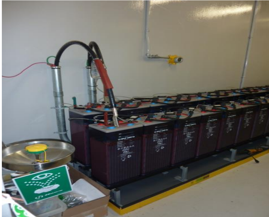
Photo H.13: AC Substation Control Building - Battery #2 Cabling.
