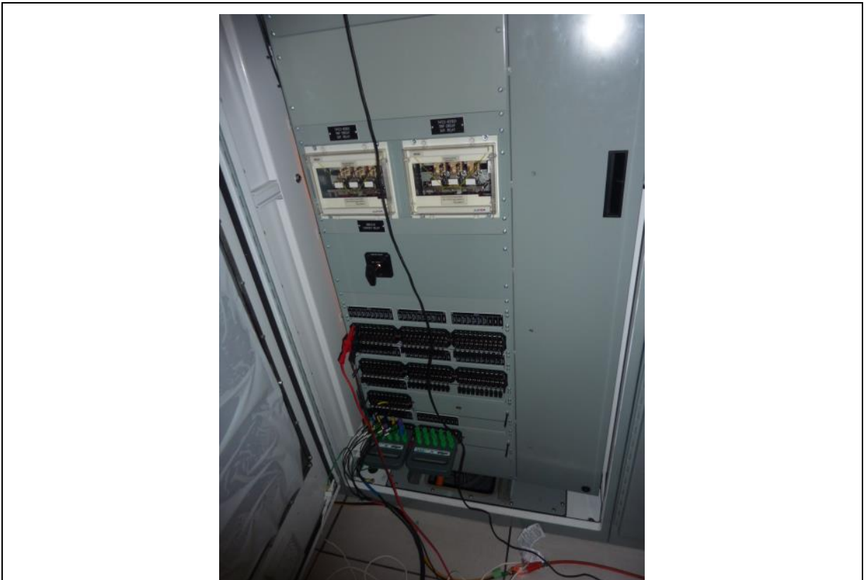
Photo H.12: AC Substation Control Building - relay panels in place undergoing testing.
