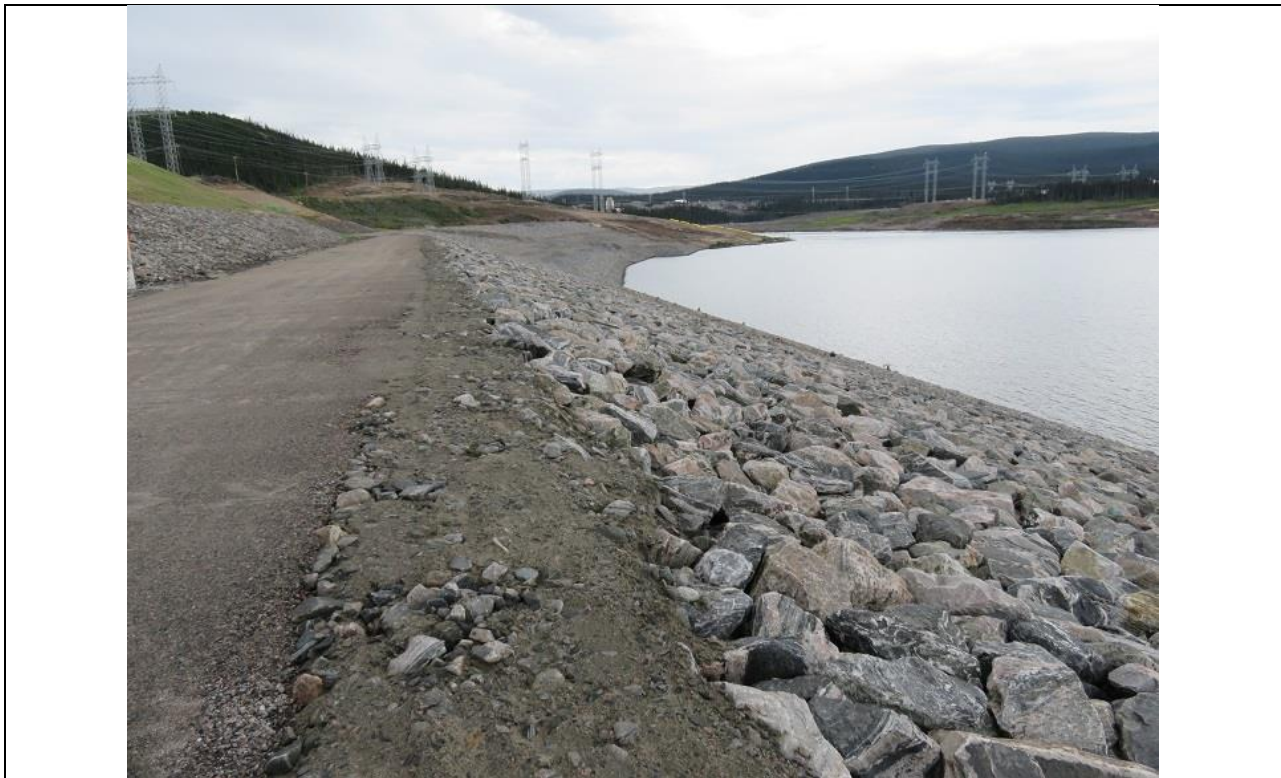
Photo E.2: Southerly view along upstream side of North Spur slope stabilization works.
