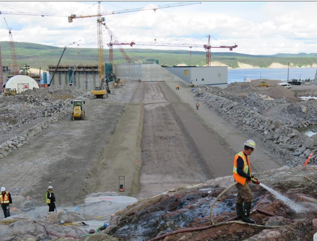
Photo D.2: Northerly view along south embankment dam towards south transition dam which forms the left abutment. Boundaries between zones of different materials are well-defined.
