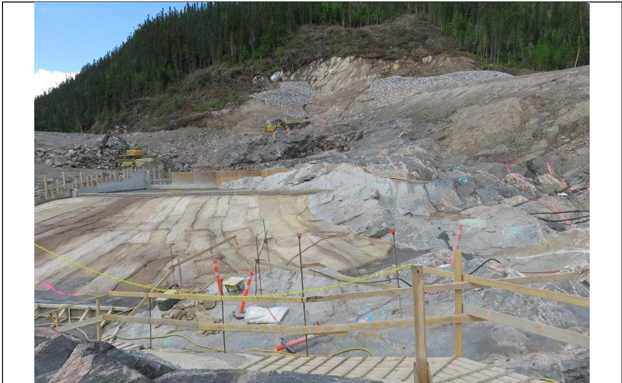
Photo C.4: Northerly view along RCC dam foundation. Area stripped to rock in background indicates future top of dam. Area at centre-left is recently-placed cast-in-place leveling concrete, covered with wet burlap for initial curing period.
