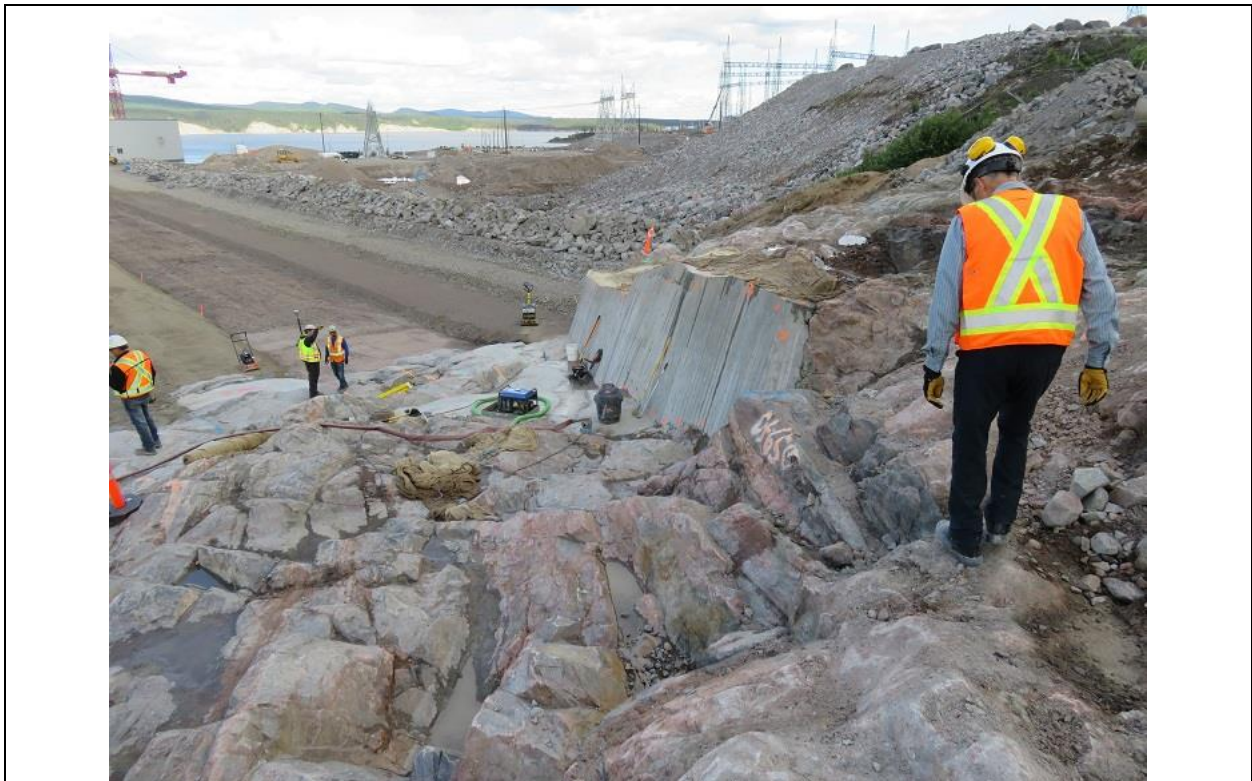
Photo D.4: Cleaned bedrock surface on lower right abutment, ready for dental concrete. Note concrete infill for local shaping of core contact zone in centre of photo.
