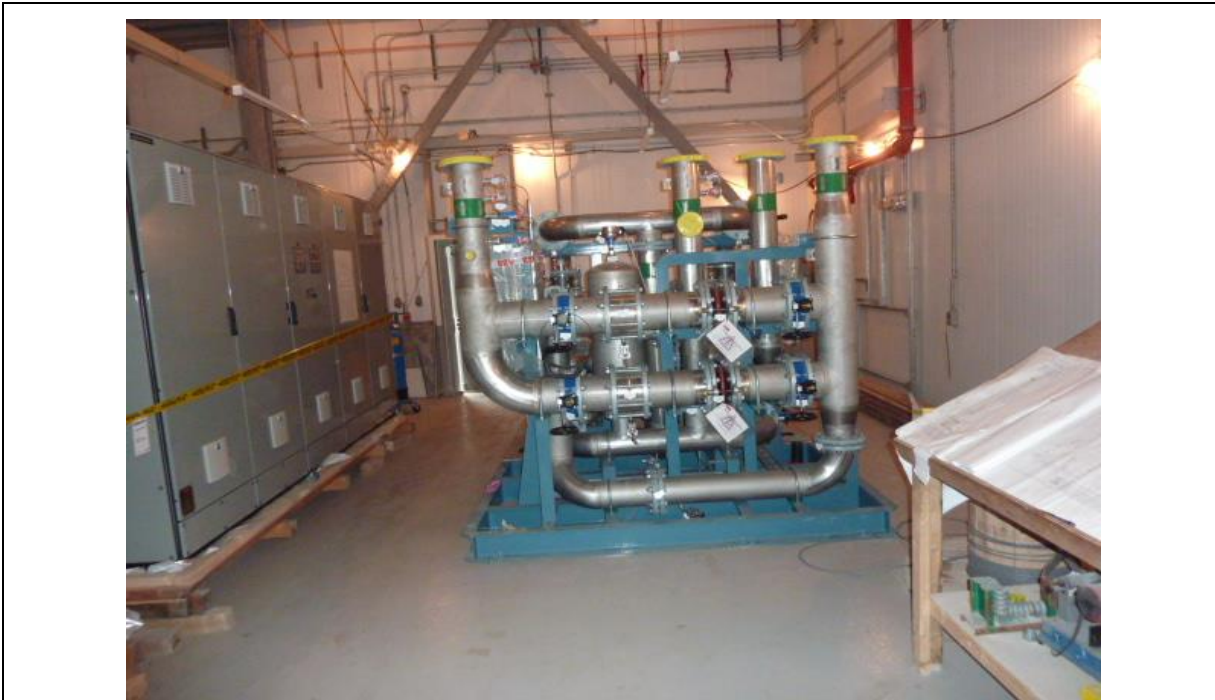
Photo H.5: Converter Station Valve Cooling - Cooling Pumps.
