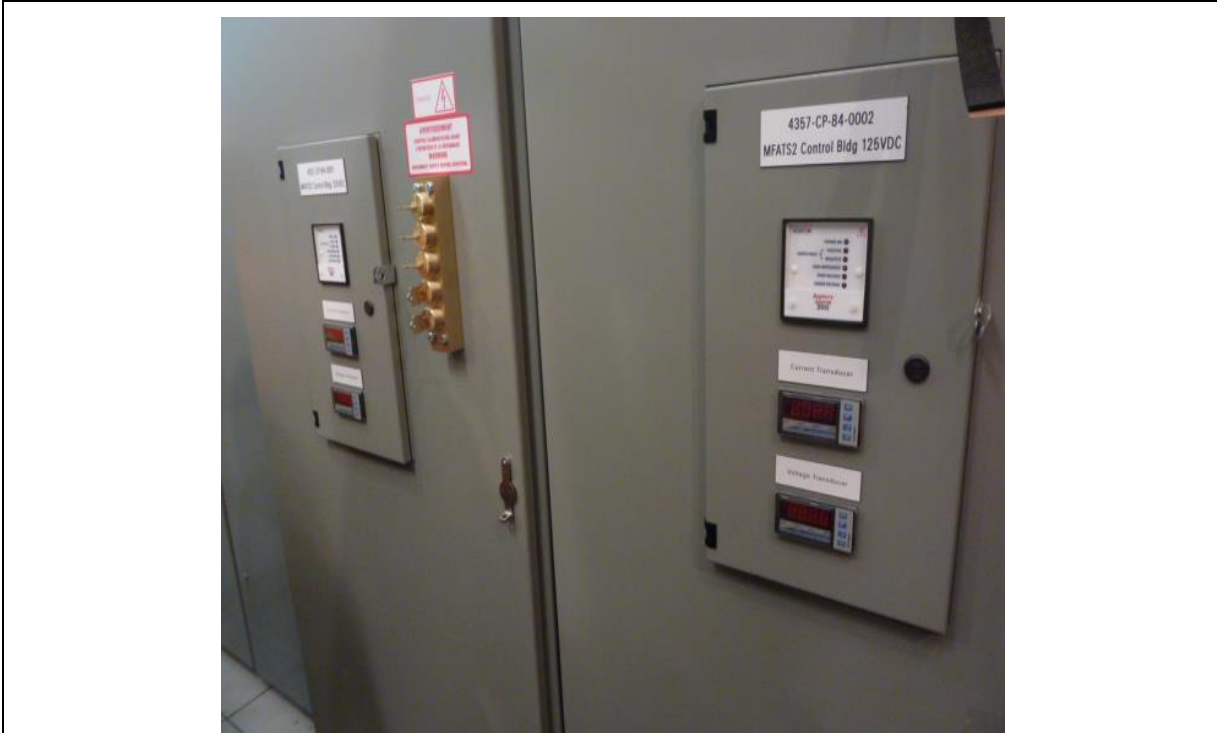
Photo F.11: 125 VDC controls and monitoring detail
