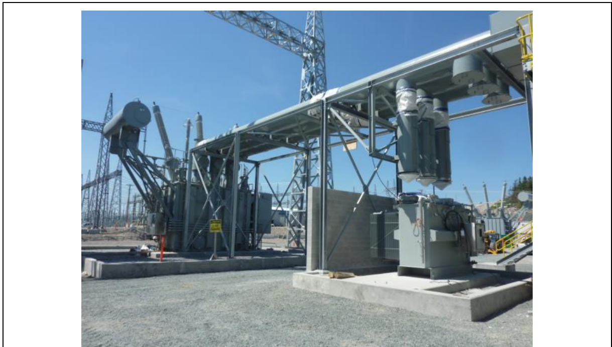
Photo H.18: Synchronous Condensers Power and Exciter Transformers.
