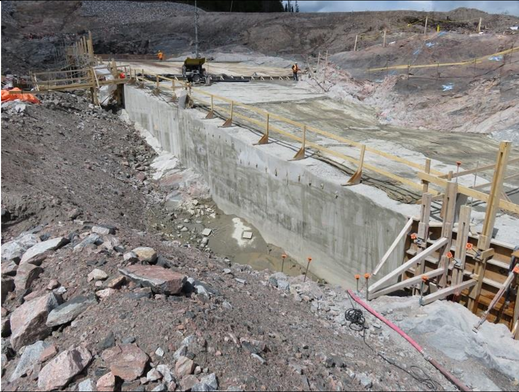
Photo C.9: Upstream side of levelling concrete after formwork removal, showing good contact with bedrock and good compaction of concrete.
