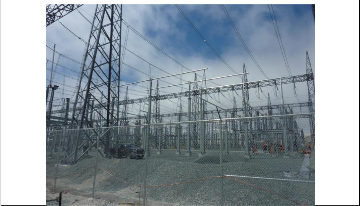
Photo H.11: AC Substation construction has been completed with testing in progress.
