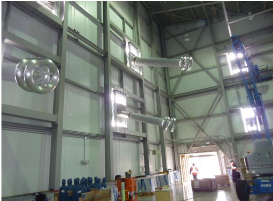
Photo H.7: Converter Station Valve Hall - Sealed floors and DC Wall Bushings are ready for equipment installation.
