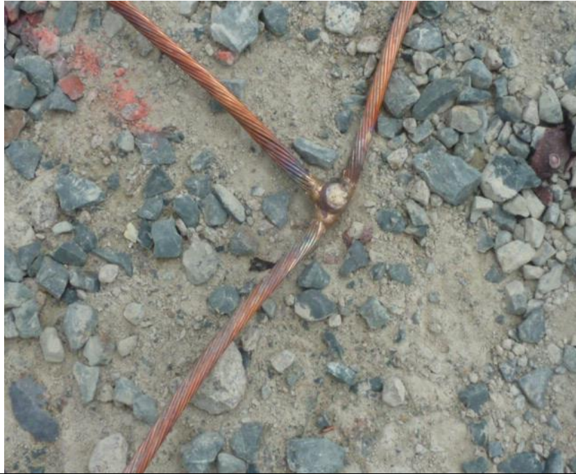
Photo H.9: Converter Station DC Yard - Ground grid cad-weld joint detail.
