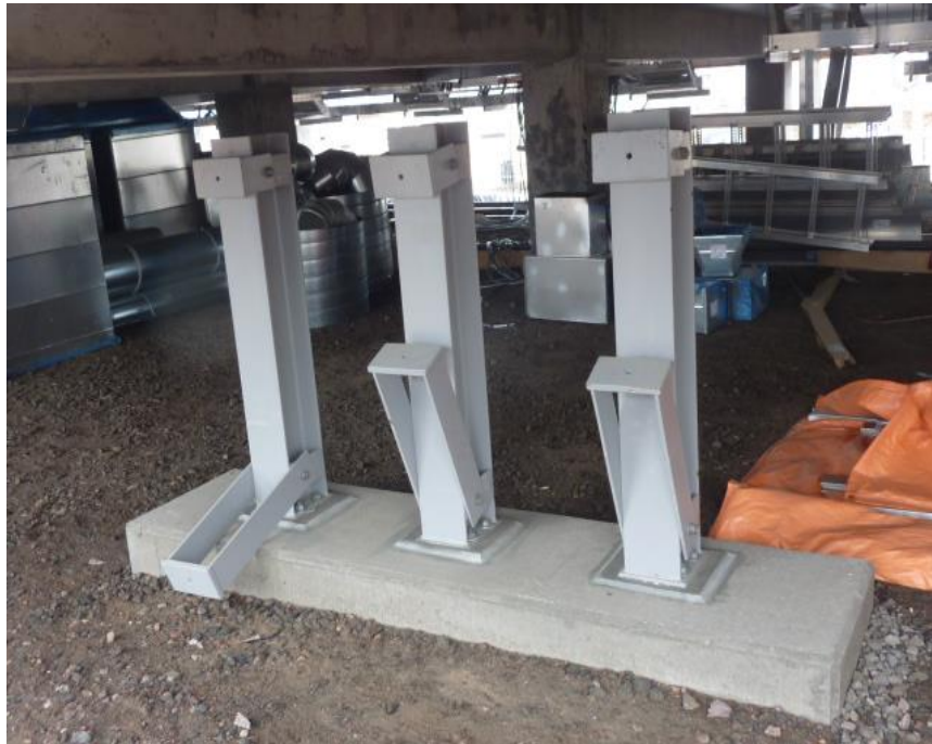
Photo F.7: GIS Building - Powerhouse collector feeder cable supports
