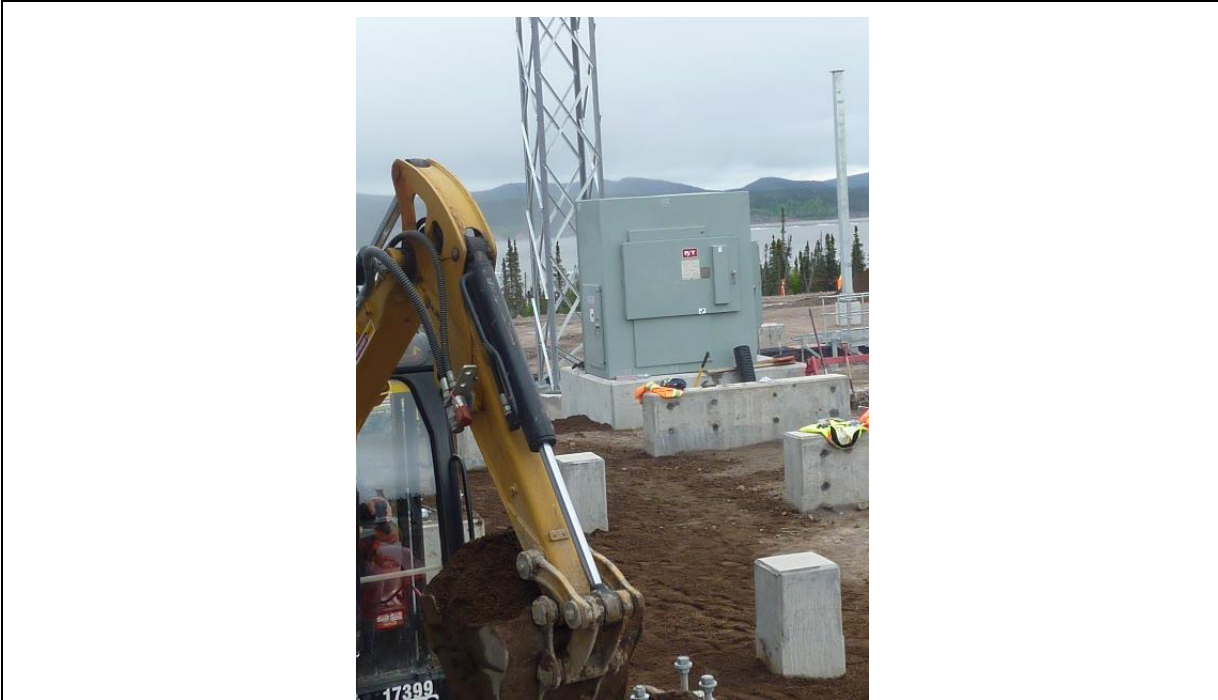
Photo F.5: Station Service Transformer with power connections led underground.
