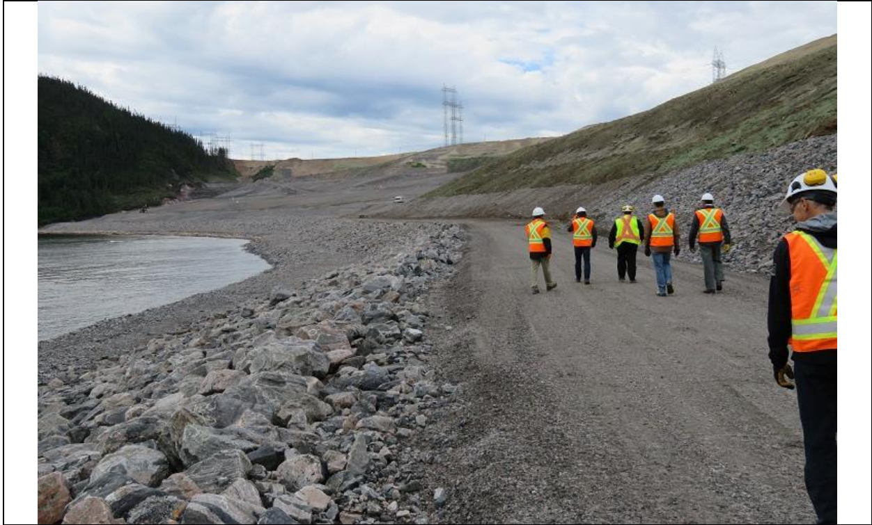
Photo E.8: Southerly view along access road at toe of downstream side of North Spur slope stabilization works.
