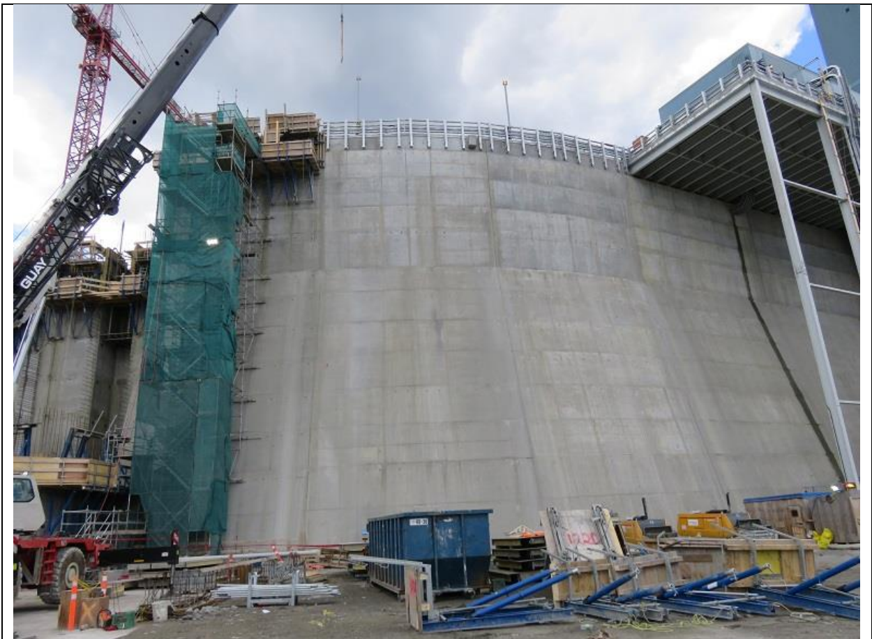
Photo B.2: Central transition dam nearing completion on south side of spillway structure.
