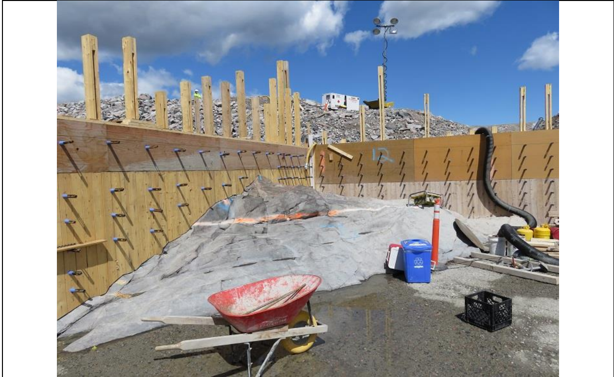
Photo C.5: Typical formwork details on irregular rock surface, with recently-placed leveling concrete in foreground.
