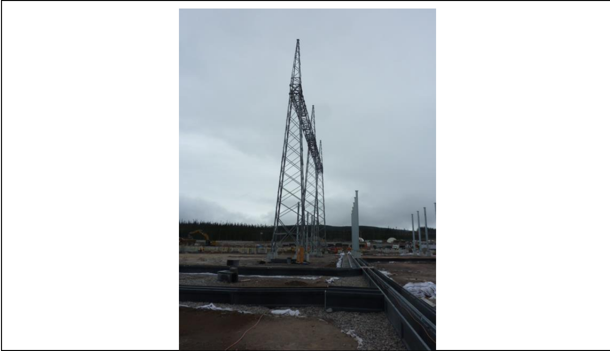
Photo F1: AC yard
