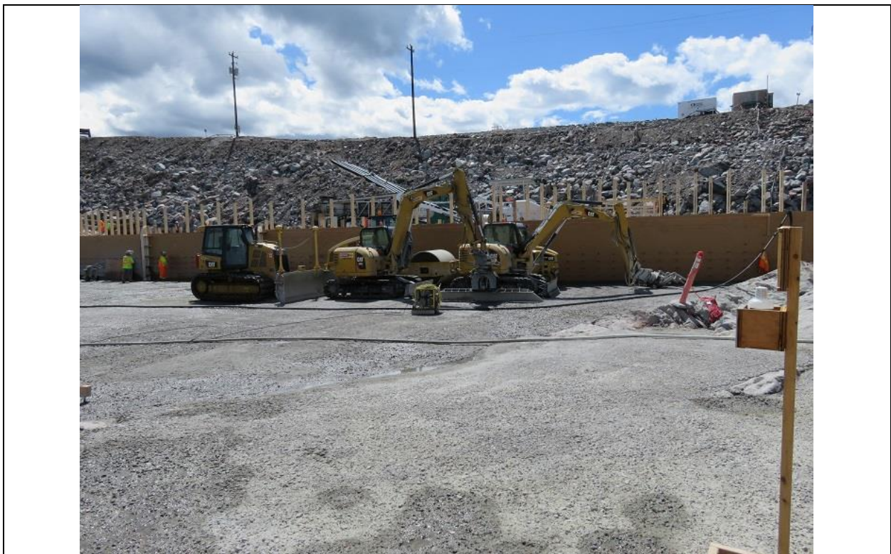
Photo C.6: Typical equipment to be used for RCC placement. Equipment is parked on cast-in-place concrete leveling slab which has been "green cut" with pressurized water.
