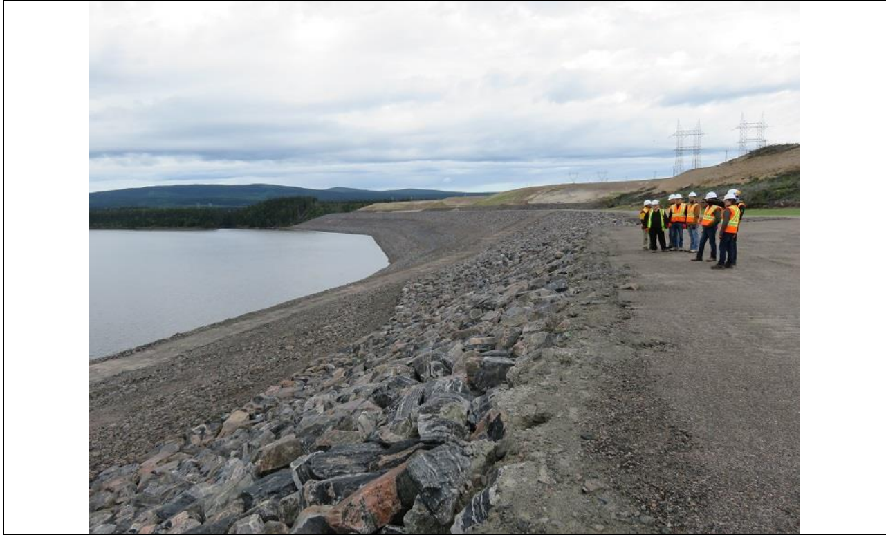
Photo E.1: Northerly view along upstream side of North Spur slope stabilization works. Group is standing on maintenance road at El. 43 m.
