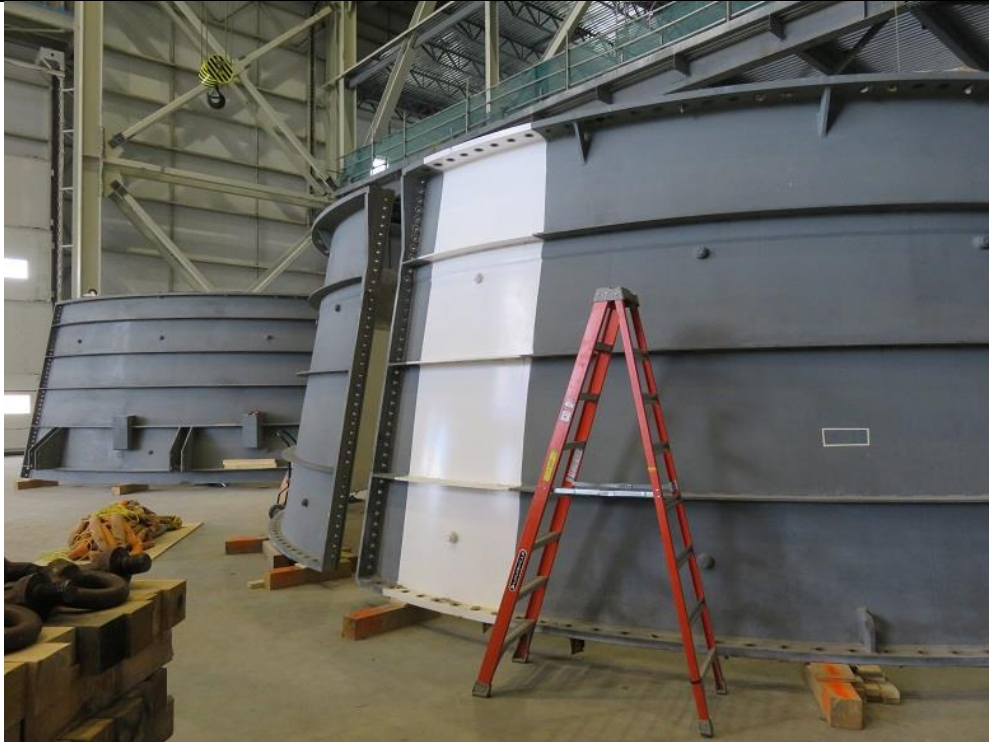
Photo A.11: Unit 1 draft tube liner segments being assembled in South Service Bay.
