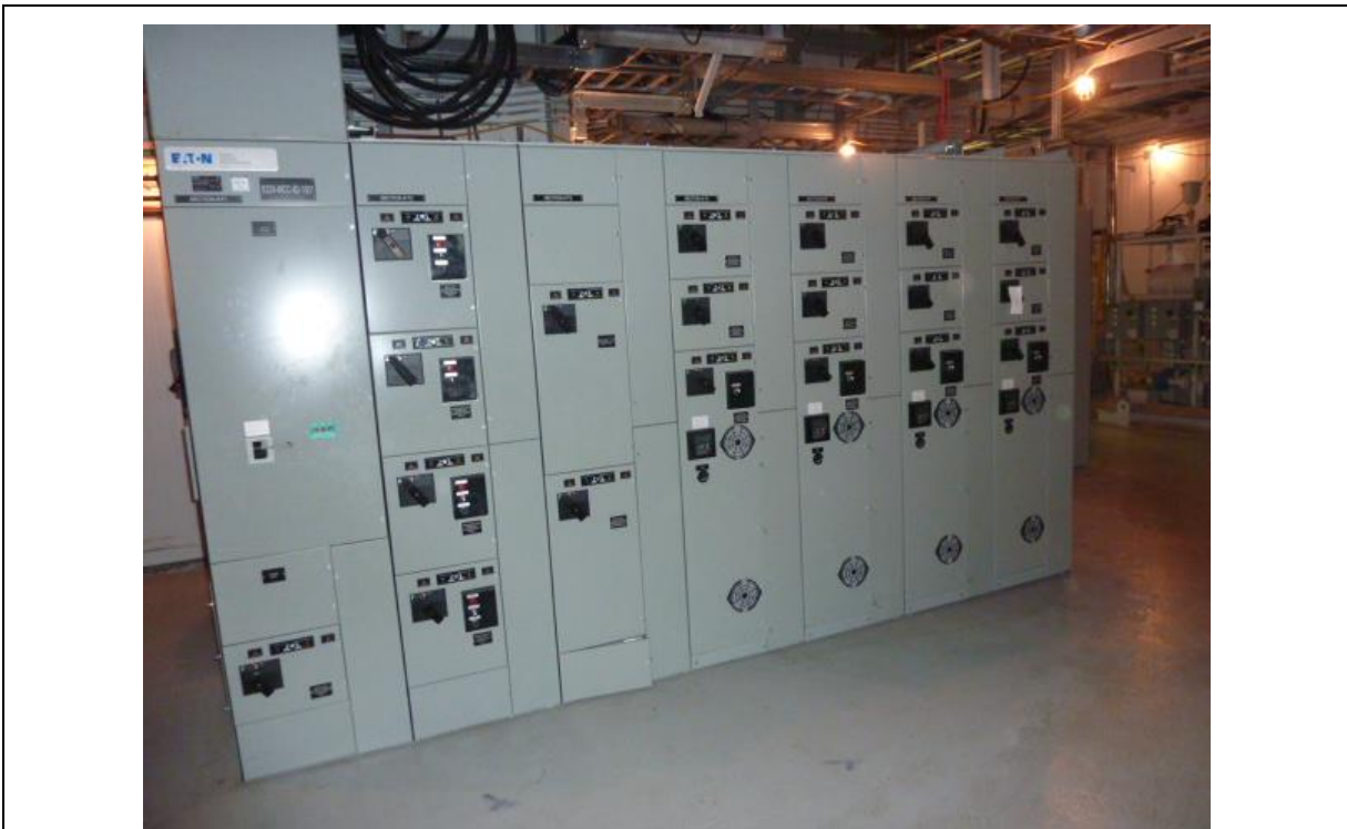
Photo H.6: Converter Station Valve Cooling - Motor Control Centre.
