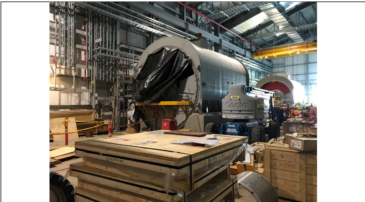
Photo H.16: Synchronous Condensers Units 2 and 3 installed on their pedestals.
