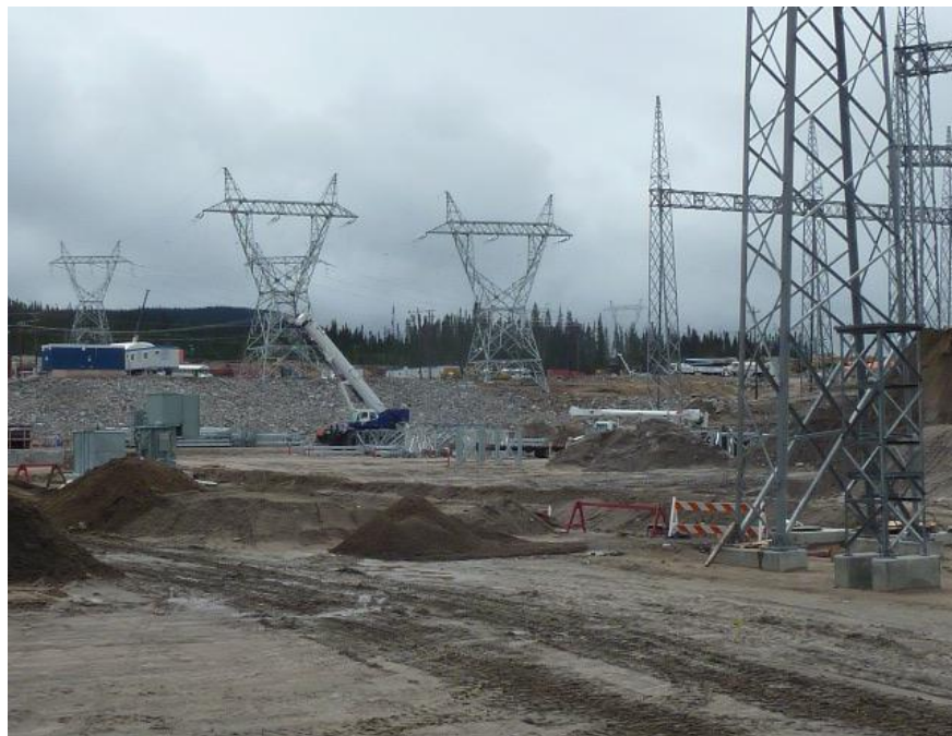
Photo F.4: Incoming Churchill Falls 315 kV AC Transmission Lines
