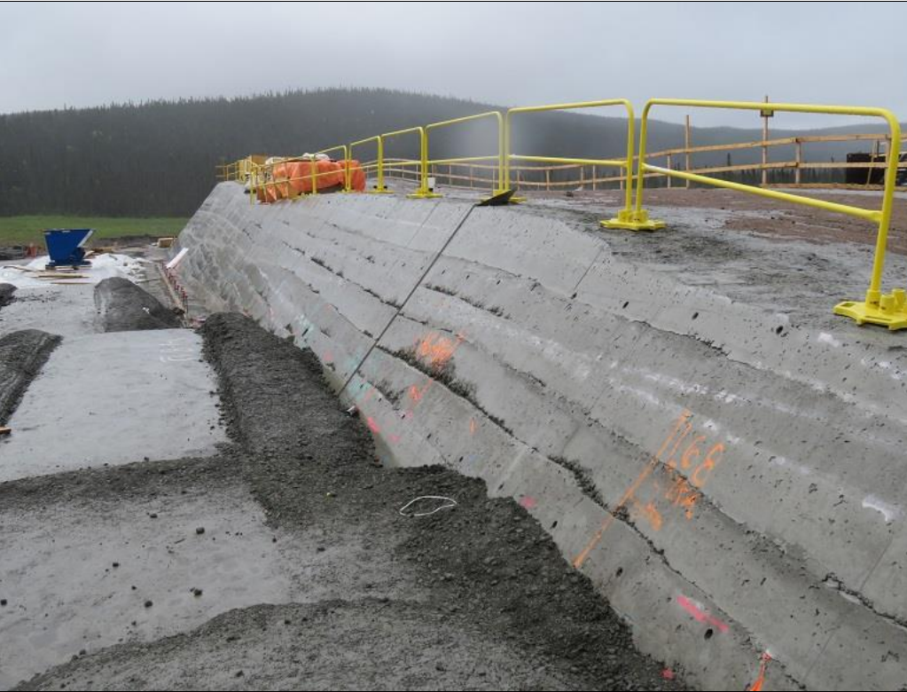
Photo C.10: Initial 2016 RCC trial placement, showing poor bonding along horizontal lift joints and honeycombing due to insufficient compaction at downstream sloping face.
