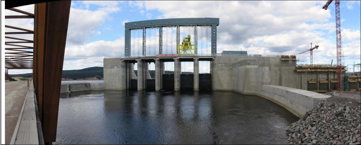
Photo B.1: Panoramic view of upstream side of spillway structure and approach channel, viewed from south end of temporary access bridge.
