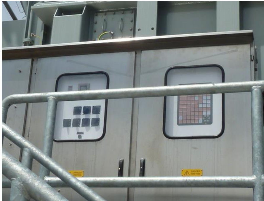
Photo H.10: Converter transformer annunciator and control panel detail.
