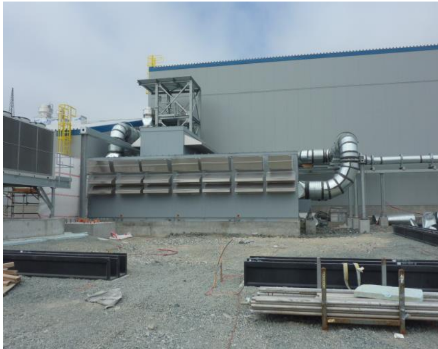
Photo H.3: Converter Station Cooling Equipment – Heat Exchangers.
