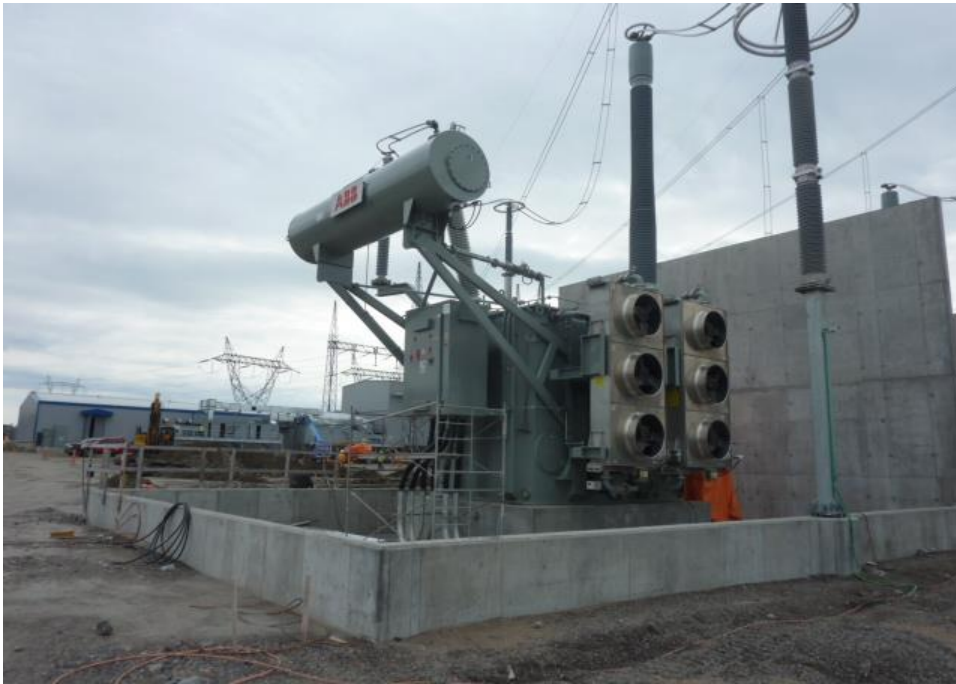
Photo G.1: CF Single Phase Transformer
