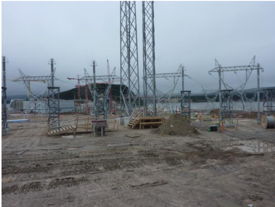
Photo F.3: Powerhouse to GIS building collector feeder lines
