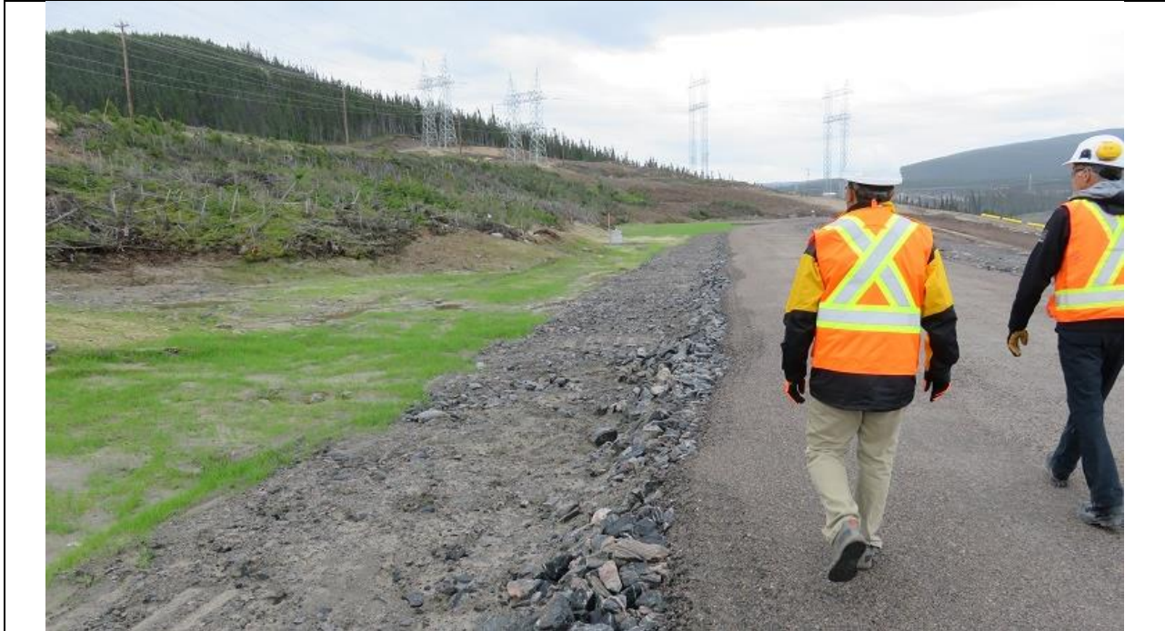
Photo E.3: Southerly view along maintenance road on upstream side of North Spur slope stabilization works. The top of the till blanket is just below the recently-seeded ditch on the inside of the road.
