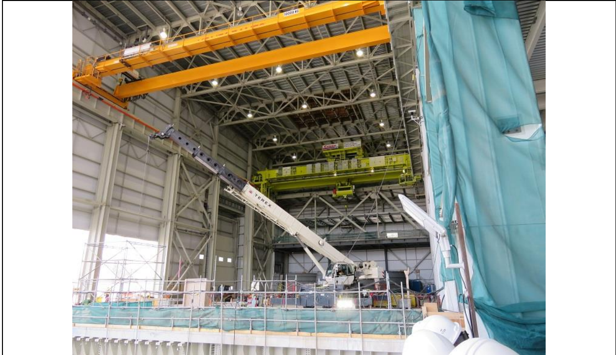
Photo A.5: South Service Bay, with overhead cranes commissioned in June 2017: 10,000 kg (orange) and 200 MT (green) capacities.
