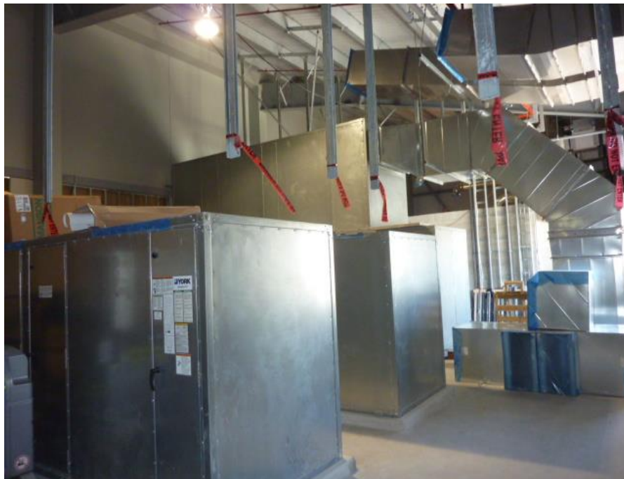
Photo H.4: Converter Station Valve Cooling - Interior Ducting.
