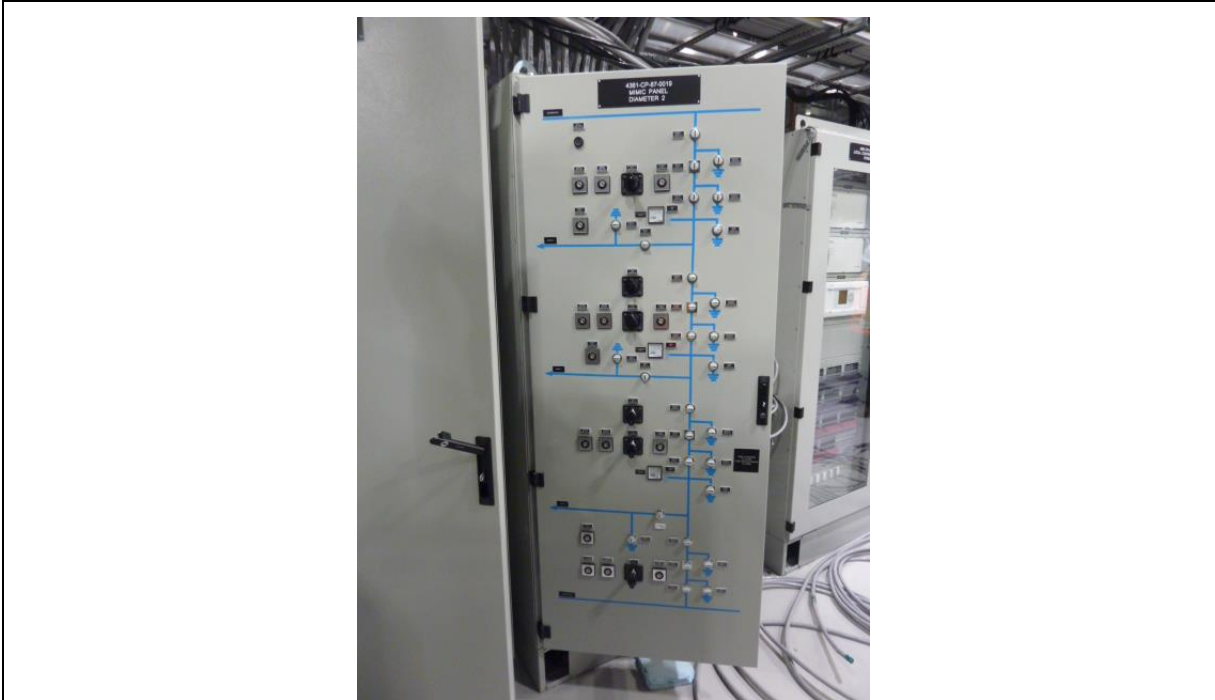
Photo F.9: GIS Equipment - Local Control Cabinets.
