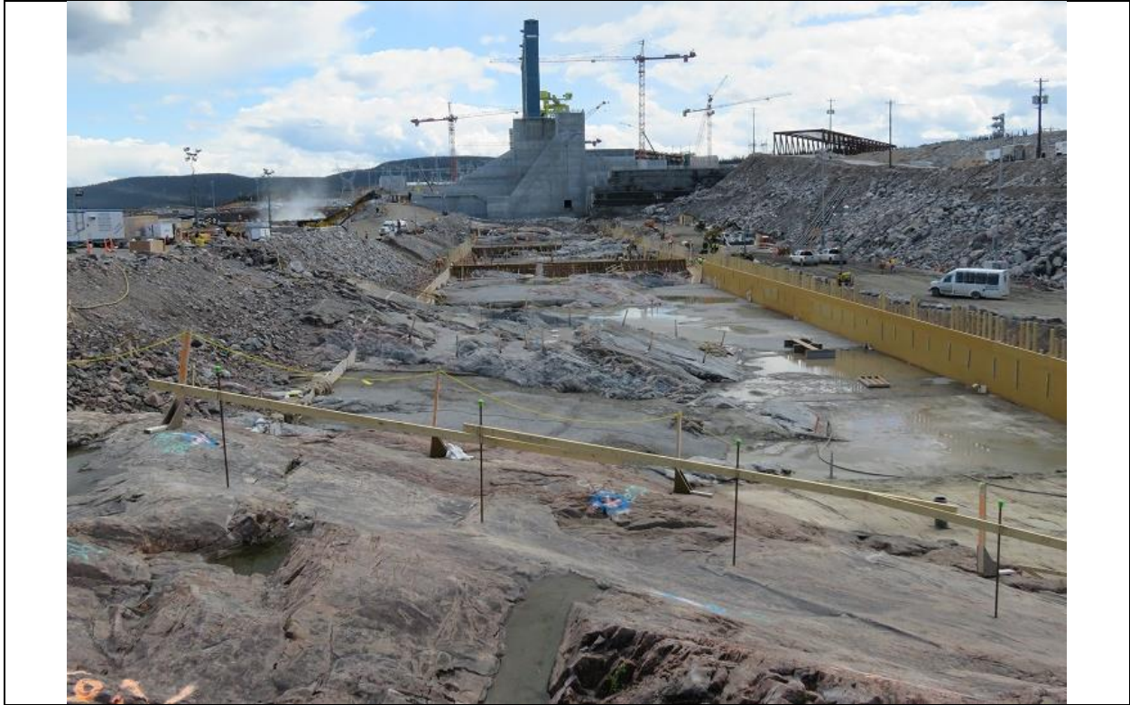
Photo C.3: Southerly view along RCC dam foundation, between downstream (left) and upstream (right) cofferdams. Formwork along sides indicates extent of dam footprint. Cast-in-place leveling concrete has been placed along upstream side.
