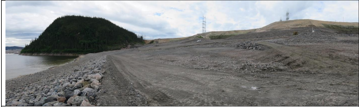
Photo E.5: Southerly panorama view along downstream side of North Spur slope stabilization works.
