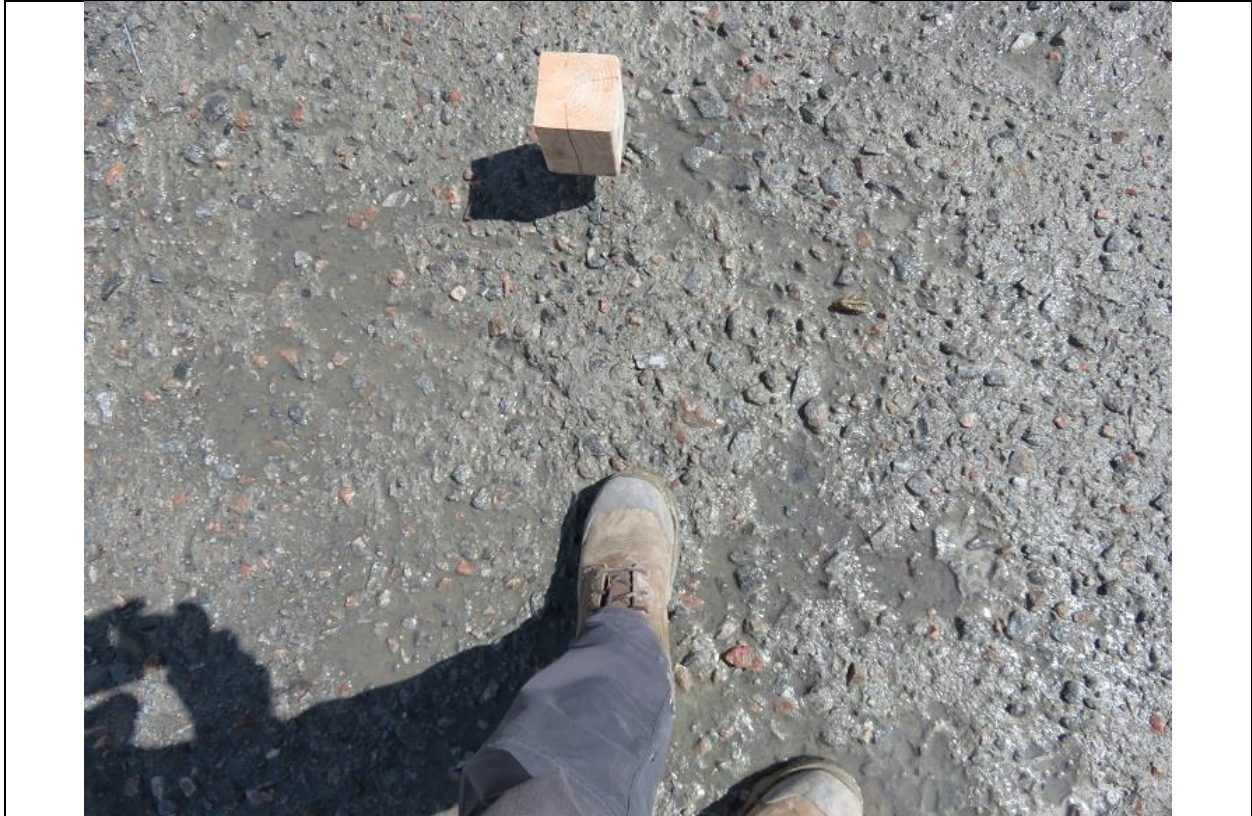
Photo C.7: Surface of leveling concrete slab after green cutting, which removes laitance and leaves exposed aggregate to provide a good bonding surface for the next layer of concrete or RCC.
