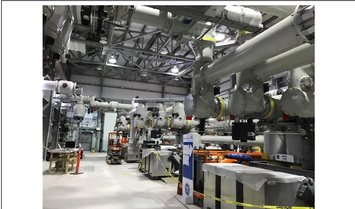
Photo G.5: CF GIS equipment installed. Cable terminations ongoing.
