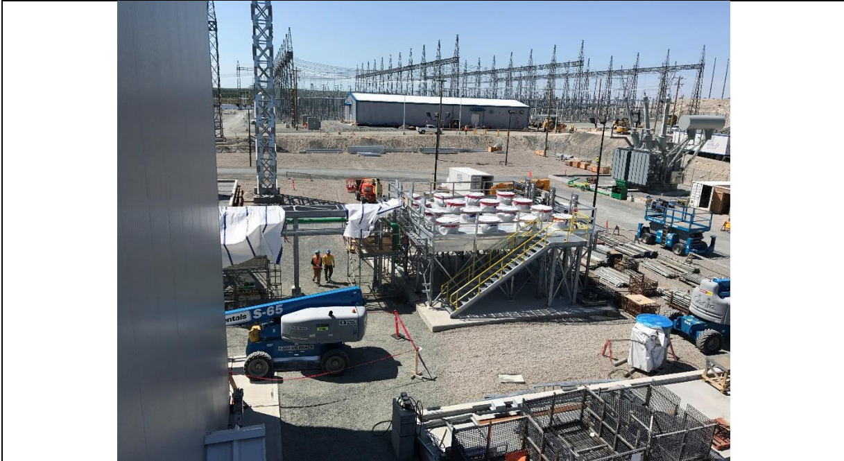
Photo H.17: Synchronous Condensers Cooling System - exterior heat exchangers
