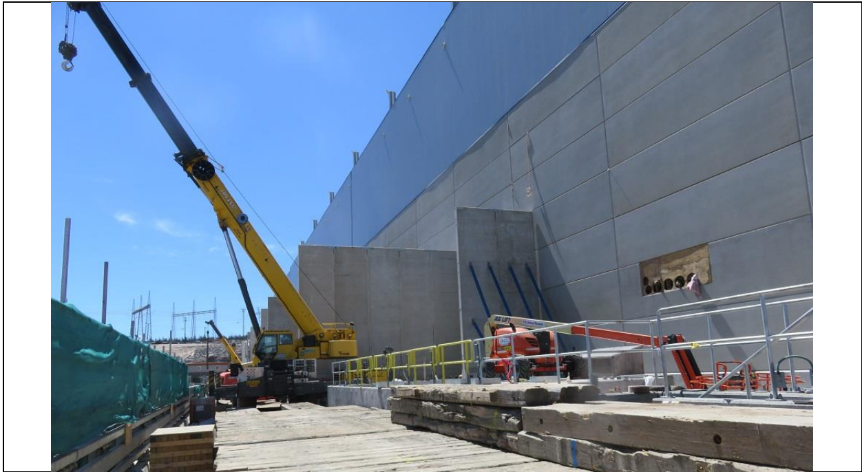
Photo B.9: Transformer bays on tailrace deck.
