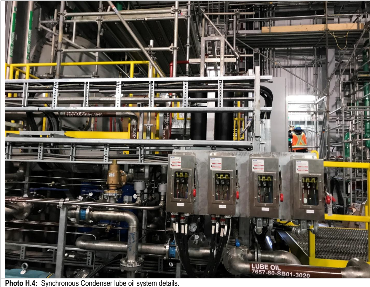
Photo H.4: Synchronous Condenser lube oil system details.
