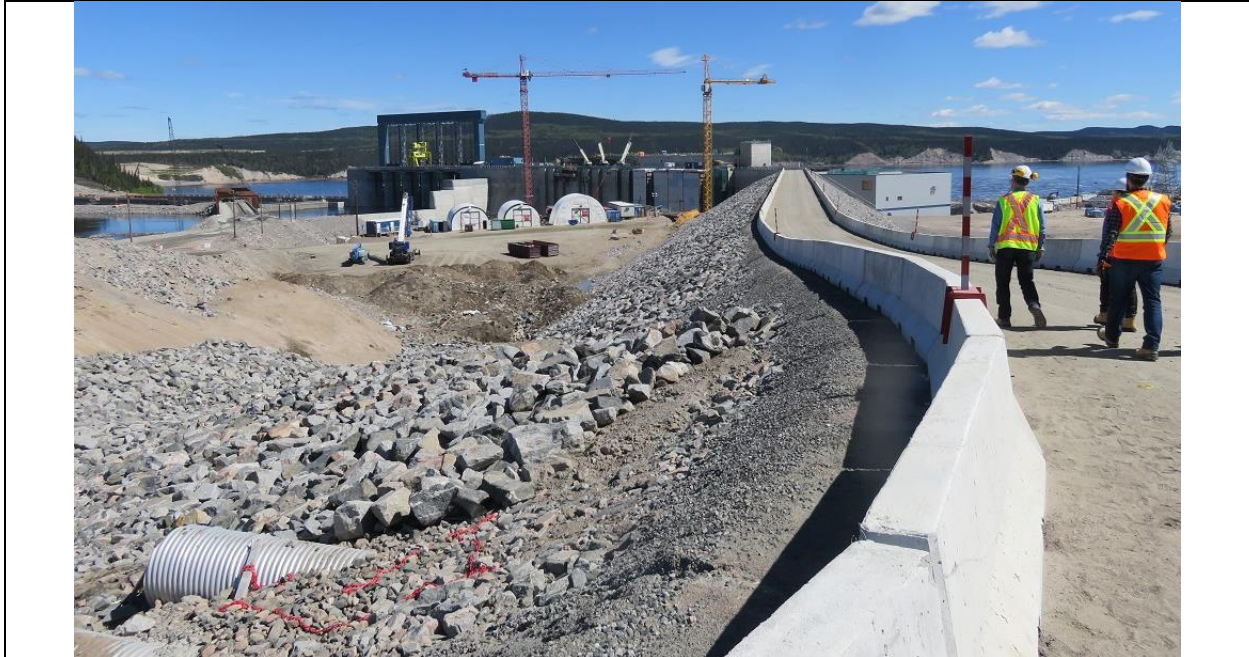
Photo E.1: Upstream side of south embankment dam, with spillway and intakes in background at left.
