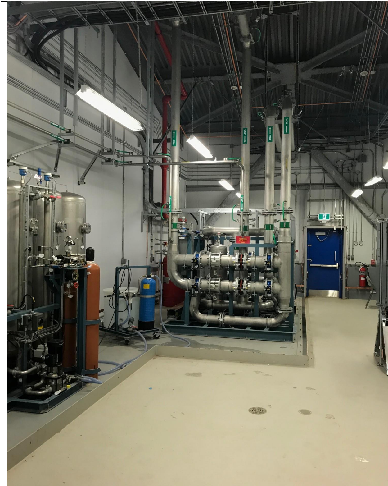
Photo H.2: Converter Station - Valve cooling system.
