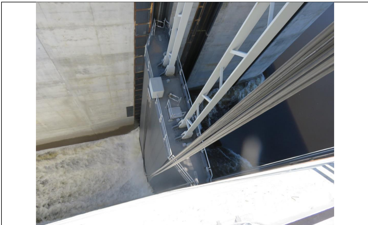
Photo C.2: Looking down at partially-open spillway service gate. Flow is right to left.
