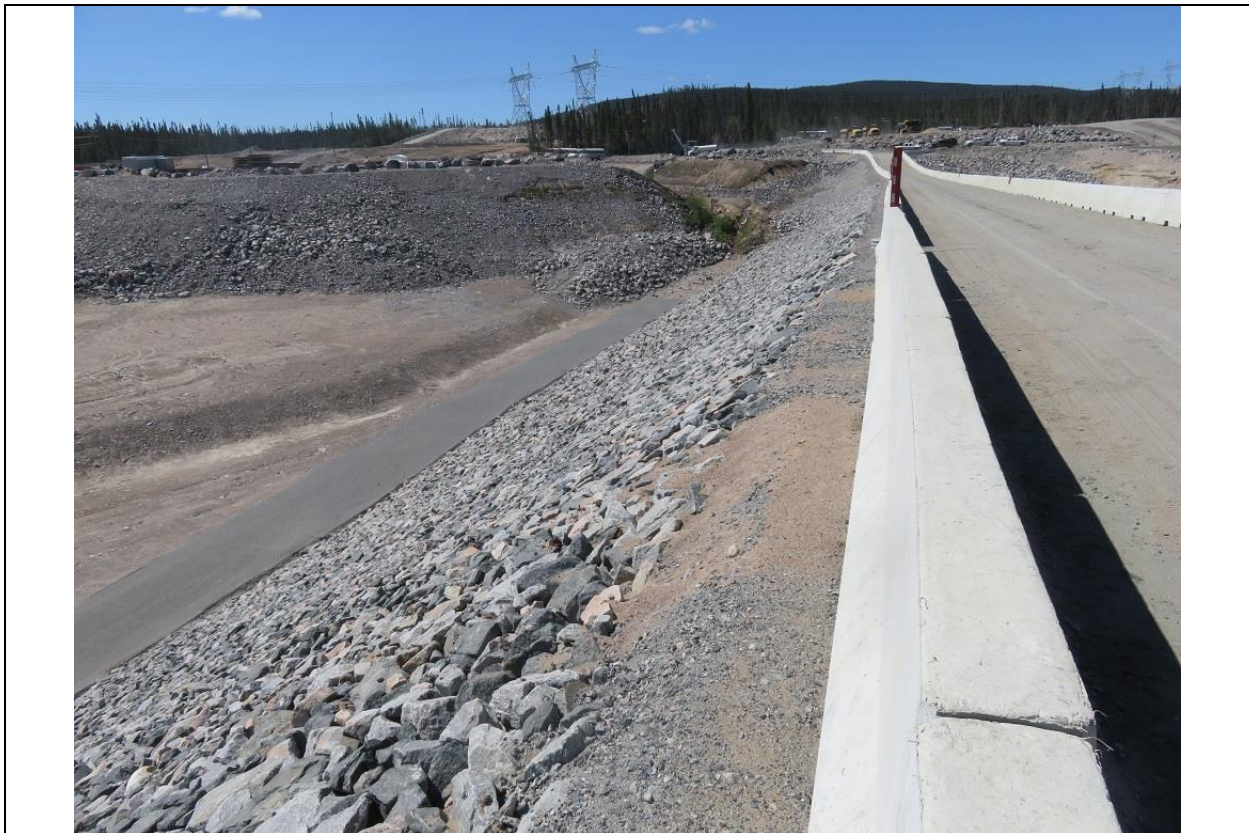
Photo E.2: Southerly view along downstream side of south embankment showing neatly-finished riprap cover.
