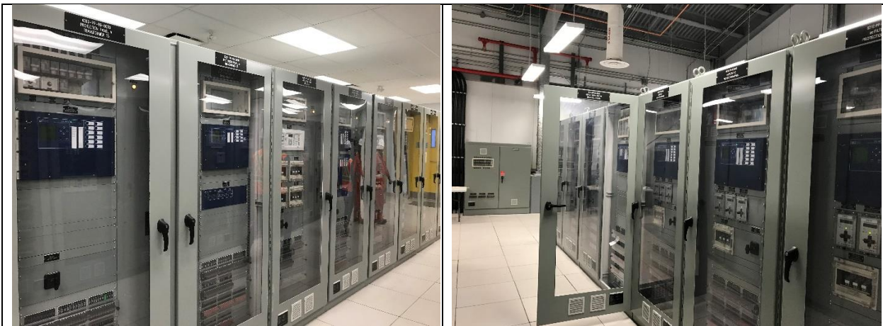
Photo G.6: Muskrat Falls Converter Station - protection panels
