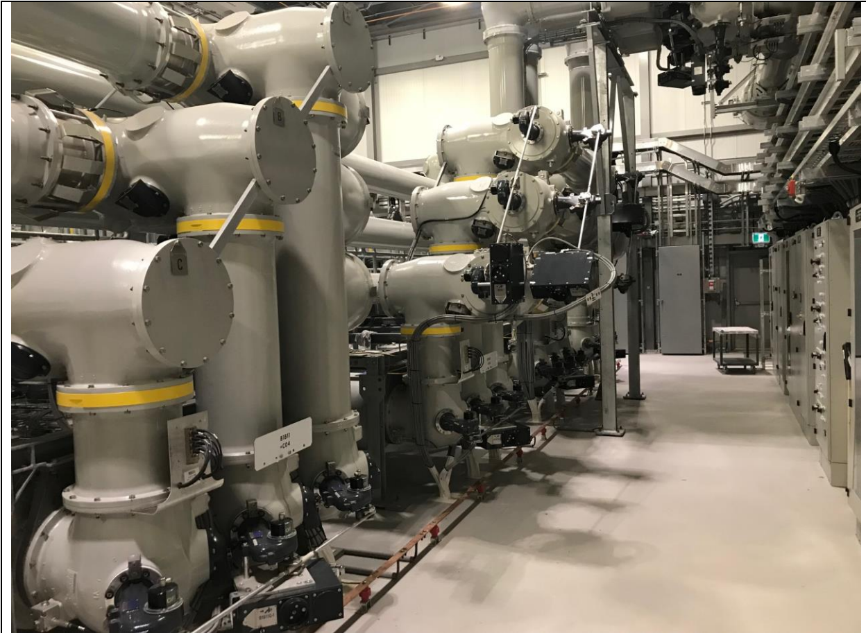
Photo G.1: Muskrat Falls -.GIS equipment energized.
