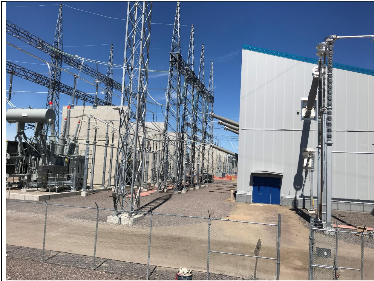
Photo G.3: Converter Station Transformers – fully dressed with Pole 1 (on the opposite side) energized.
