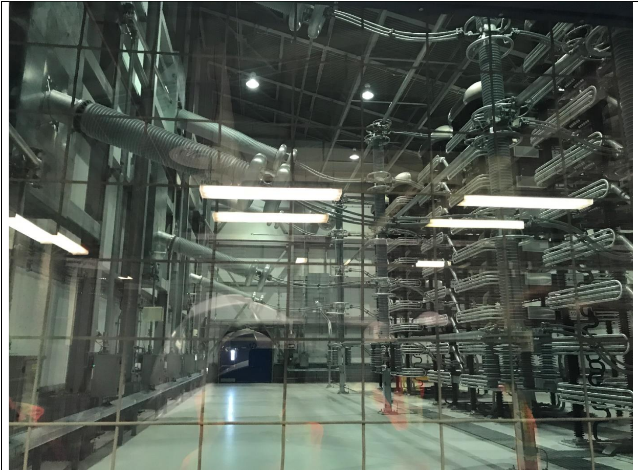
Photo G.5: Muskrat Falls – Converter Valve 1 energized.
