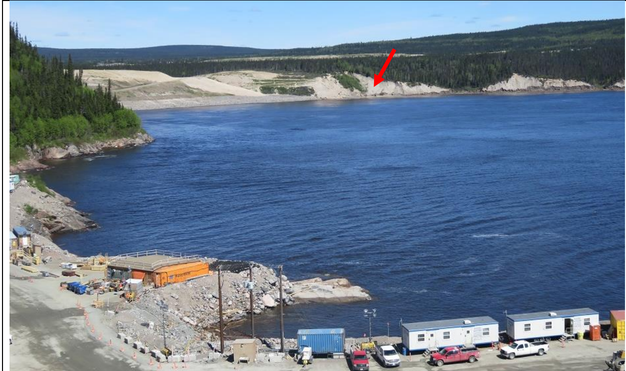
Photo F.1: North river bank downstream of North Spur. Arrow indicates approximate location of local surficial slide reported in early February 2018, within a pre-existing erosional slope. Dark area just above river level to downstream indicates extent of ongoing recent erosion along toe of other similar slopes.
