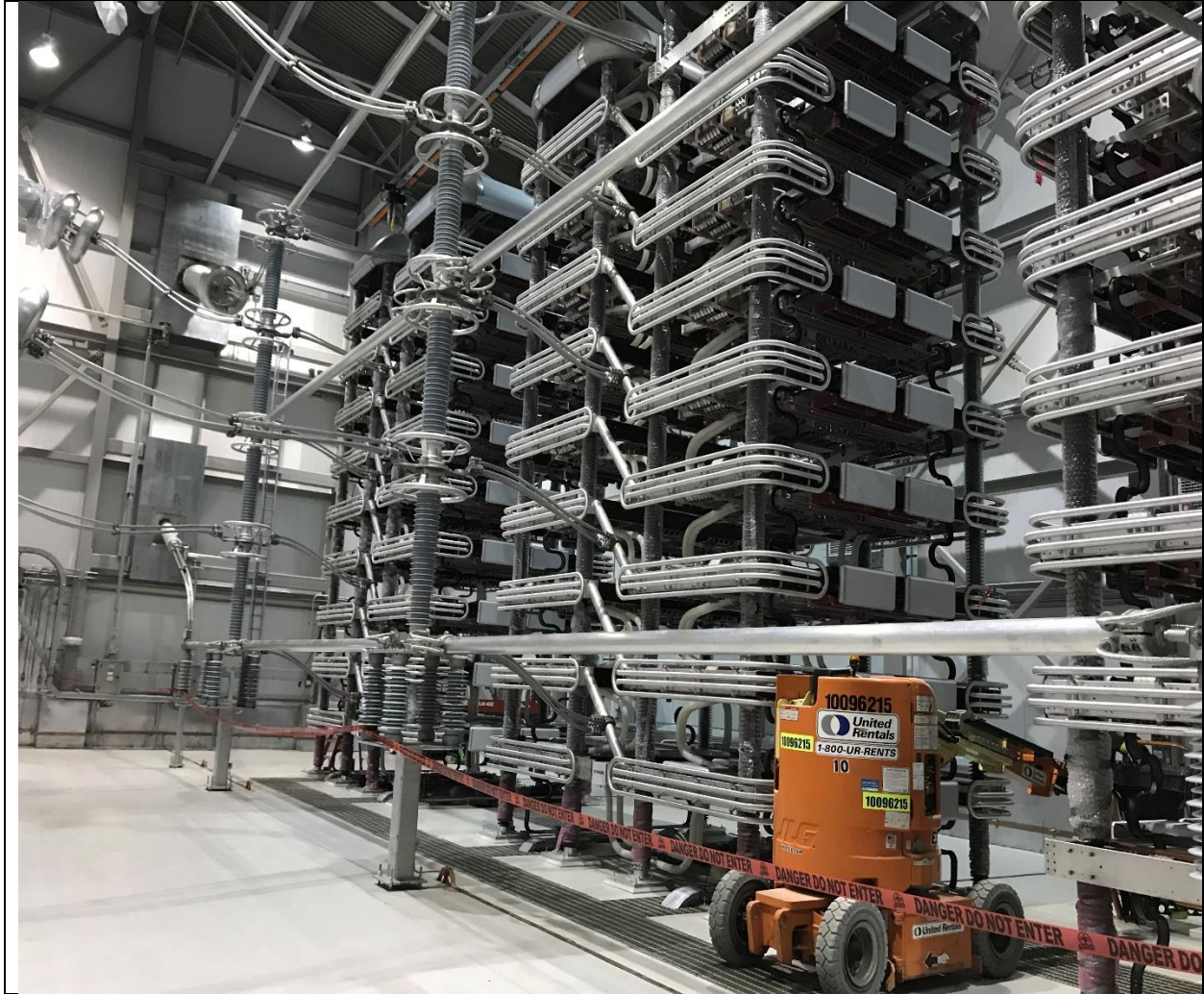
Photo H.1: Converter Station - Valve hall 2.
