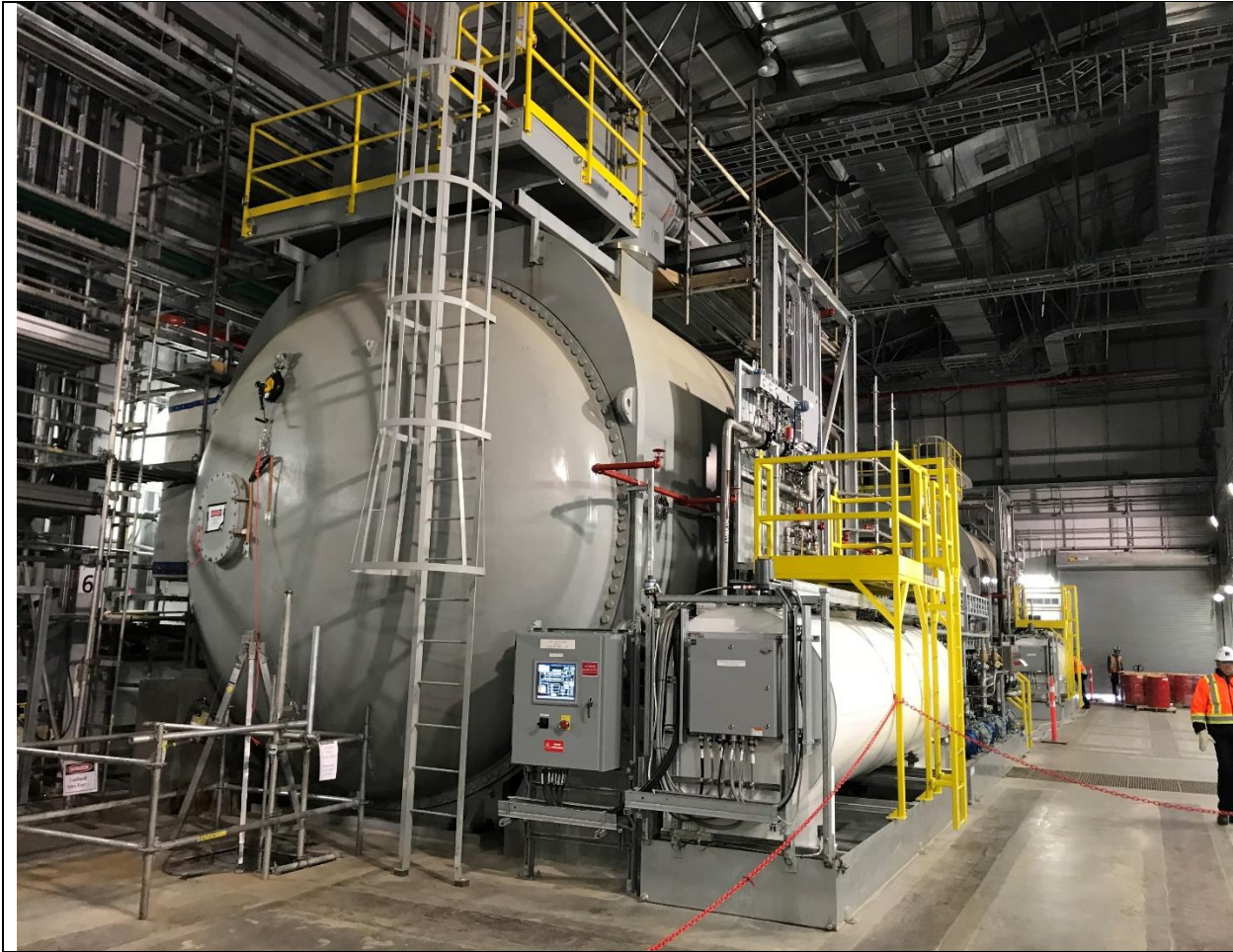
Photo H.3: Synchronous Condensers.
