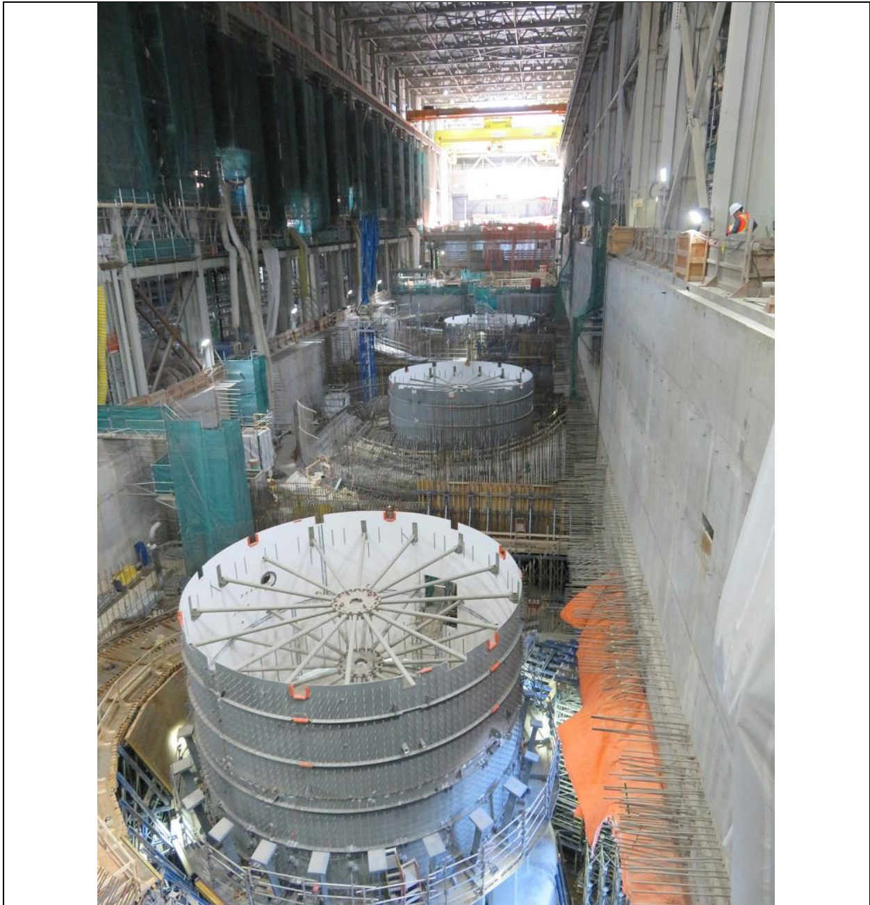
Photo B.3: Interior view of powerhouse from North Service Bay (generator floor level), with Unit 4 in foreground.
