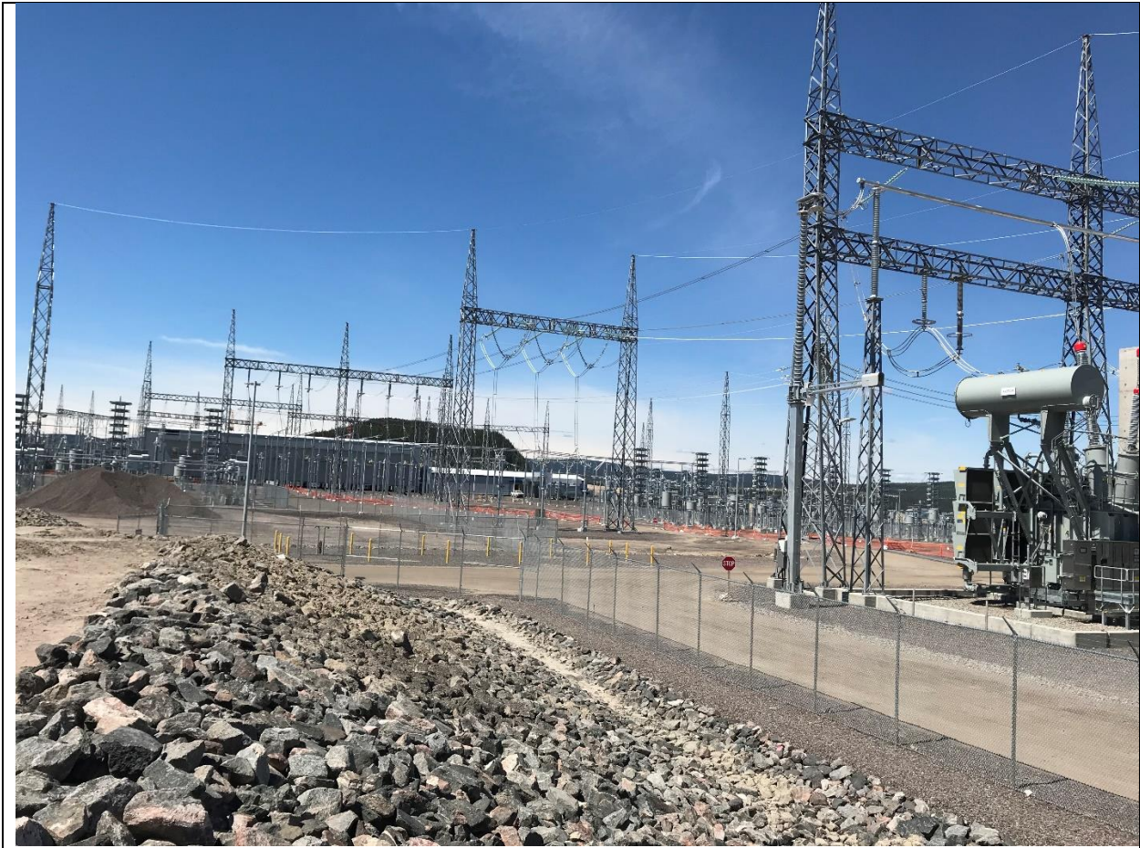
Photo G 2: AC Switchyard with GIC and Control buildings on the background.
