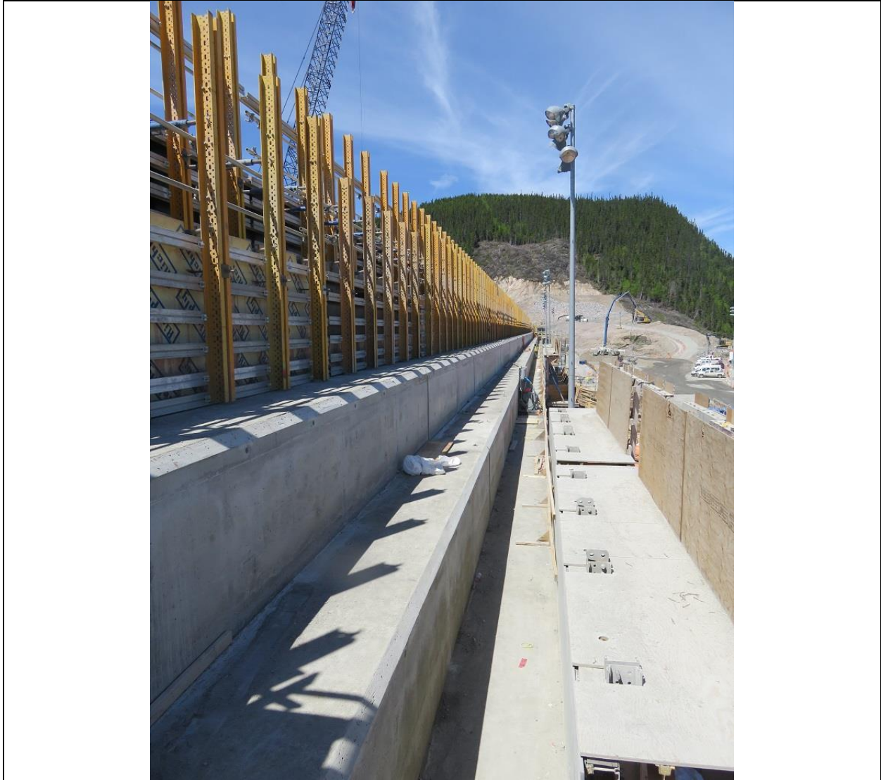
Photo D.4: Stepped downstream side of RCC dam, constructed with RCC and facial conventional concrete.
