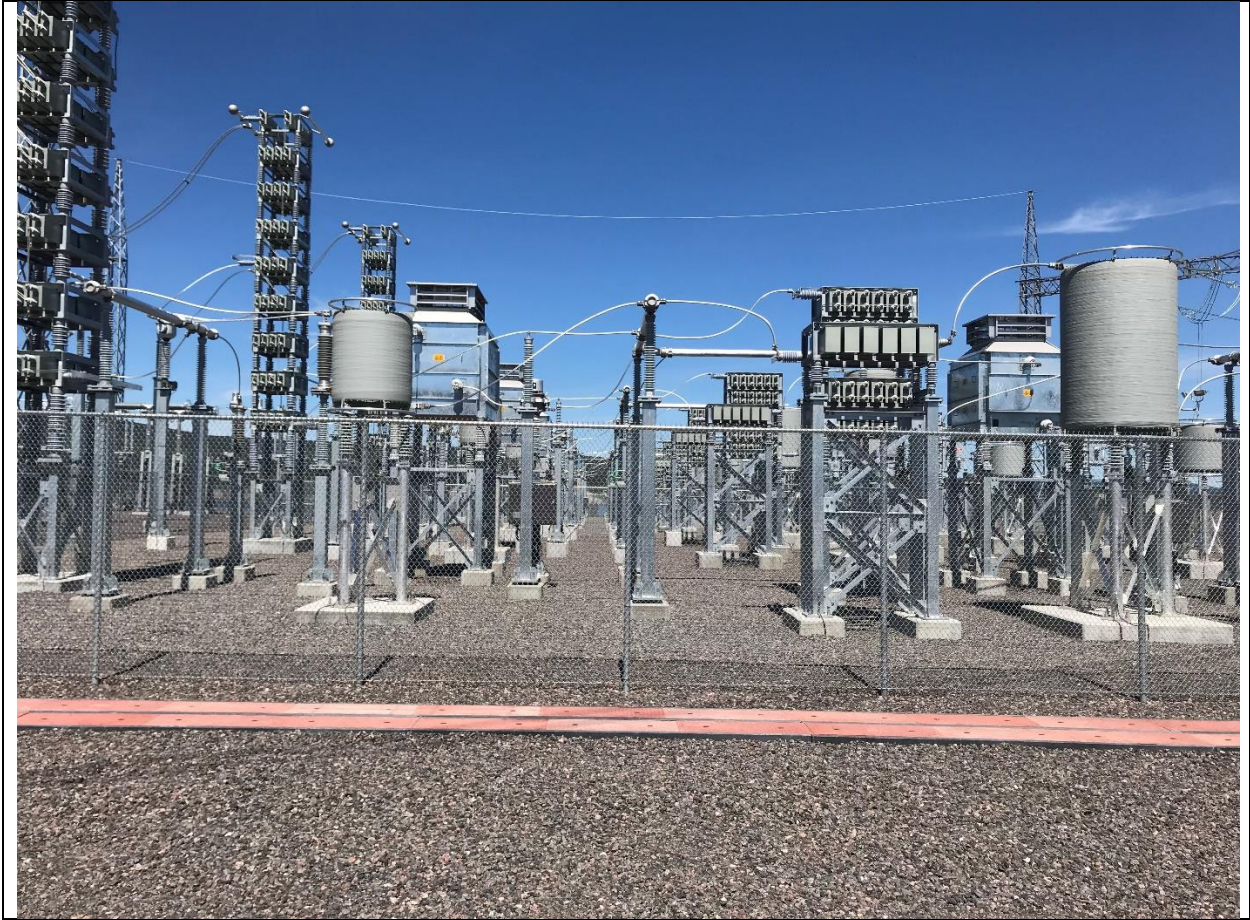
Photo G.4: Converter Station AC filters yard.
