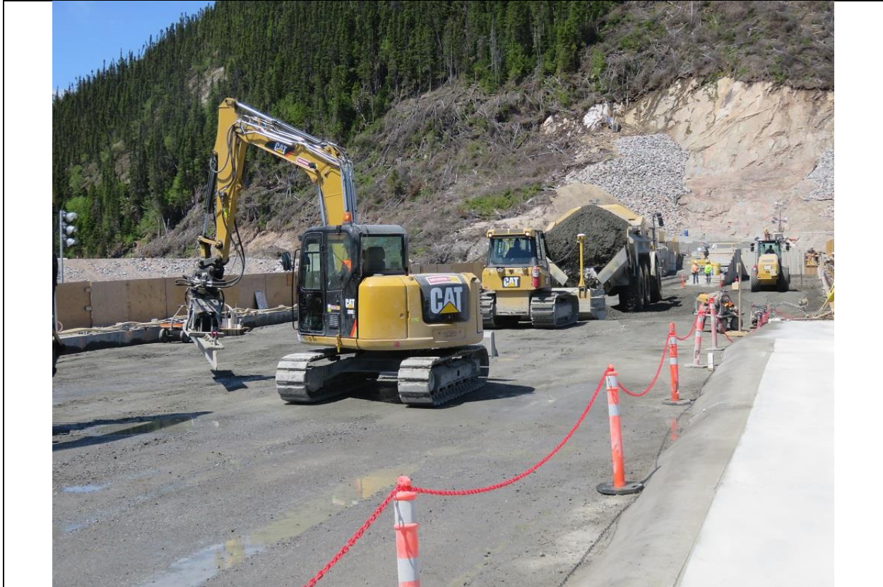
Photo D.2: RCC placement in progress at north end of RCC dam. Smooth concrete at right is conventional concrete that forms one of the steps on the downstream side of the dam.
