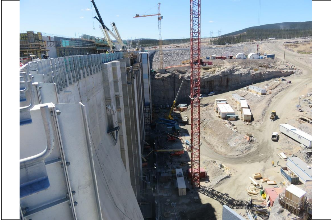
Photo B.1: Power intakes and intake channel, with south embankment dam in background.
