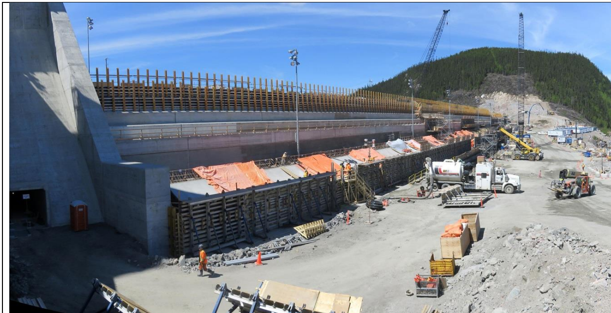
Photo D.3: Downstream side of RCC dam, with north transition dam at left.
