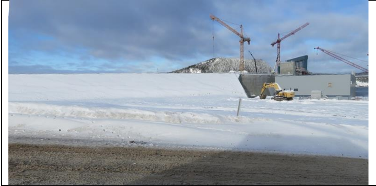
Photo E.3: Downstream side of south embankment dam and contact with south transition dam.
