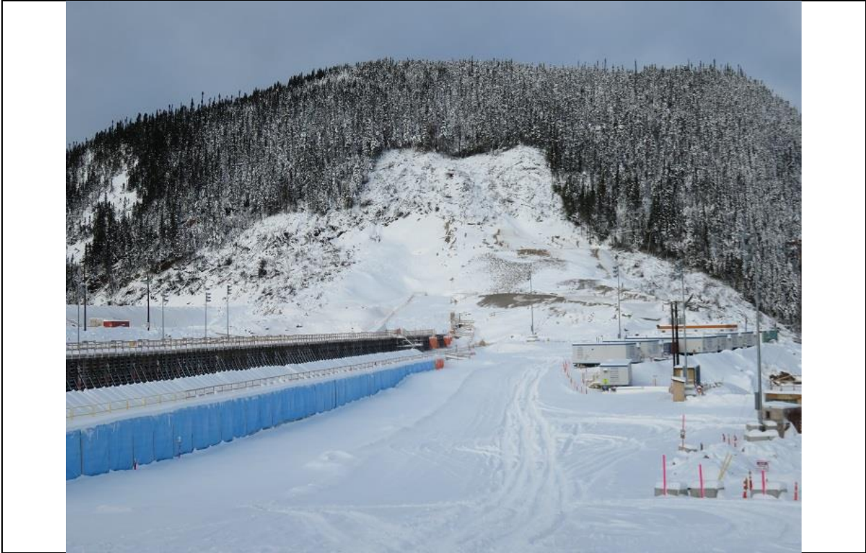
Photo D.3: Northerly view along downstream side of RCC dam. Formwork remains in place on the upper part of the dam and the lower part has been covered with blue tarps for winter insulation.
