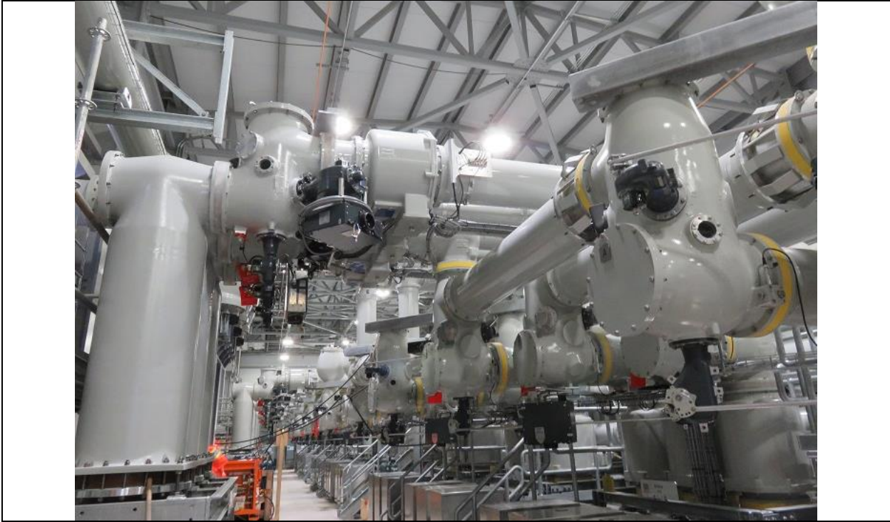
Photo F.5: GIS equipment.
