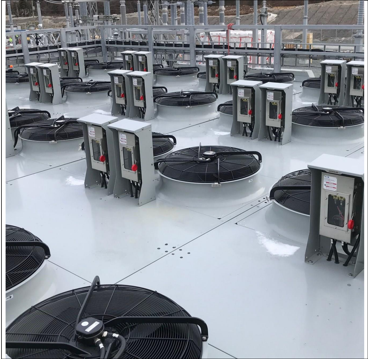
Photo G.4: Valve cooling heat exchangers.
