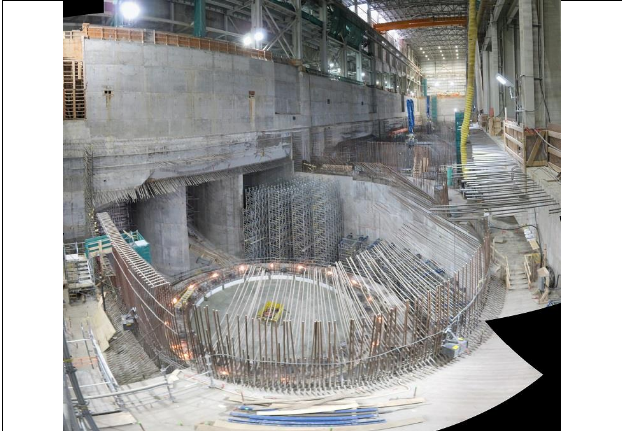
Photo B.3: Interior of powerhouse, with Unit 1 draft tube in foreground and Unit 1 intakes at centre left.
