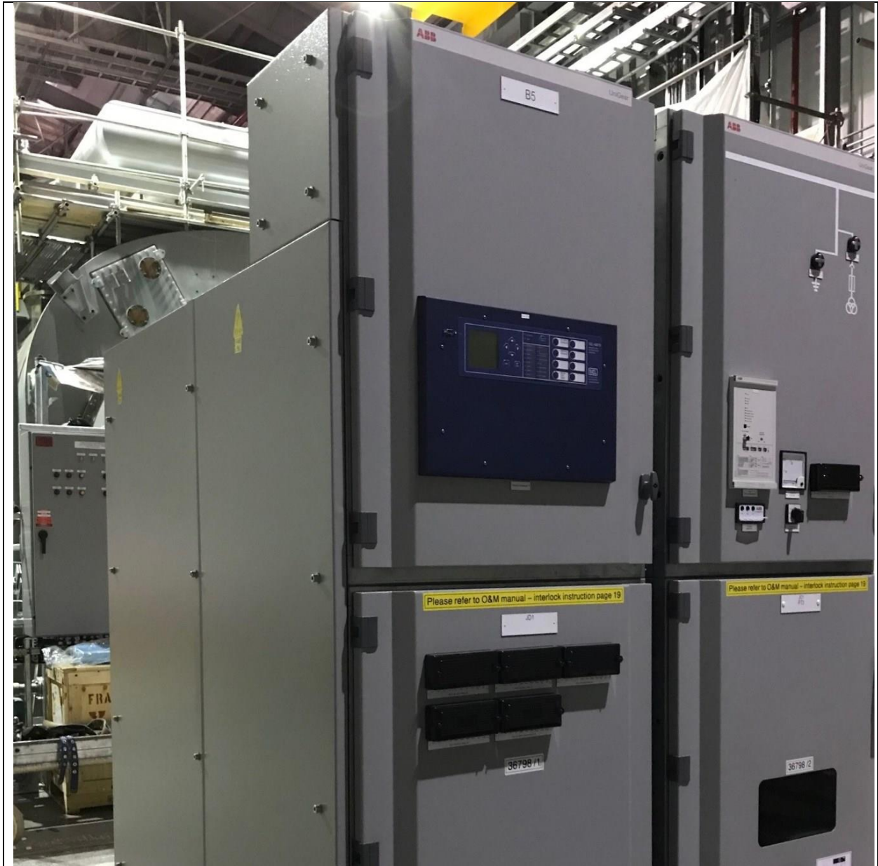
Photo G.6: Synchronous condenser control cabinets.
