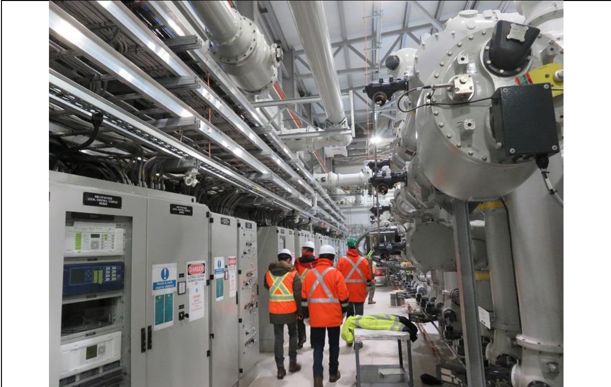
Photo F.6: GIS equipment, cable trays and control cabinets.
