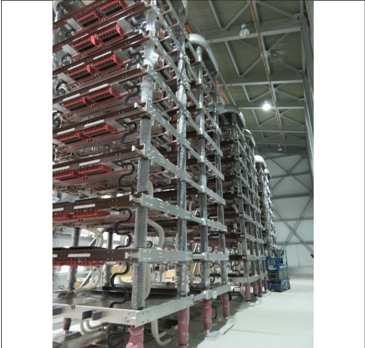
Photo G.3: Soldier's Pond converter building valve hall.
