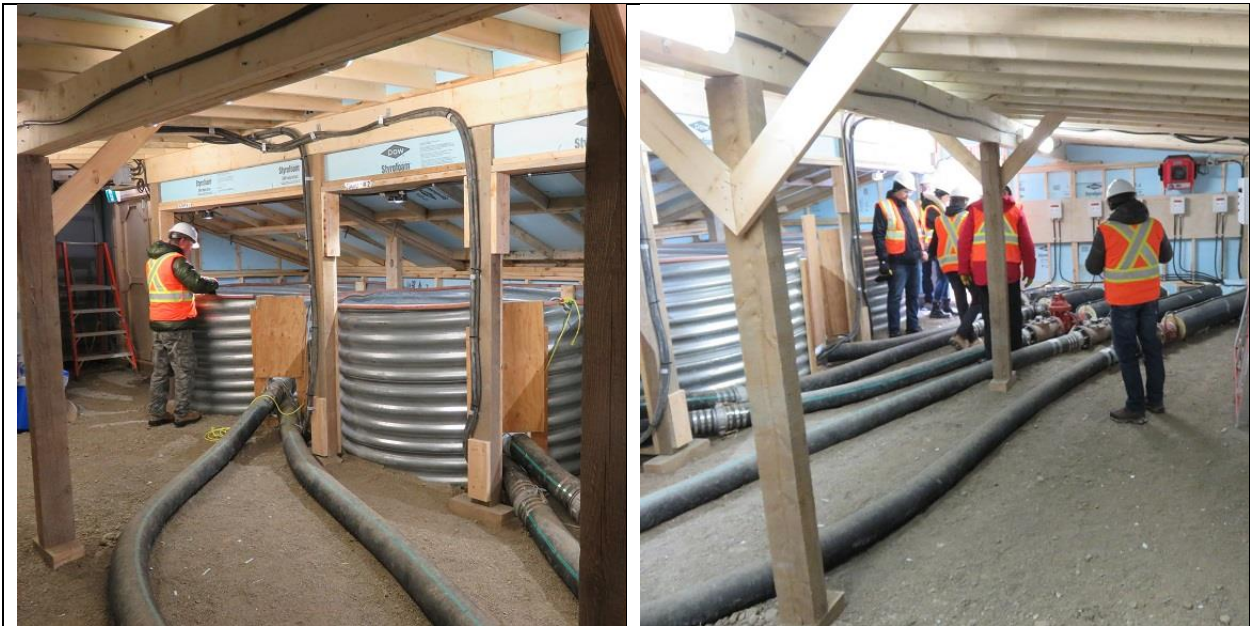
Photo D.4: Upstream cofferdam dewatering system housed inside insulated temporary structure. Inside each vertical corrugated metal pipe is a seepage collection sump with a pump. Pumped flows are measured by flow meters and returned to the reservoir.
