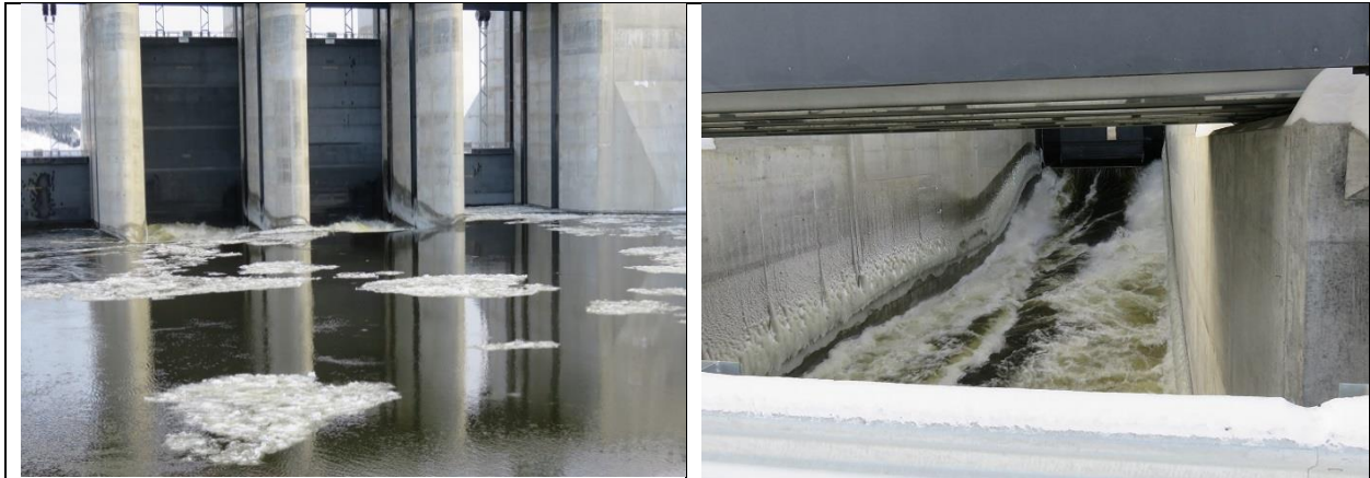
Photo C.3: Open spillway gates showing entrance flow conditions (left) and exit flow conditions (right).
