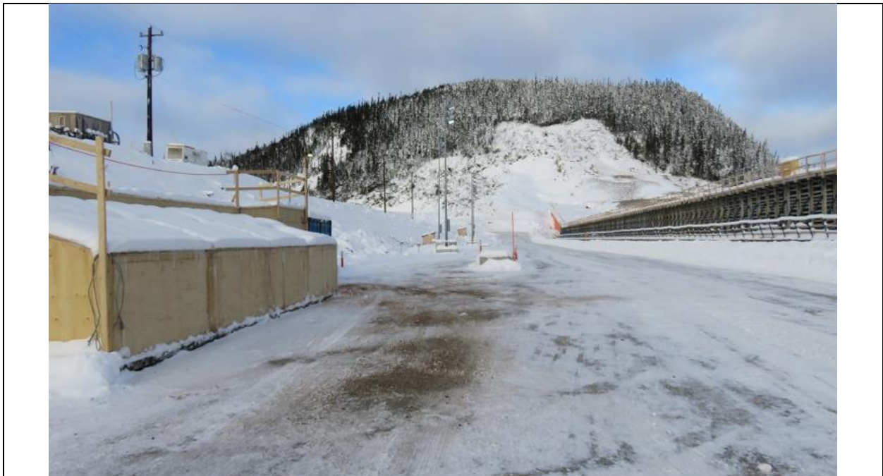
Photo D.2: Northerly view between upstream cofferdam (left) and RCC dam (right). Wooden structure at left houses the cofferdam dewatering system.
