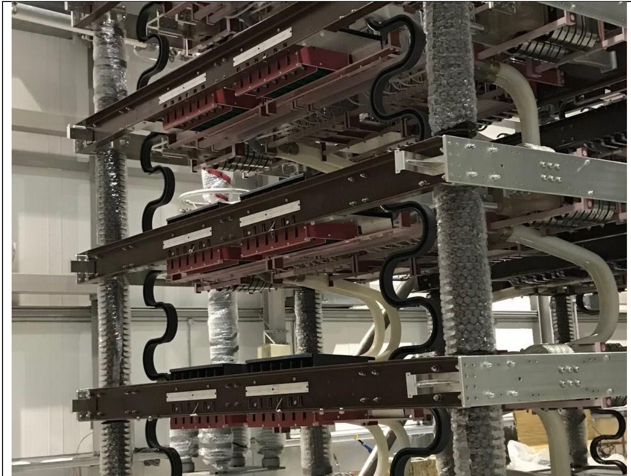
Photo F.4: Valve cooling detail.
