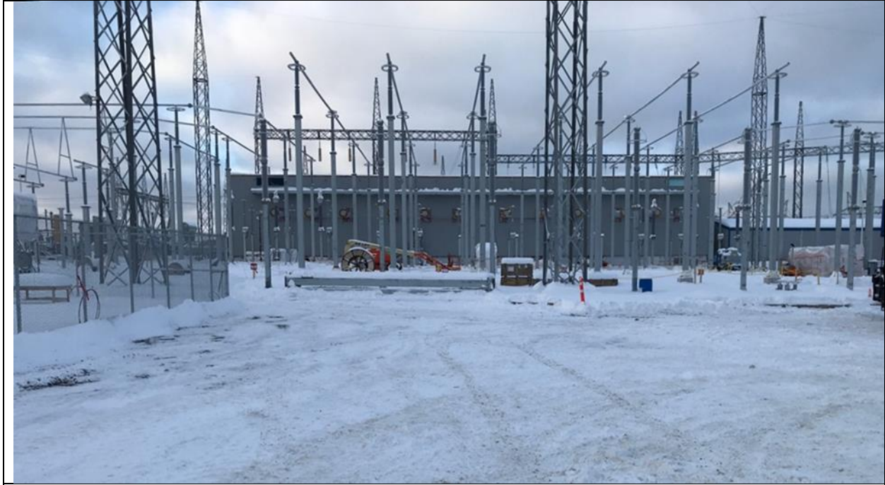
Photo F.1: Muskrat Falls DC switchyard.
