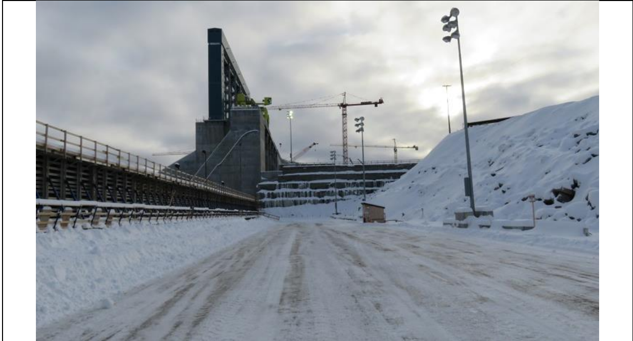
Photo D.1: Southerly view between RCC dam (left) and upstream cofferdam (right). RCC formwork is being left in place through the winter for insulation purposes.
