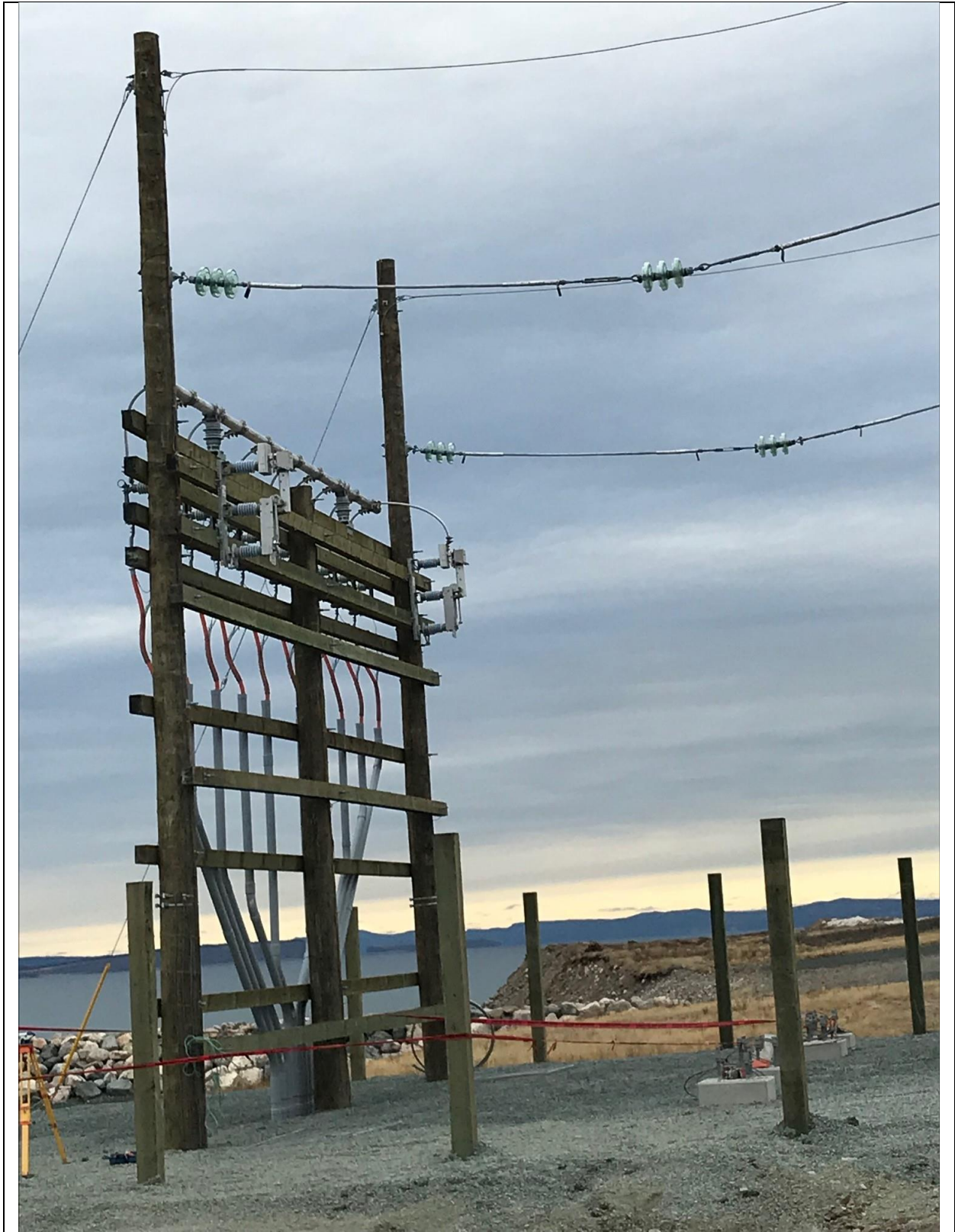
Photo H.2: Dowden's Point grounding lines terminations.
