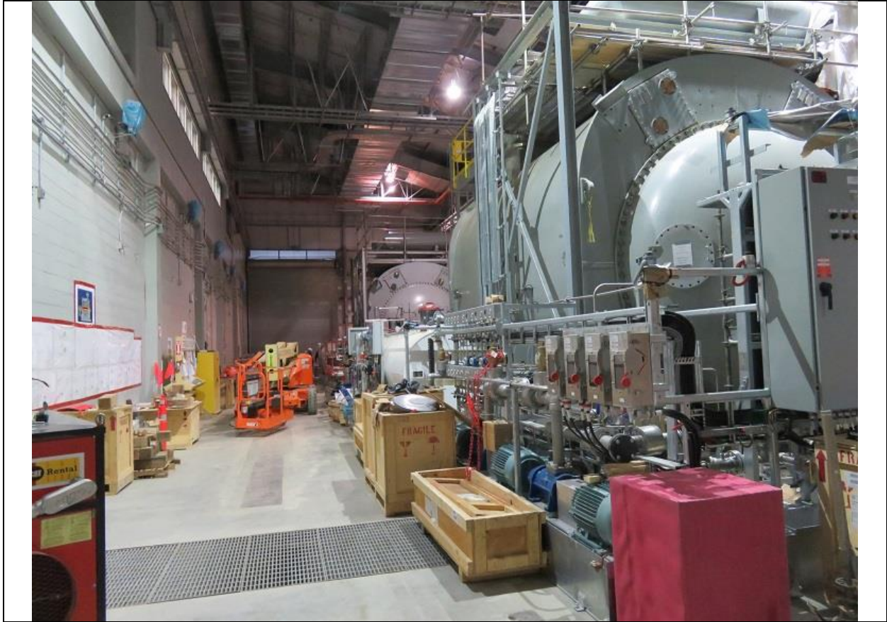
Photo G.5: Synchronous condensers.
