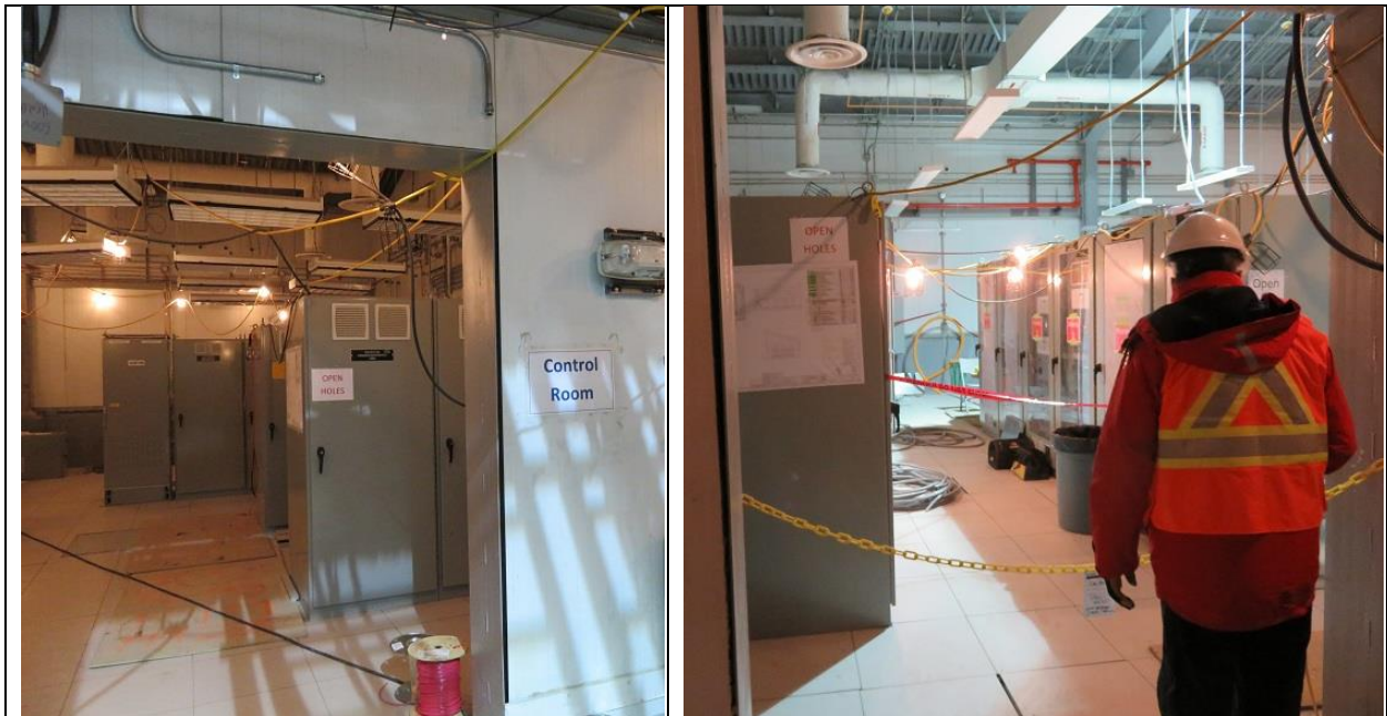
Photo F.2: Muskrat Falls converter building control room (left) and P&C room (right).
