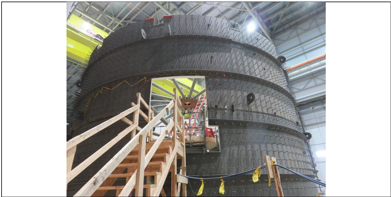
Photo B.6: Turbine pit liner with external Nelson stud anchors that will be embedded in second stage concrete.
