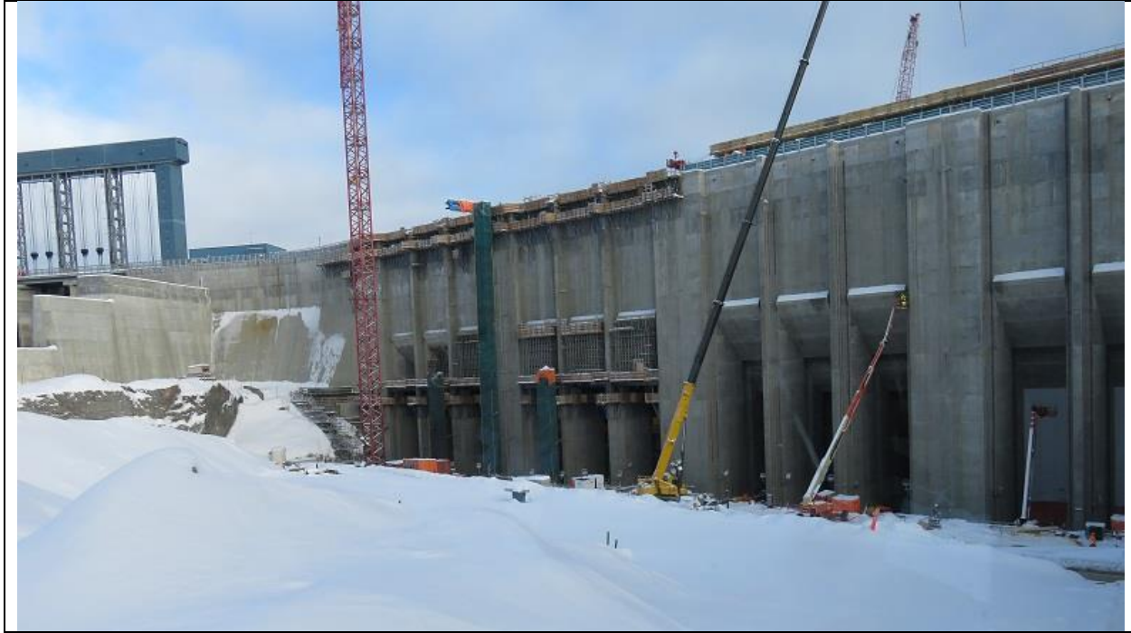
Photo B.1: Upstream side of power intake structure with Unit 4 intake at left (3 intake bays per unit).
