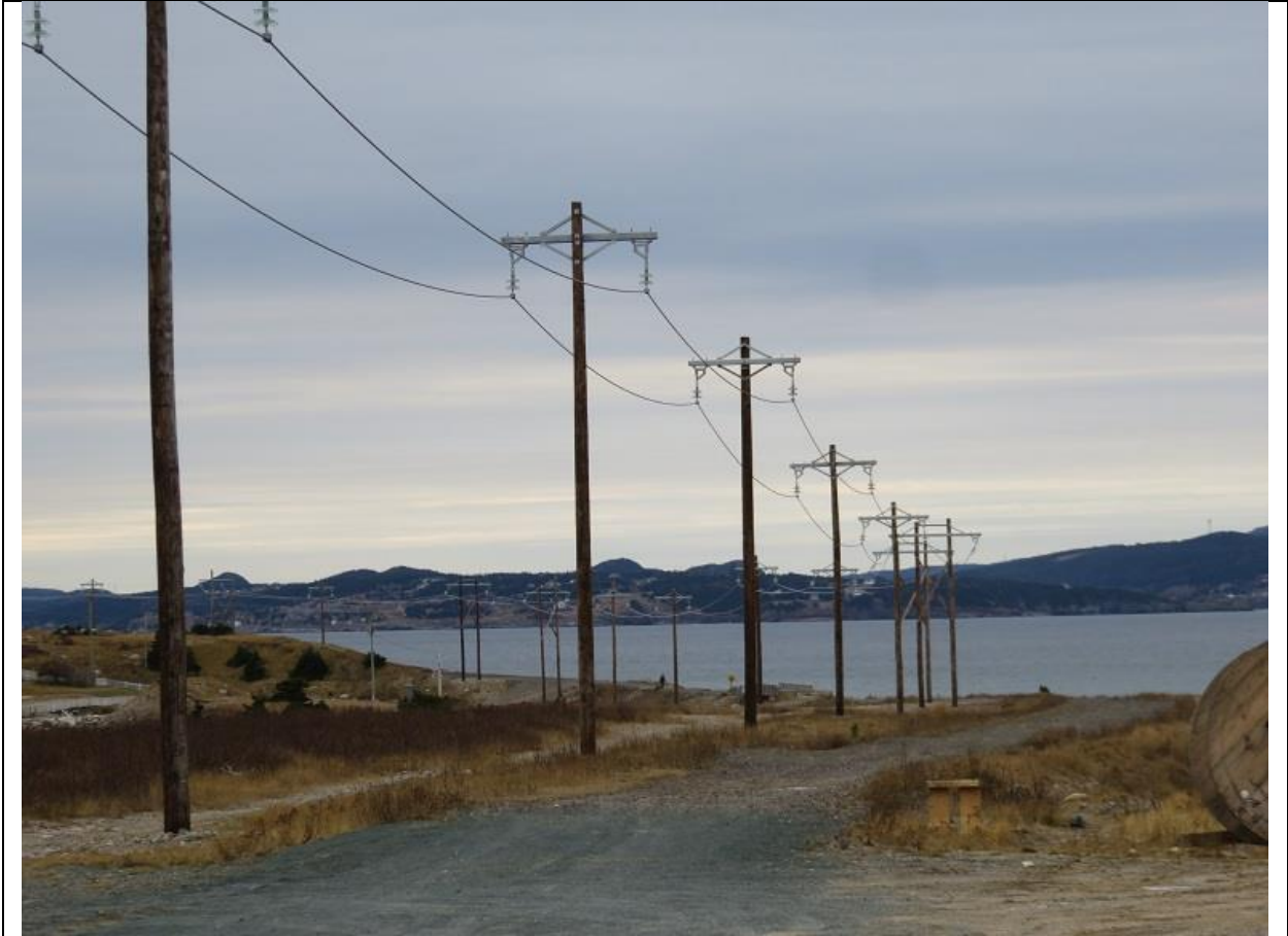
Photo H.1: Grounding line on west side of Dowden’s Point site.
