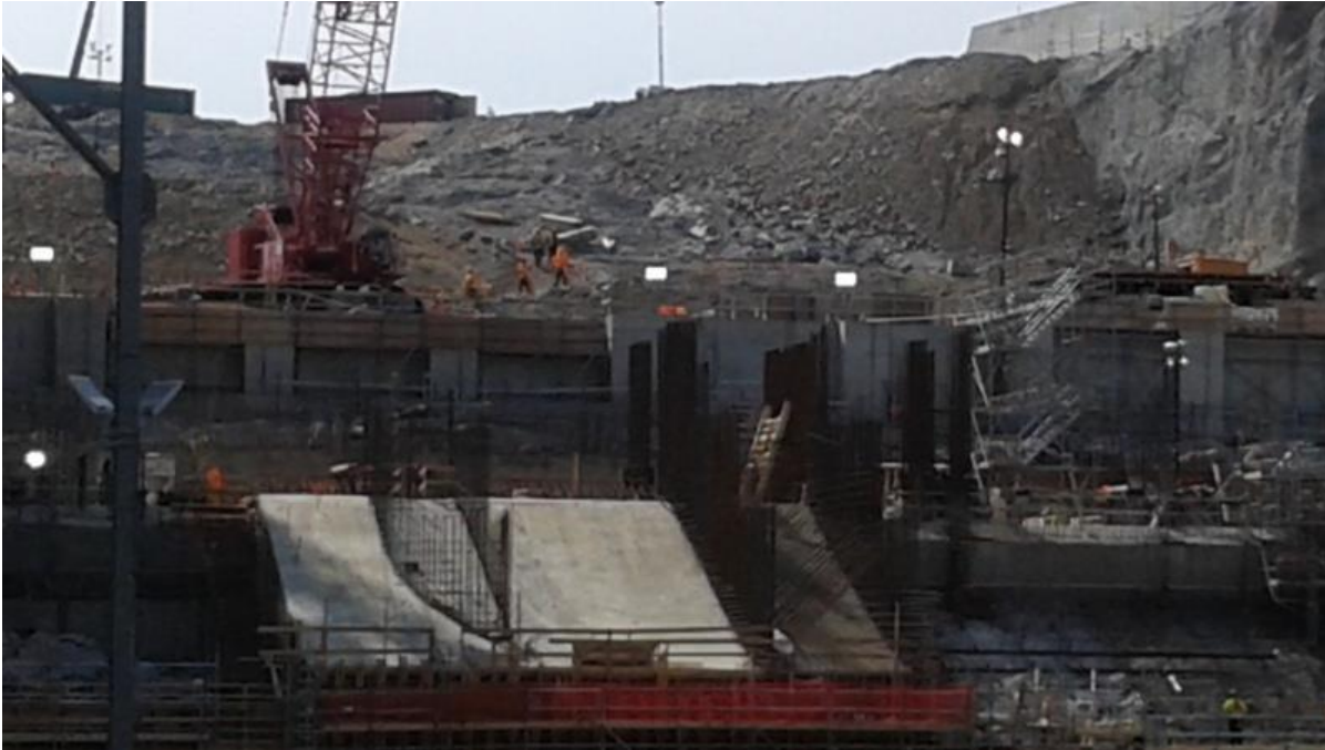
Photo 7.1 Unit 3 – Intake invert slab completed with central pier reinforcement dowels in place (July 7, 2015).
