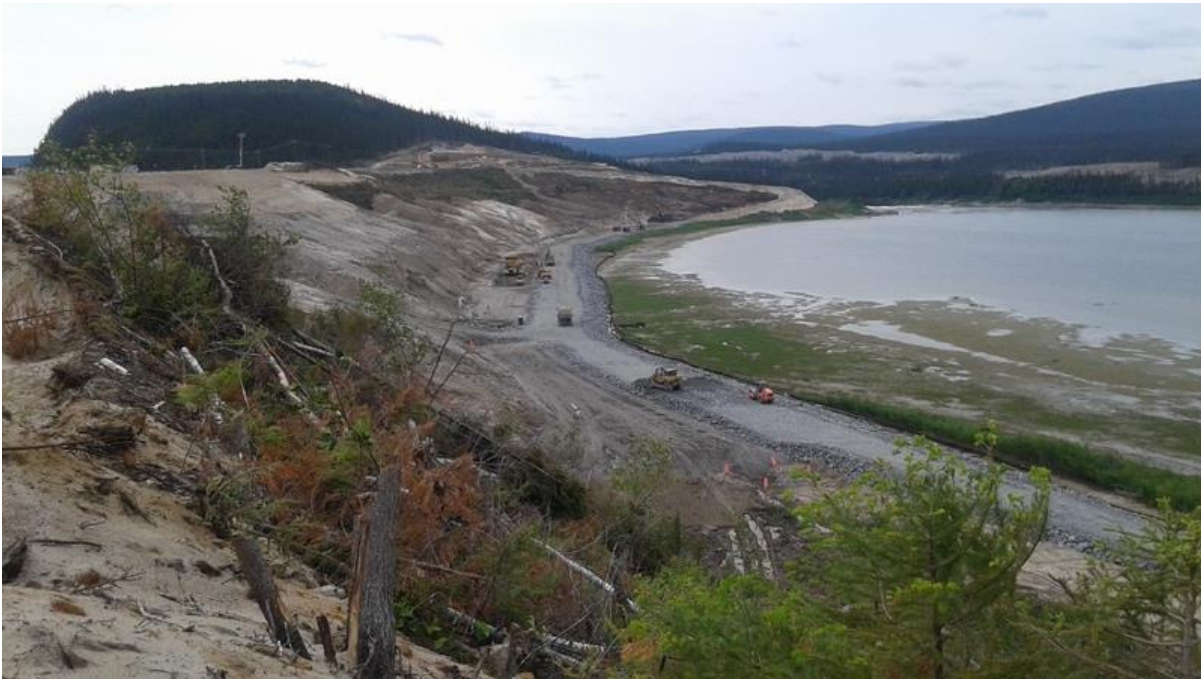
Photo 1.1 Looking at Upstream Slope of North Spur. Clearing and OM excavation completed. Contractor working on preparation of CB Work platform ( July 7, 2015 )
