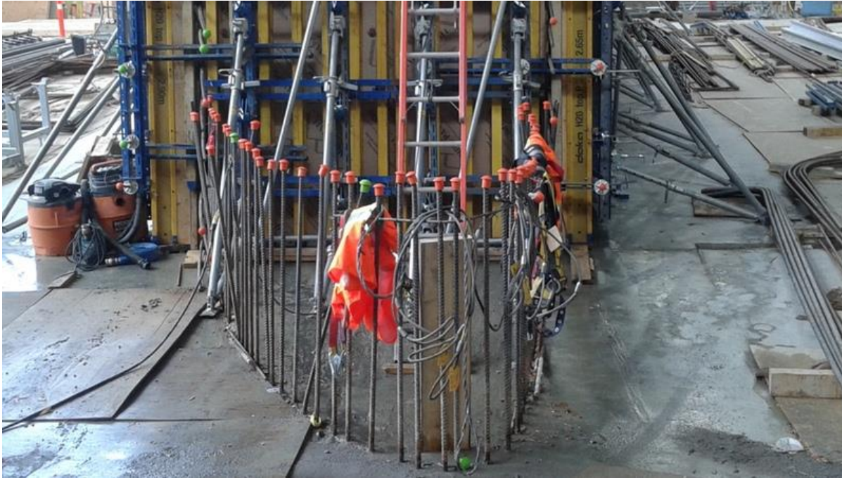
Photo 7.3 Unit 1 – Invert slab of draft tube completed. Upstream end of draft tube central pier ready for formwork and reinforcement erection (July 7, 2015).
