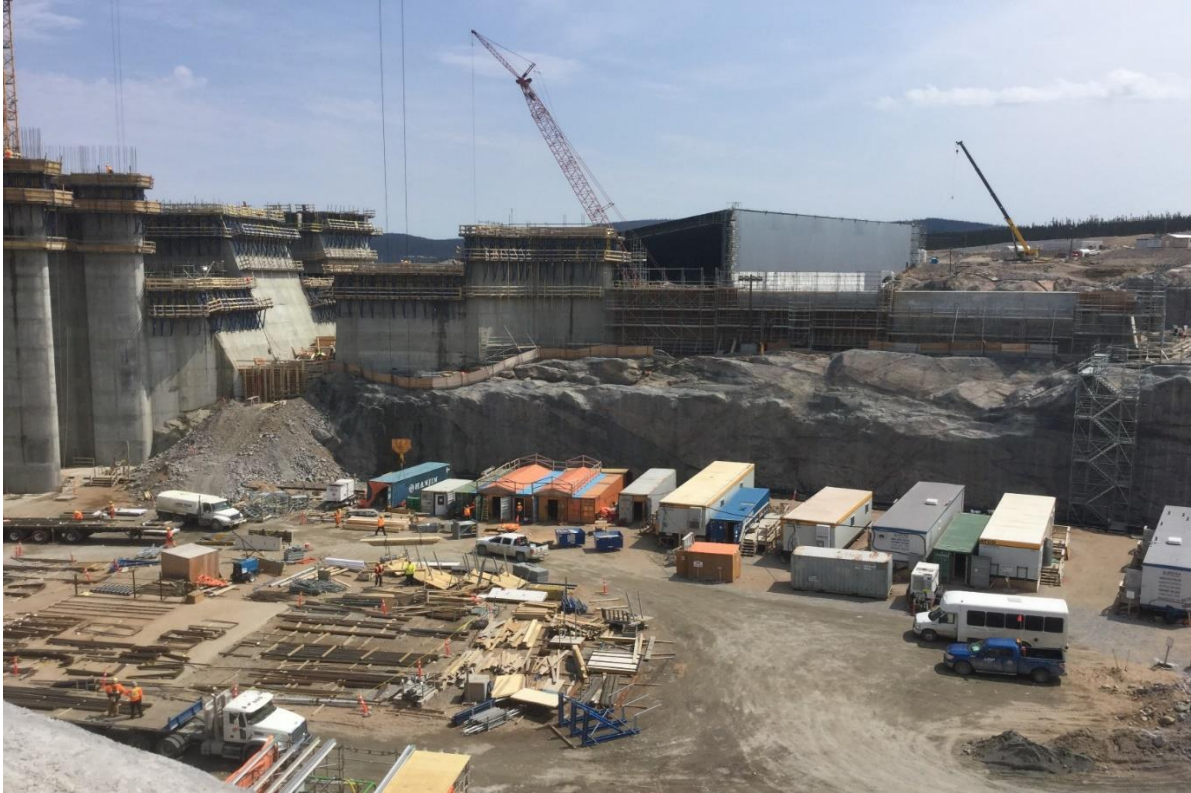
Photo 2: Looking (from top of RCC Cofferd Dam) along proposed centerline of Temporary Access Bridge to South Dam. (July 7, 2015)
