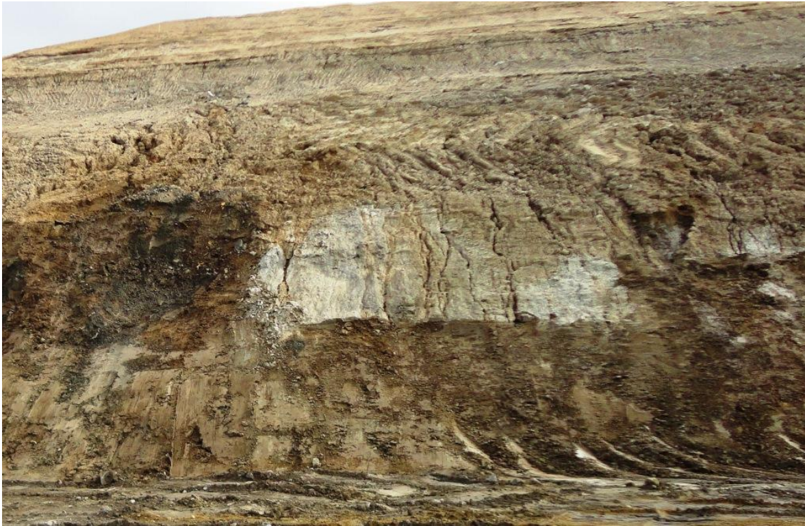
Photo 3.13: Upstream slope- Excavated slope in the upper clay and sand. Note the erosion runnels in the sand/silt at mid height.
