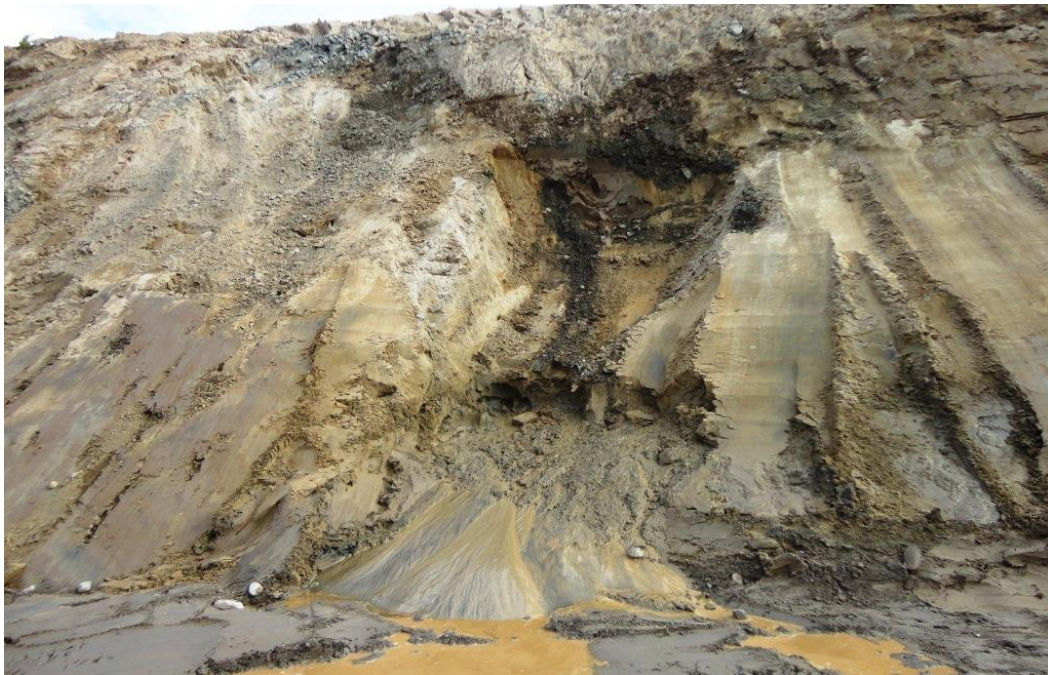
Photo 3.14: Upstream slope, layered Upper Clay/Sand zone. Note the water seepage from sand layers at lower and upper slope levels. This has caused localized washout of materials.
