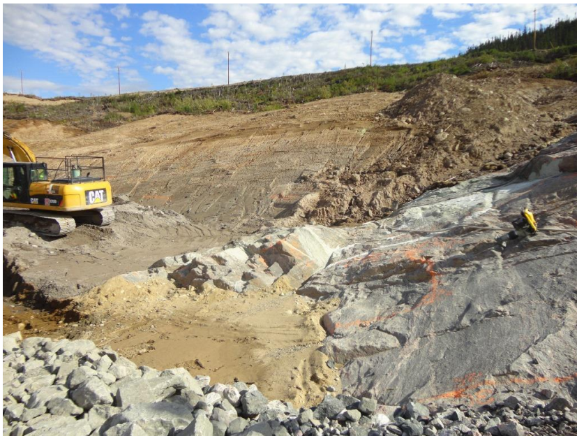
Photo 3.12: Upstream slope. Placement of fine grained till and granular transition on the bedrock outcrop at the south end of the upstream slope.
