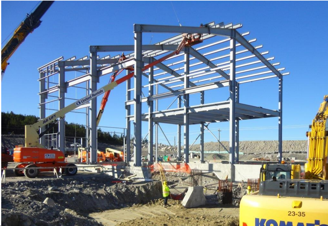
Photo 2.5: Synchronous condenser building
