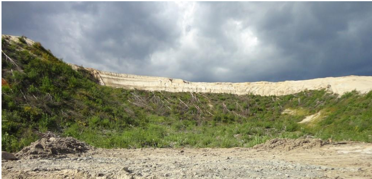
Photo 3.19: Downstream slope. View of the scarp of the 1978 landslide.
