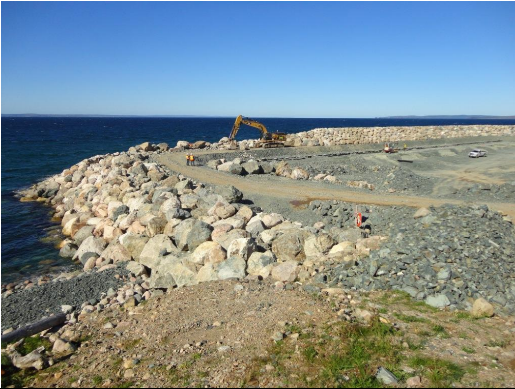
Photo 1.3: West end of the Dowden's Point dyke. Note the ongoing armour stone placement work.
