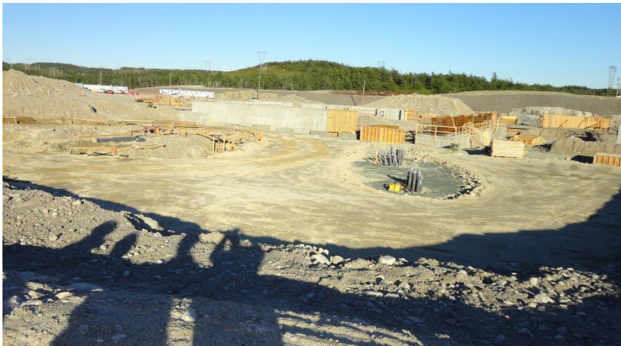
Photo 2.10: DC transformer foundation southern area
