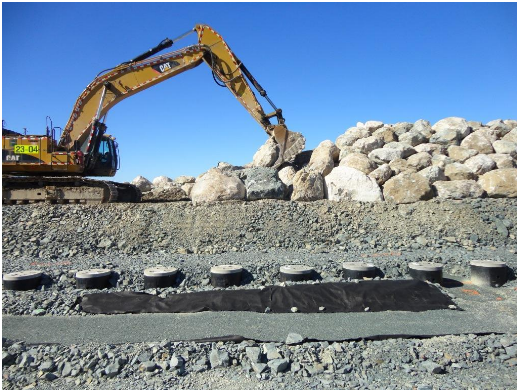
Photo 1.6: Placing and dressing the armour stone at the west end of the dyke. Electrode wells visible in foreground.
