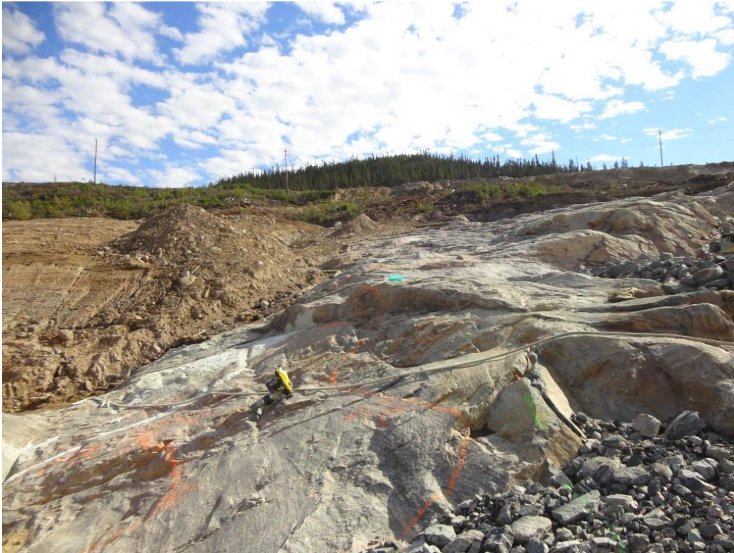
Photo 3.11: Upstream slope. Granitic bedrock exposed at the periphery of the rock knoll at the south end of the upstream slope.
