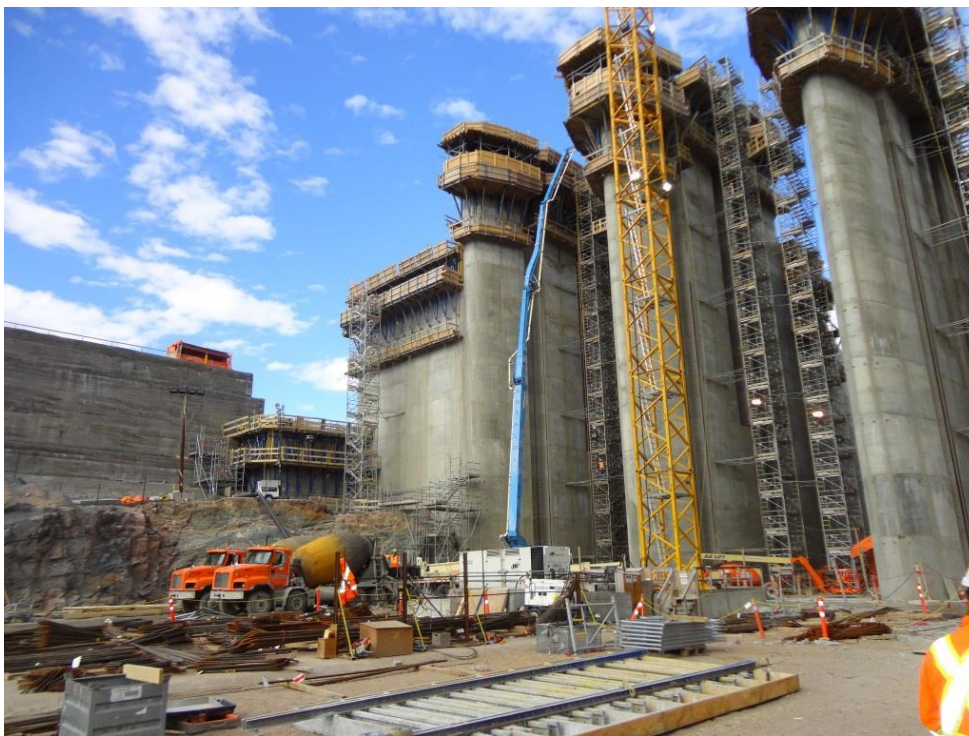
Photo 4.6: Spillway, right upstream corner. The RCC cofferdam and partially completed concrete transition dam are visible.
