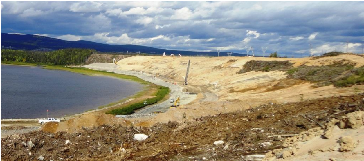
Photo 3.1: Upstream slope - Overall view of the upstream slope of the North Spur, showing the excavated slope and the cut-off wall line along el 20m the toe berm. View is looking towards the north. The working platform at el 20m is visible along the toe of the excavated and trimmed slope. In the back ground, the el 24m and el 28m fill intermediate placement berms can be seen.
