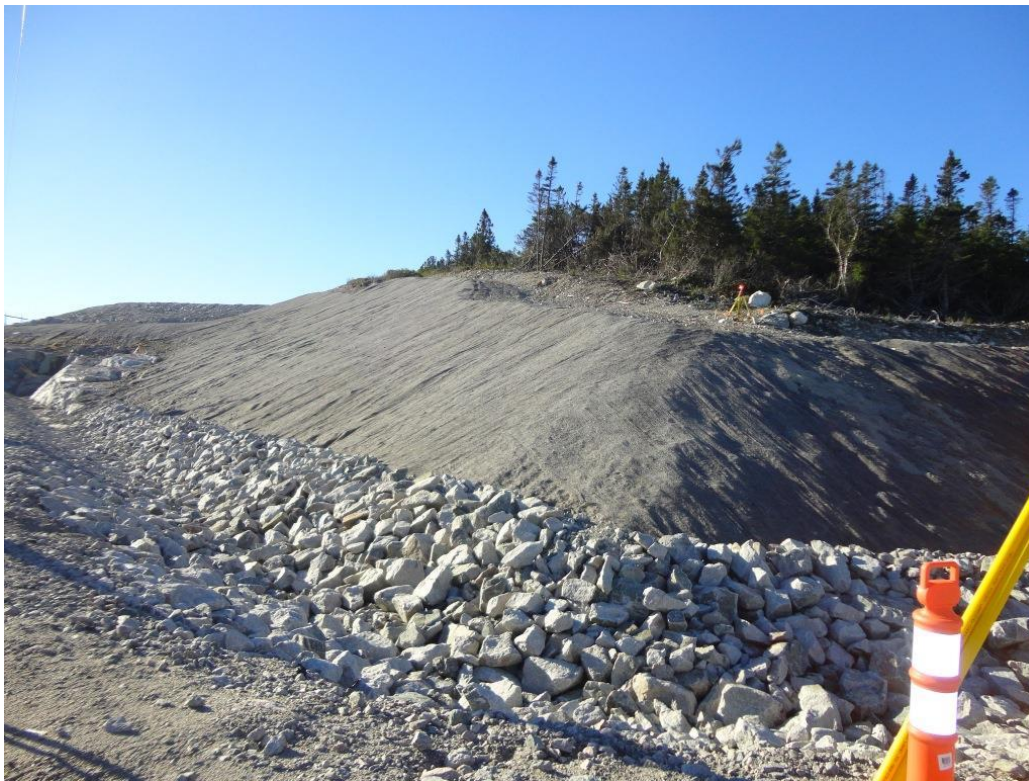
Photo 2.2: Cut slope in glacial moraine at west end of the facility. The upper slope is covered by porous coconut/wire mesh slope protection. No seeding has been done and this mat has deteriorated in many places. Rip rap layer in place on the lower slope.
