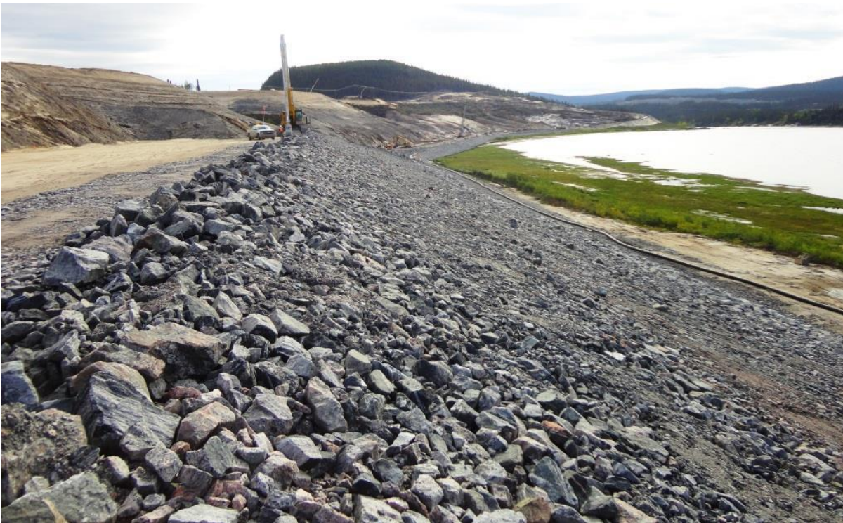
Photo 3.6: Upstream slope - Upstream rockfill as viewed looking south from the el 24m level.
