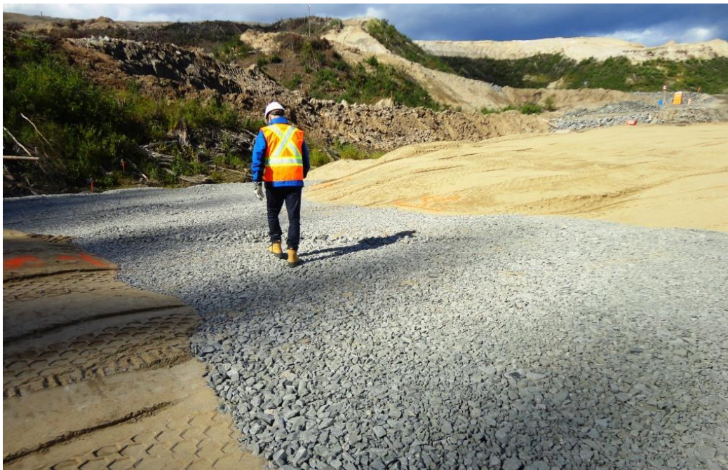
Photo 3.22: Downstream slope; finger drain near the toe of the slope. The finger drain filters extend across the slope.
