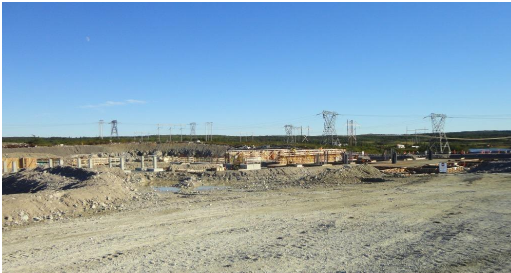
Photo 2.1: AC/DC converter site
