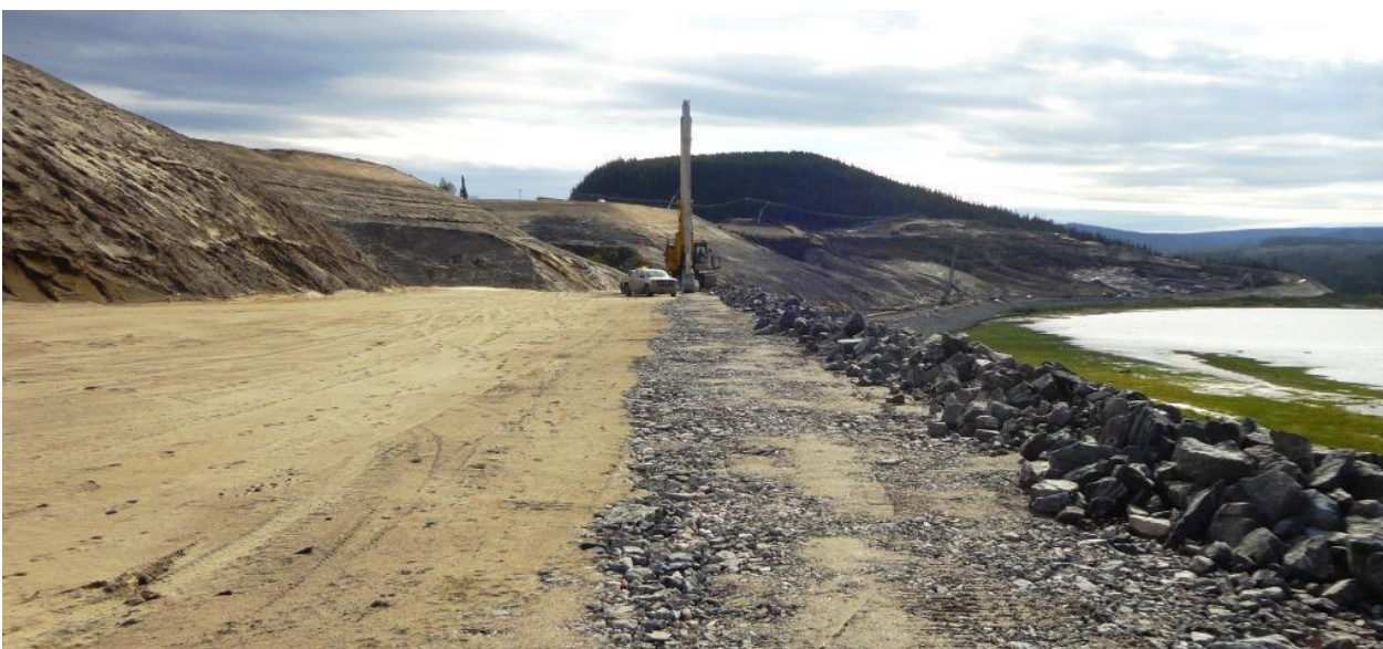
Photo 3.4: Upstream slope. El 28m berm at the north end of the cutoff. View shows, from right to left, the zoning of the rip rap, transition zones, and sandy fill.
