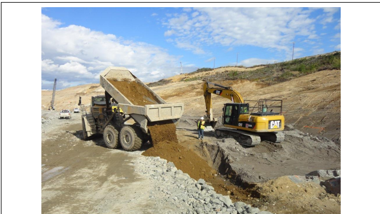
Photo 3.10: Upstream slope. Placing granular transition for the impervious blanket at the south end of the upstream slope.
