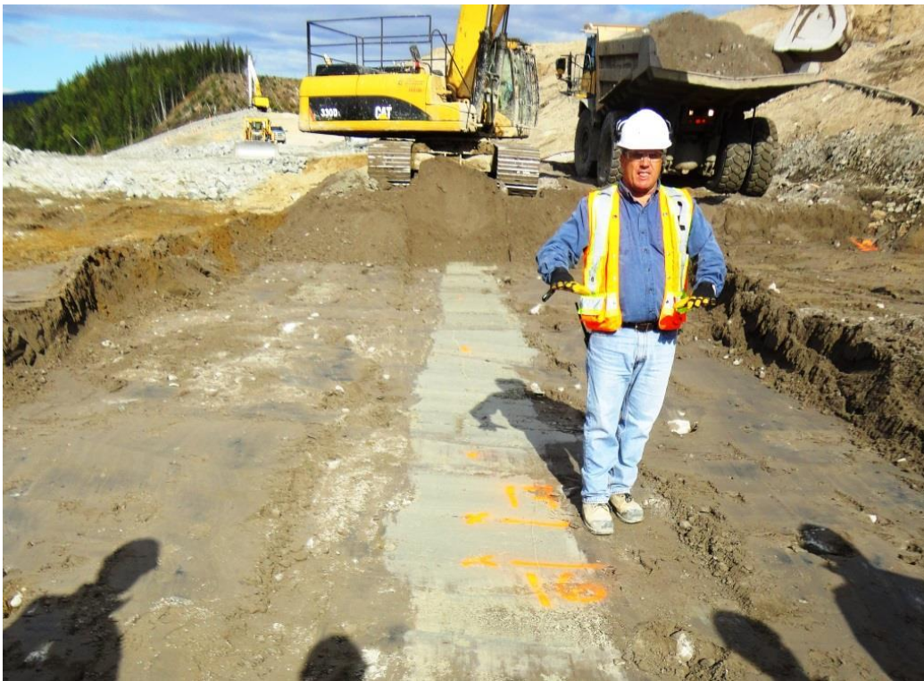
Photo 3.8: Upstream slope. Top of the cement/bentonite cut-off wall at el 20m. Note ongoing placement of the till blanket covering the wall in the background of the photograph.
