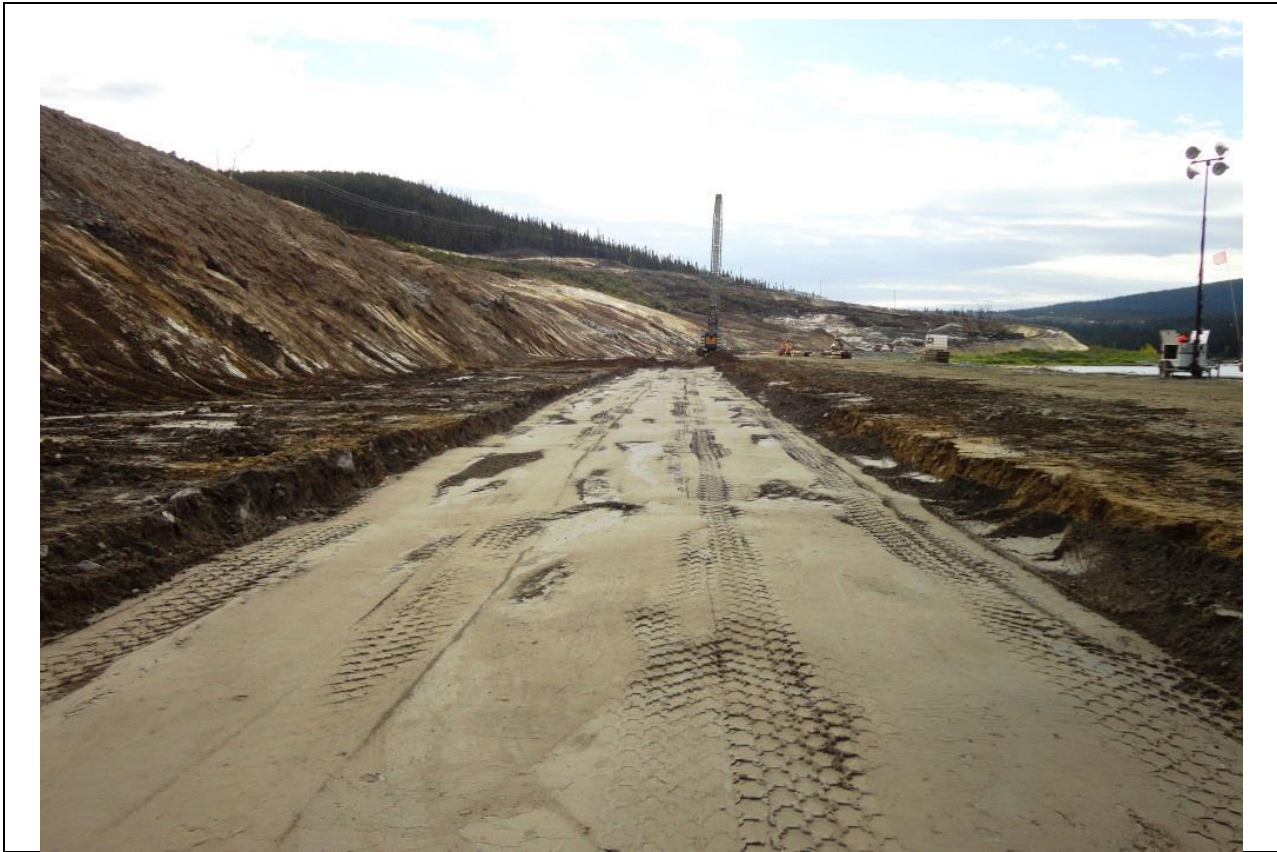
Photo 3.9: Upstream slope - Compacted fine grained till placed over the top of the cut-off wall at el 20m.
