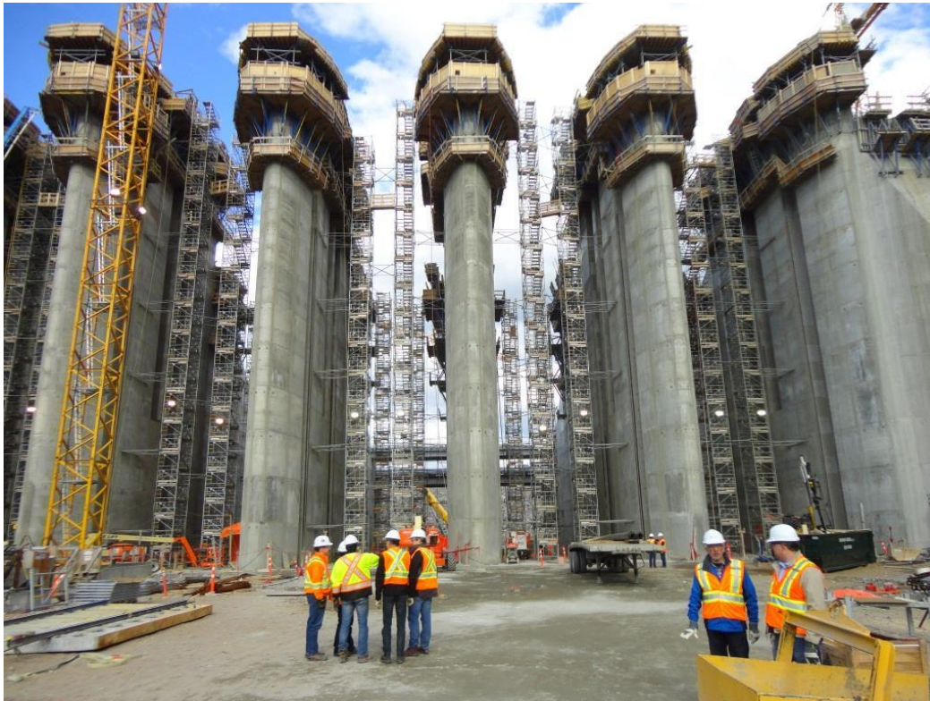
Photo 4.4: Spillway looking towards downstream. From right to left, Bays 1, 2, 3, and 4 are visible.
