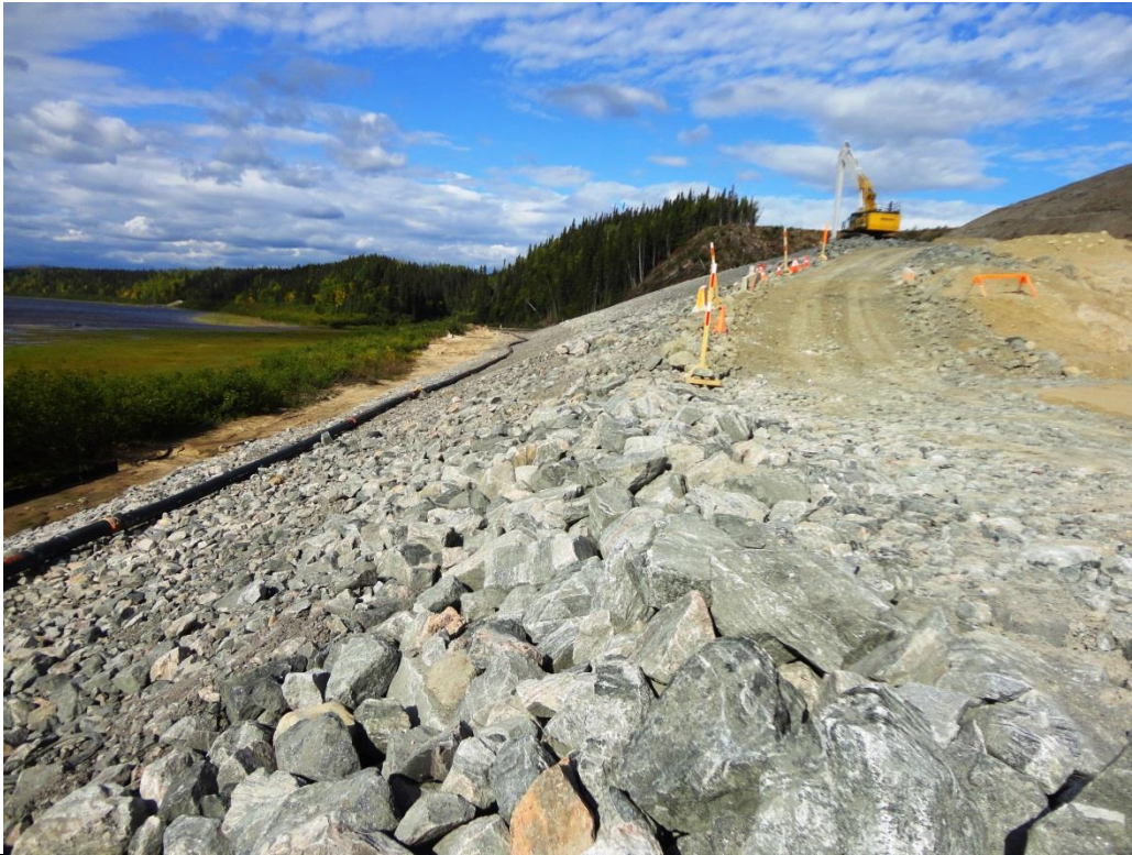
Photo 3.5: Upstream slope. Upstream rip rap blanket as viewed looking north from the el 24m level.
