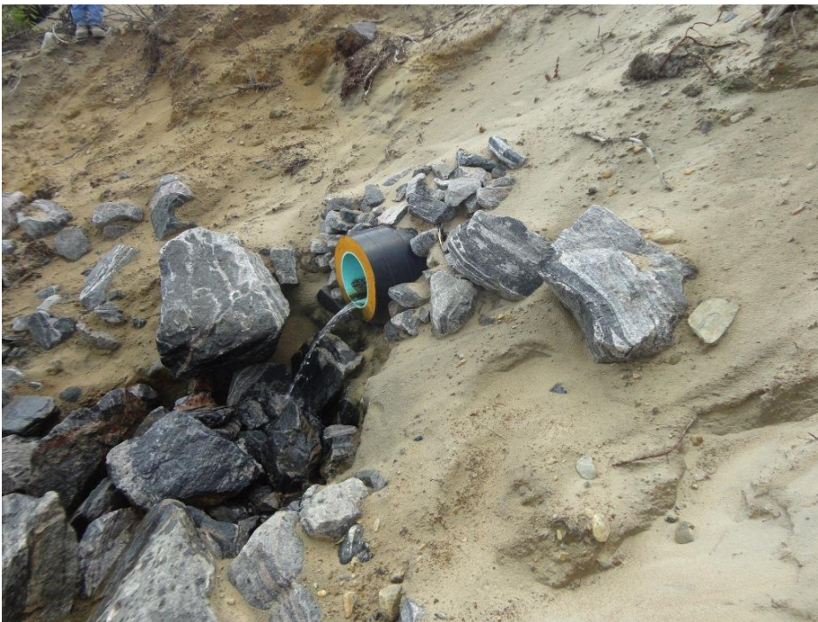
Photo 3.26: Pumped wells outlet pipe in the ravine downstream of the kettle lakes.
