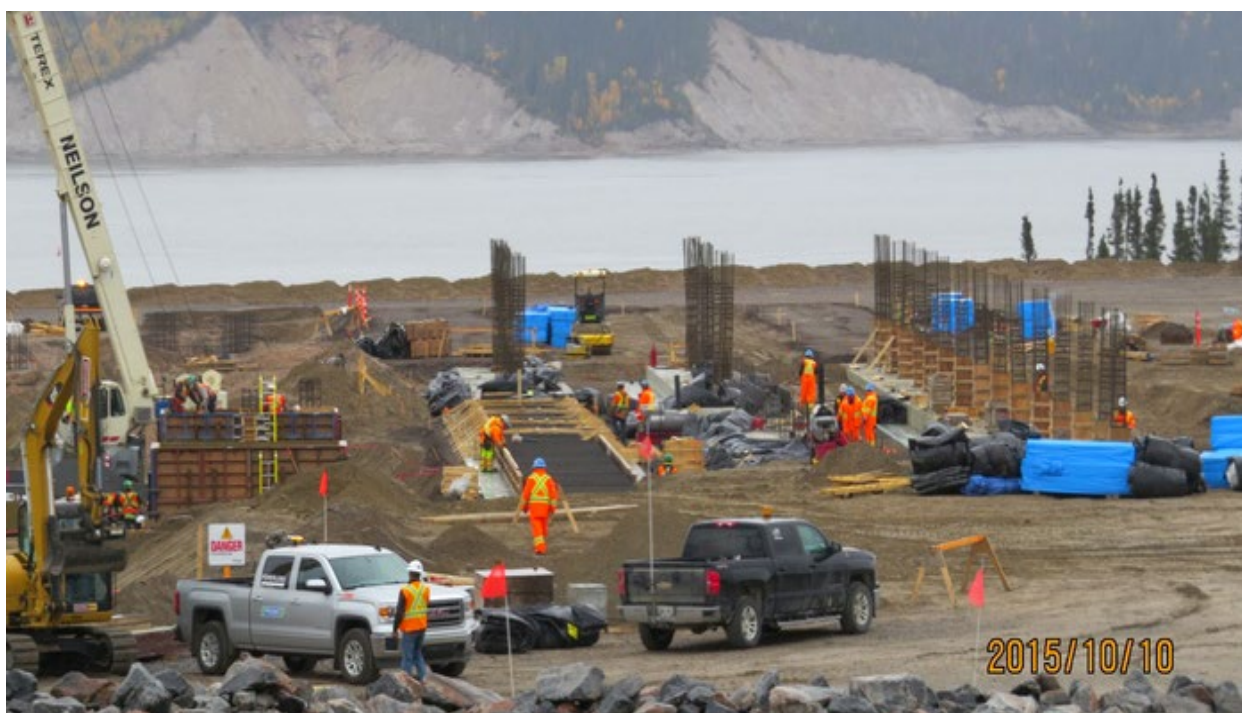
Muskrat Falls Switchyard – October 2015
