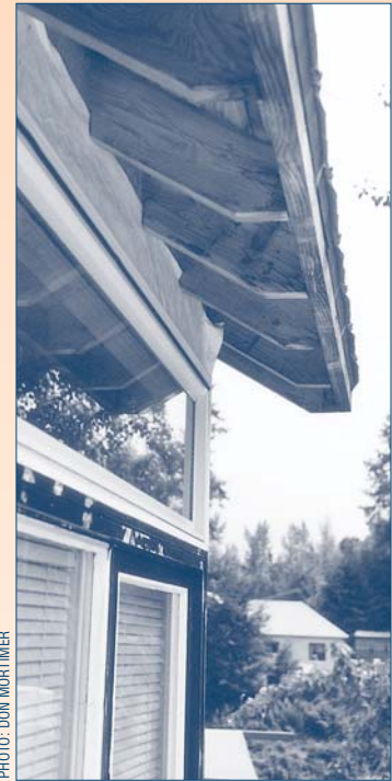
▲ Open eaves, vents not screened. (6 pts)
