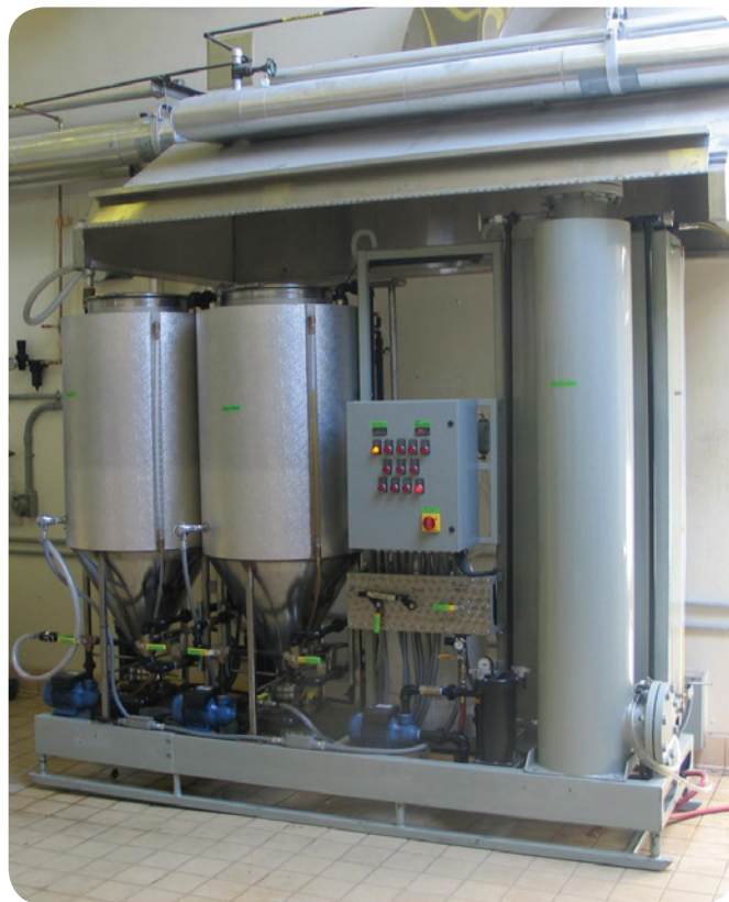
MI Biodiesel Project
