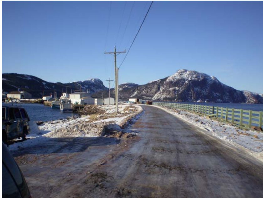
Photo 4.2.2.3 – Existing wharf access road showing harbour to the left and retaining wall/spraywall to the right
