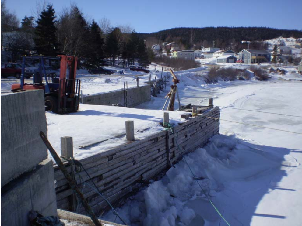
Photo 4.7.4.1 – Photo showing possible new outflow wharf location looking from Nordic Salmon’s existing wharf
