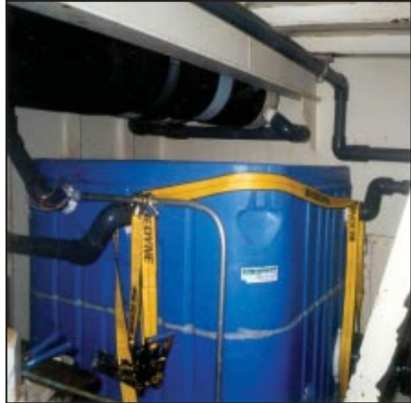
The reservoir tank holds fresh seawater.
